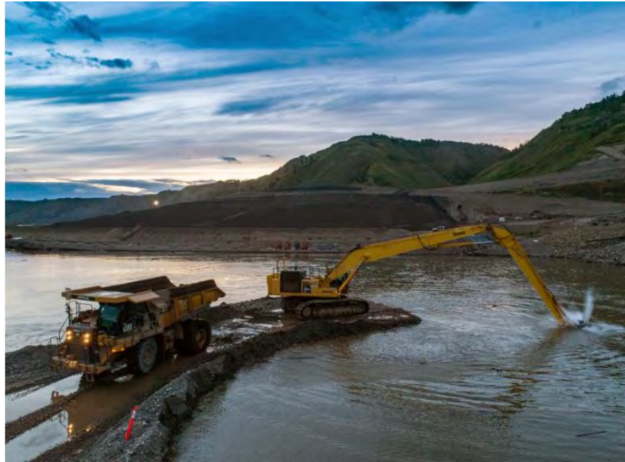
Figure A-27 A specialized excavator dredges and deepens the approach channel to the diversion tunnels (August 2020)
