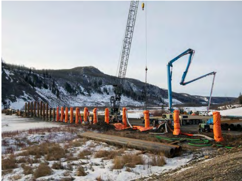
Figure A-9 Moberly River piles are cut to final elevation, filled with concrete and tarped to maintain adequate temperature during the curing process (February 2020)
