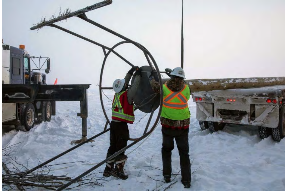
Figure A-43 Workers attach a bald eagle nest structure to an 18-metre-long pole. (November 2020)
