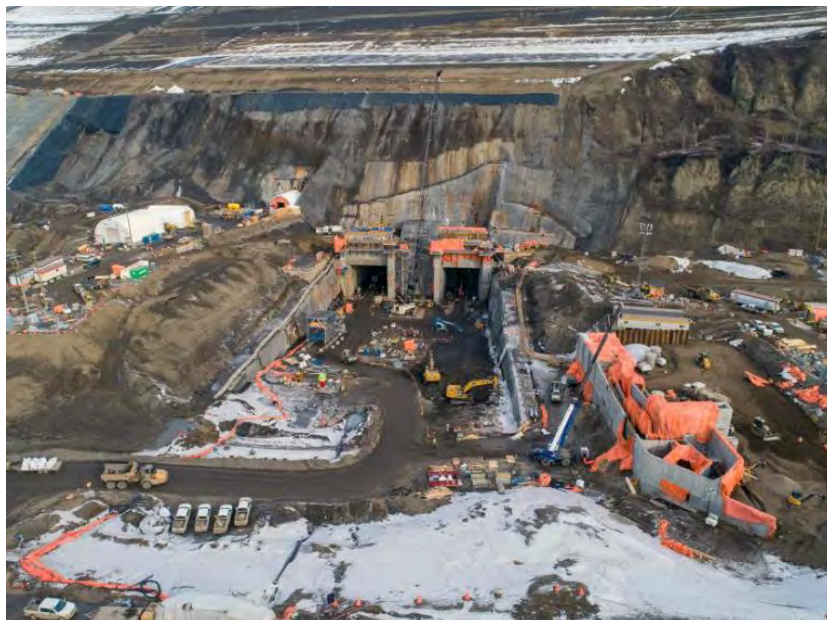
Figure A-6 Aerial view of the diversion tunnel outlet portals and the temporary fish passage facility under construction (February 2020)
