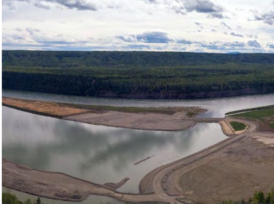
Figure A-31 The completed toe berm of the Lynx Creek East Highway 29 segment (August 2020)
