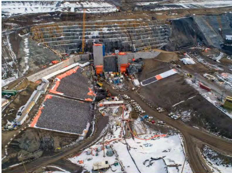
Figure A-5 Aerial view of the diversion tunnel inlet portals. The tower structures house the mechanical gates required to control water flows into the tunnels (February 2020)
