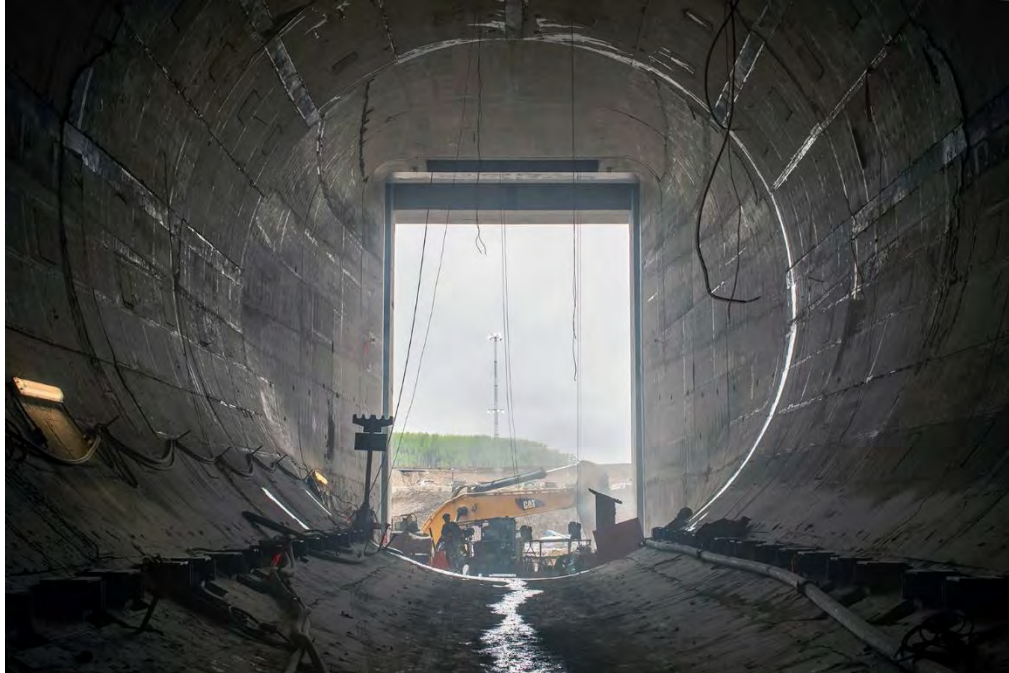
Figure A-15 A view from inside one of the two recently completed diversion tunnels (May 2020)
