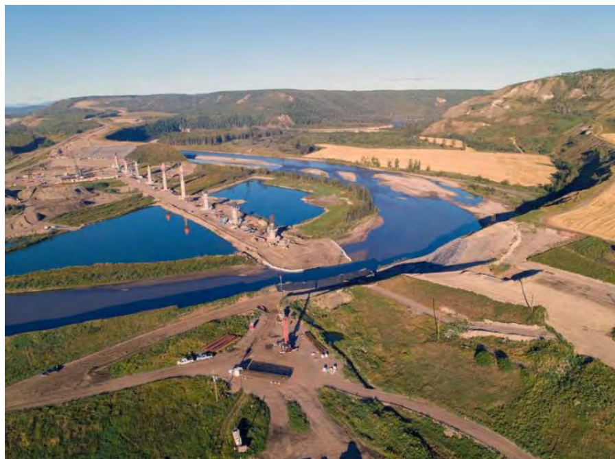
Figure A-36 The new Halfway River Bridge, with nine of 12 piers under construction (September 2020)
