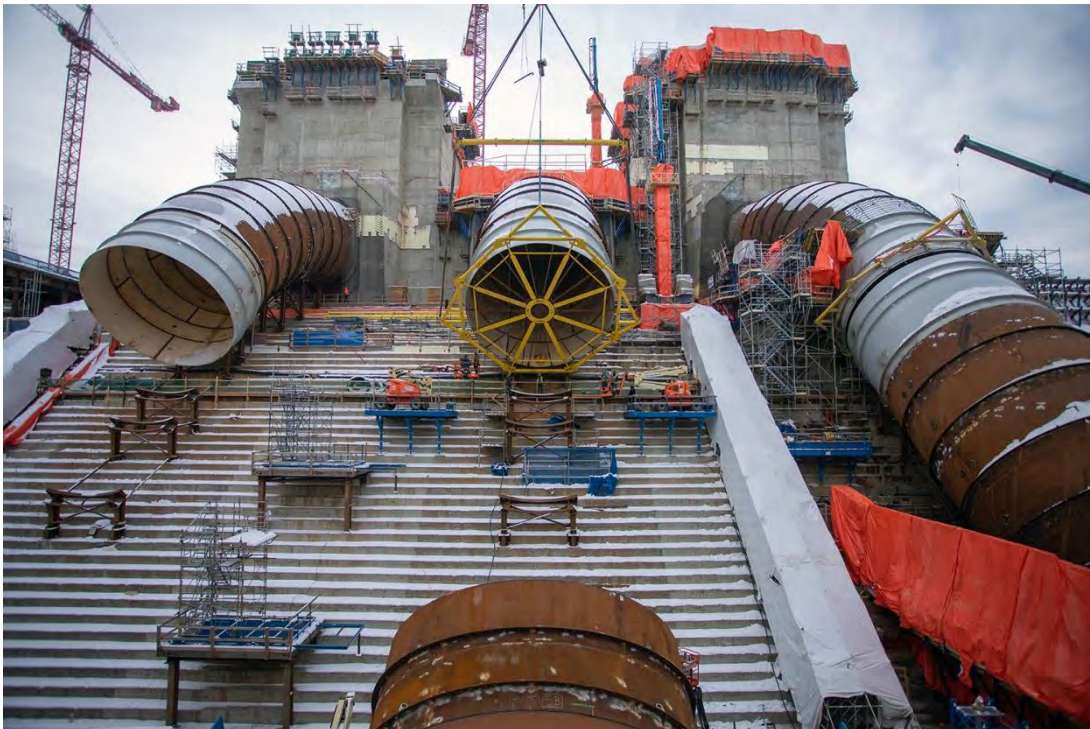
Figure A-44 A penstock piece is lowered into place as part of the penstock installation for Unit 2 (November 2020)
