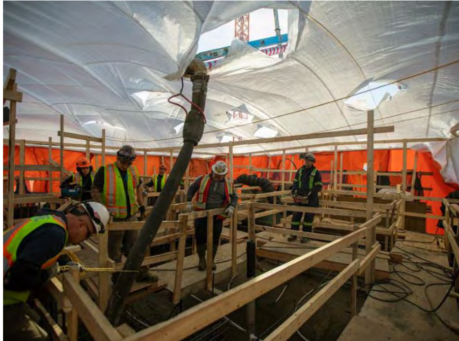
Figure A-1 A concrete placement takes place at the intake area of the powerhouse (January 2020)
