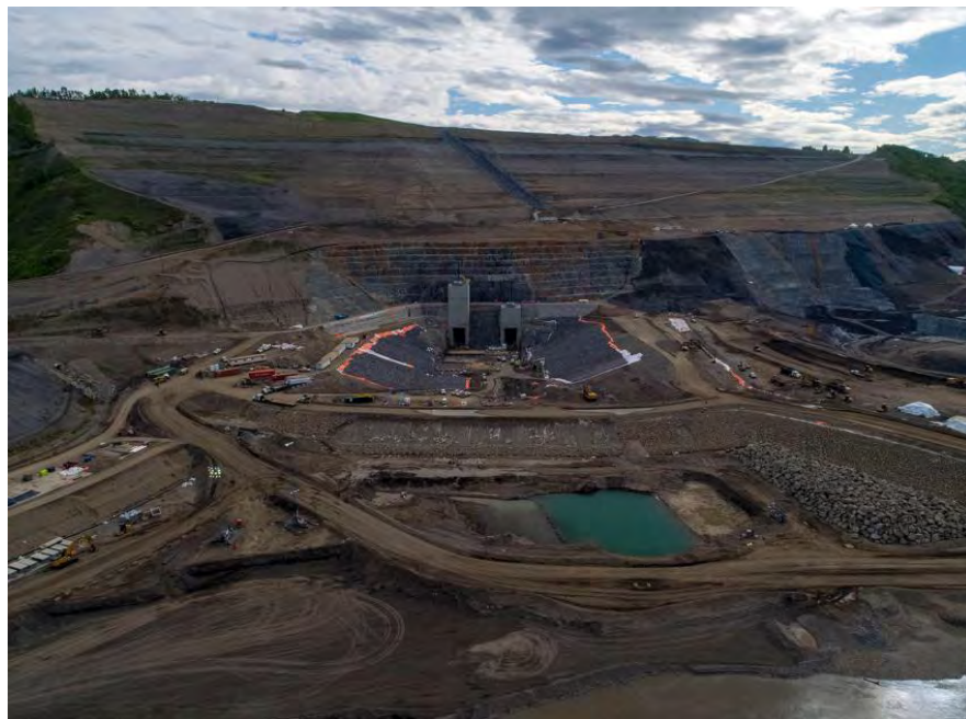
Figure A-16 North bank overview of the completed diversion tunnel inlets (May 2020)
