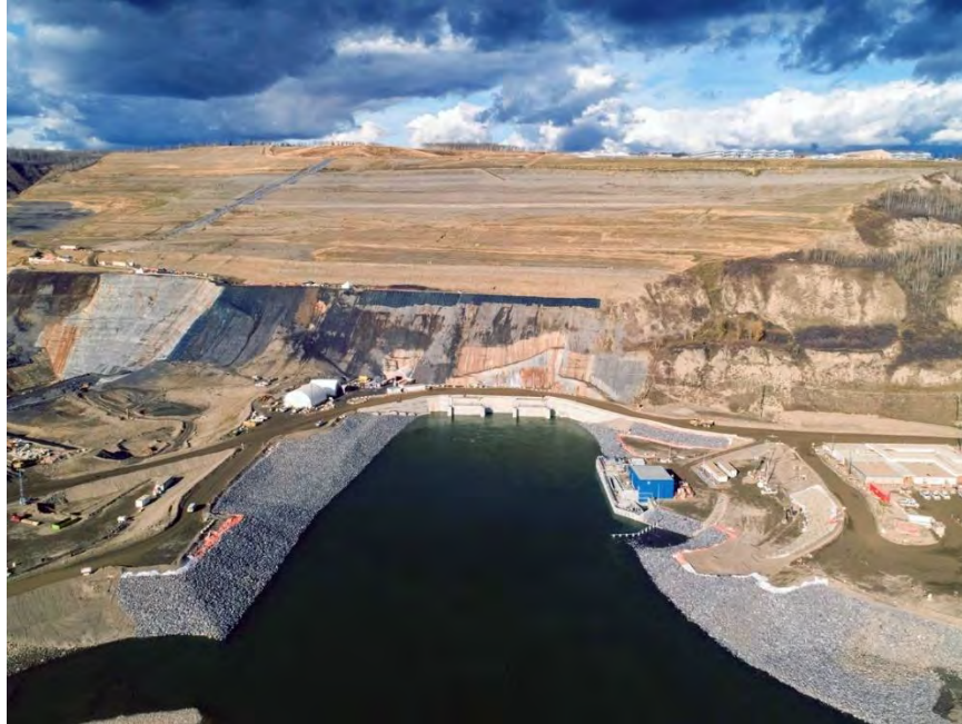
Figure A-41 The Peace River flows out of the diversion tunnels near the temporary fish passage facility (blue building) (October 2020)
