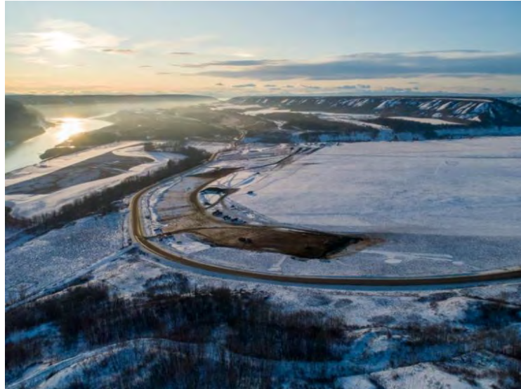
Figure A-11 Construction of Cache Creek East embankment, as part of Highway 29 realignment (March 2020)
