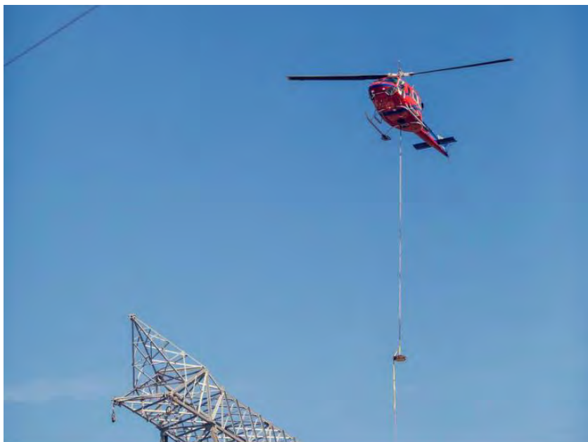
Figure A-33 The helicopter completes the sock line installation on a free standing 500 kilovolt transmission tower near the Peace Canyon switchyard (August 2020)
