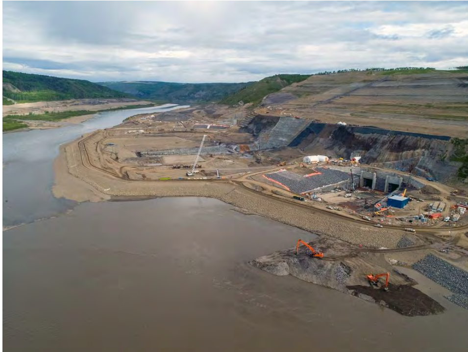
Figure A-21 In-river construction begins at the dam site, to prepare for river diversion in the fall (June 2020)
