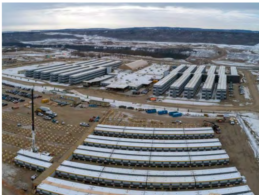
Figure A-12 An expansion of the Site C worker accommodation lodge is underway. These wooden cribs are installed to prepare for the 450-bed camp expansion. The existing lodge is in the background (March 2020)
