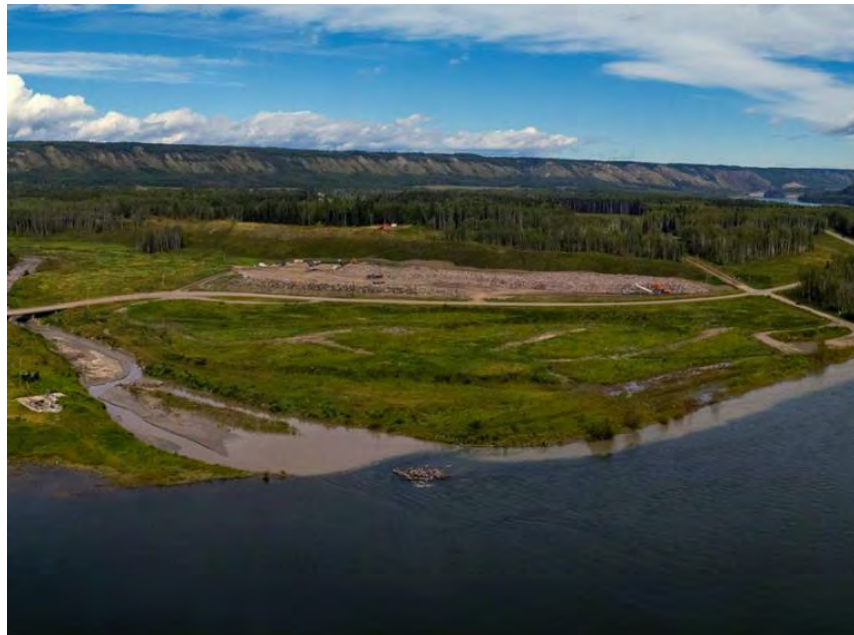
Figure A-30 Aggregate is stockpiled for the Highway 29 realignment at Lynx Creek West (August 2020)
