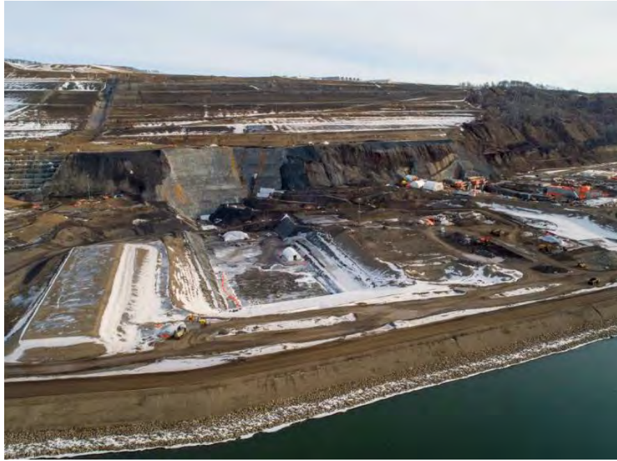
Figure A-7 Dam core trench excavation on the north bank is nearing completion (February 2020)
