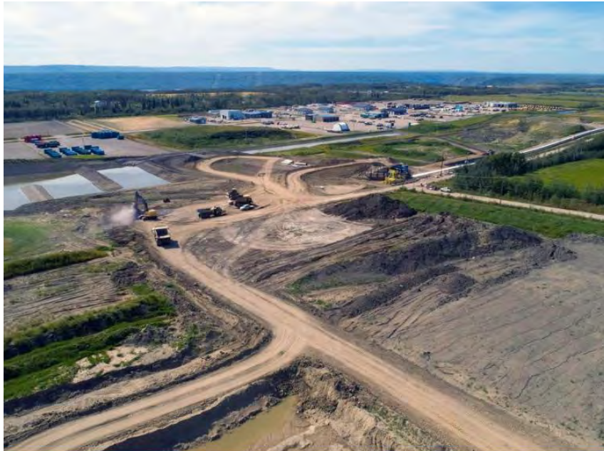
Figure A-29 Dam core materials from the 85th Avenue Industrial Lands are transported by a conveyor system to the dam site (August 2020)
