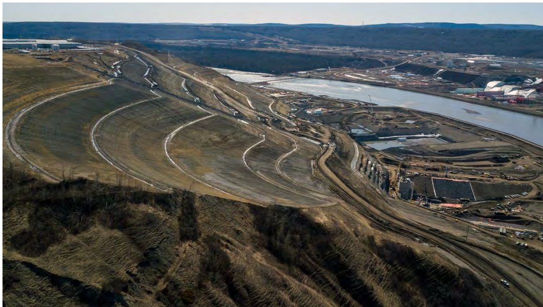
Figure A-14 This slope has been flattened to remove excess material to ensure stability and will be the future left bank of the earth fill dam (April 2020)
