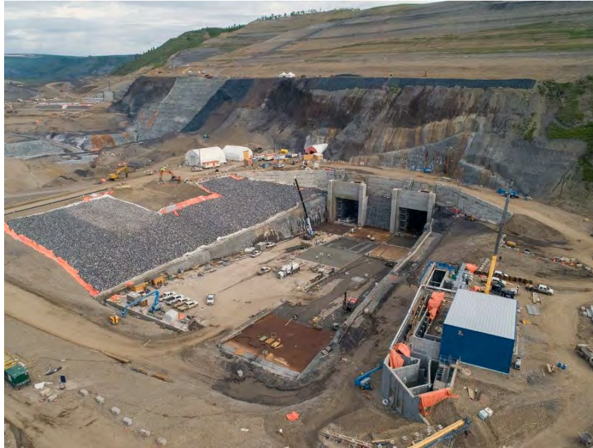
Figure A-17 The completed diversion tunnels outlet portal on the north bank and temporary fishway nearing completion (May 2020)
