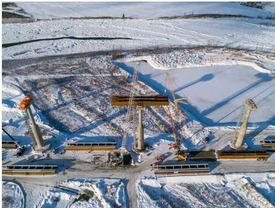
Figure A-42 The first steel girder was installed at the Halfway River Bridge on November 18, 2020 (November 2020)
