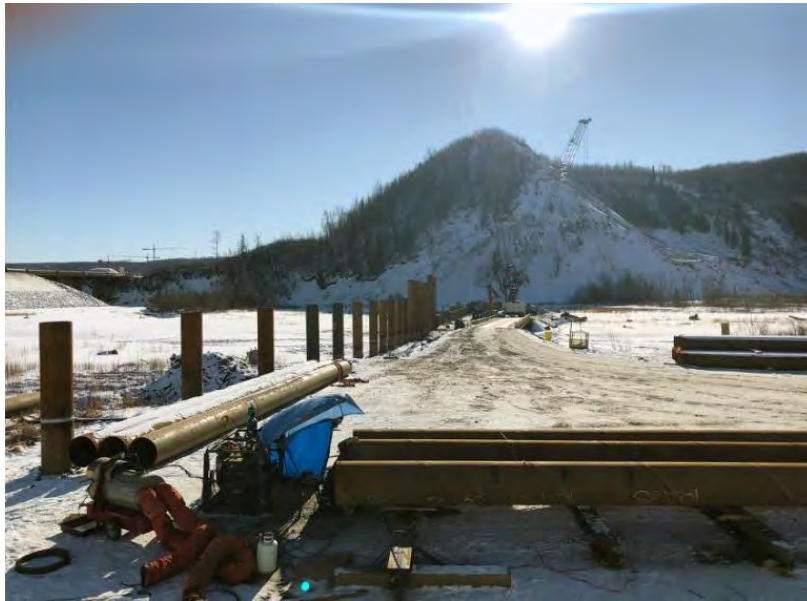
Figure A-3 Piles are being installed across the Moberly River to catch floating debris during river diversion. Debris booms will also be installed across the Moberly River, as well as the Peace River (February 2020)
