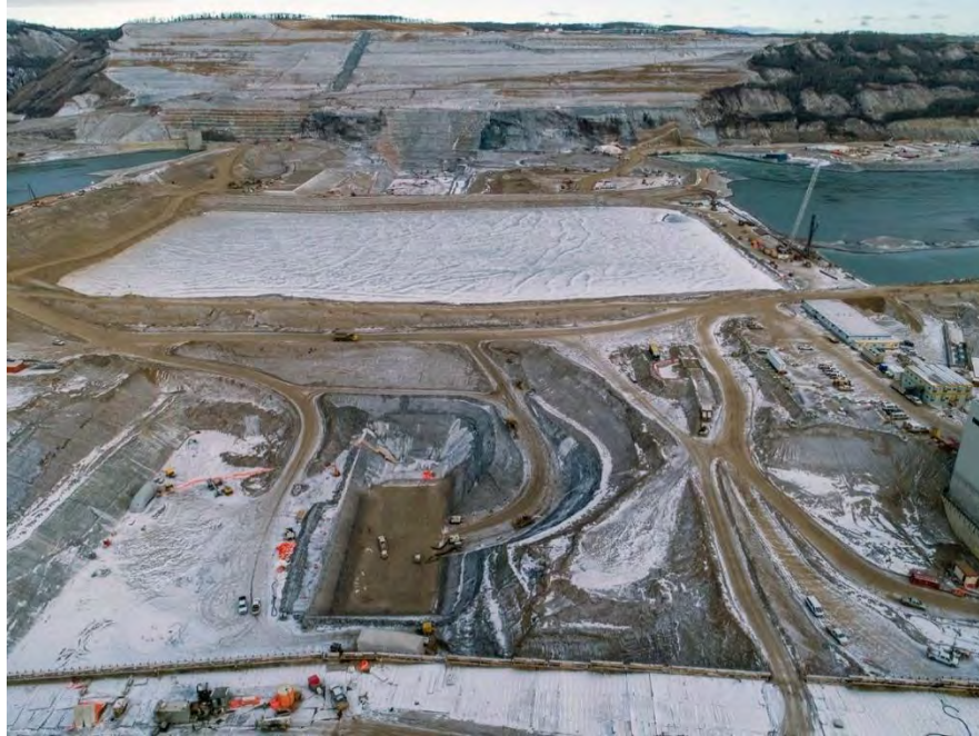
Figure A-47 An aerial view of the south bank dam core trench looking north across the diverted Peace River (December 2020)
