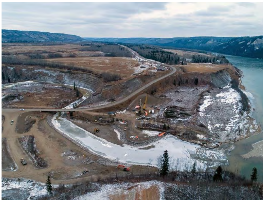
Figure A-46 An aerial view of the Highway 29 Farrell Creek alignment and work area where construction is continuing on the new highway and bridge (December 2020)
