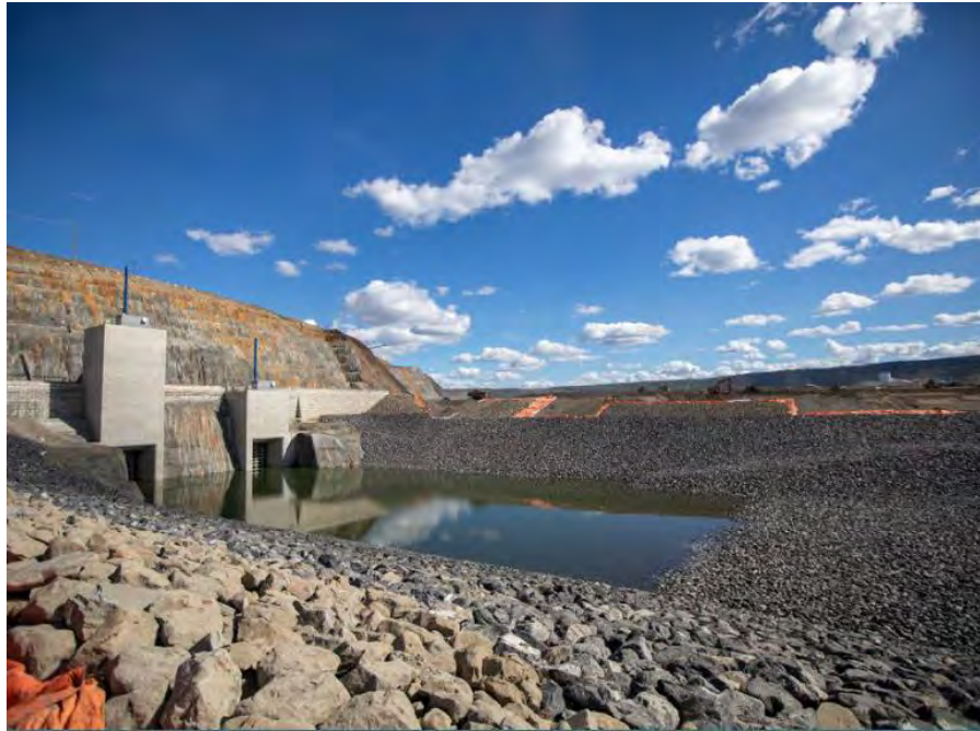
Figure A-35 Filling the inlet cofferdam in preparation for the diversion tunnel gates leakage testing (August 2020)
