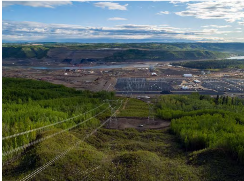
Figure A-19 View of the Site C substation down the transmission line right-of-way with the completed tower installations (May 2020)
