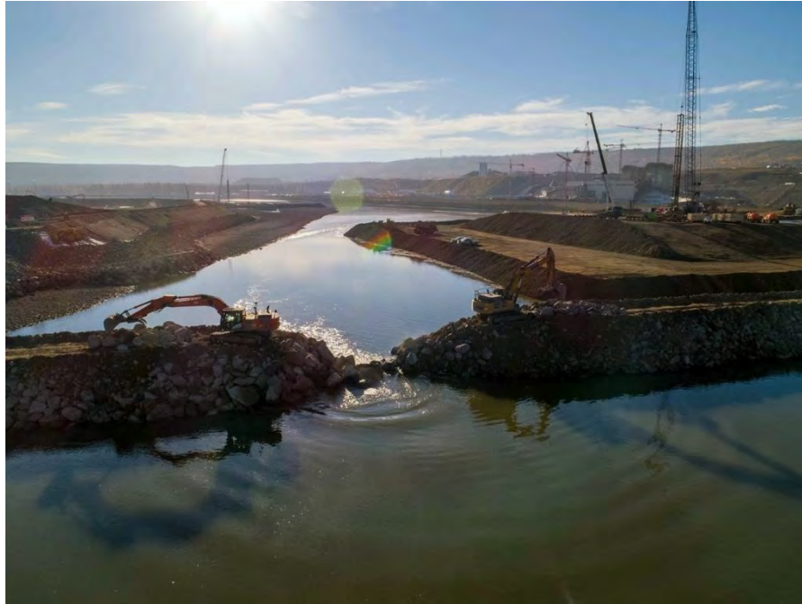
Figure A-39 On October 3, 2020, the final rock materials were placed to complete the rockfill berm, initiating full diversion of the Peace River (October 2020)
