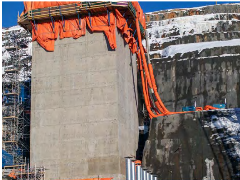
Figure A-4 The completed inlet structure for diversion tunnel No. 2 stands 30.5 metres, or nearly 10 stories high (February 2020)
