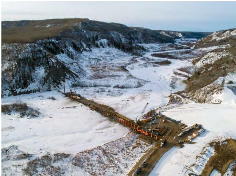
Figure A-10 An aerial view of the Moberly River pile structure under construction. This structure, in combination with a debris boom, will be used to capture debris floating in the river (February 2020)
