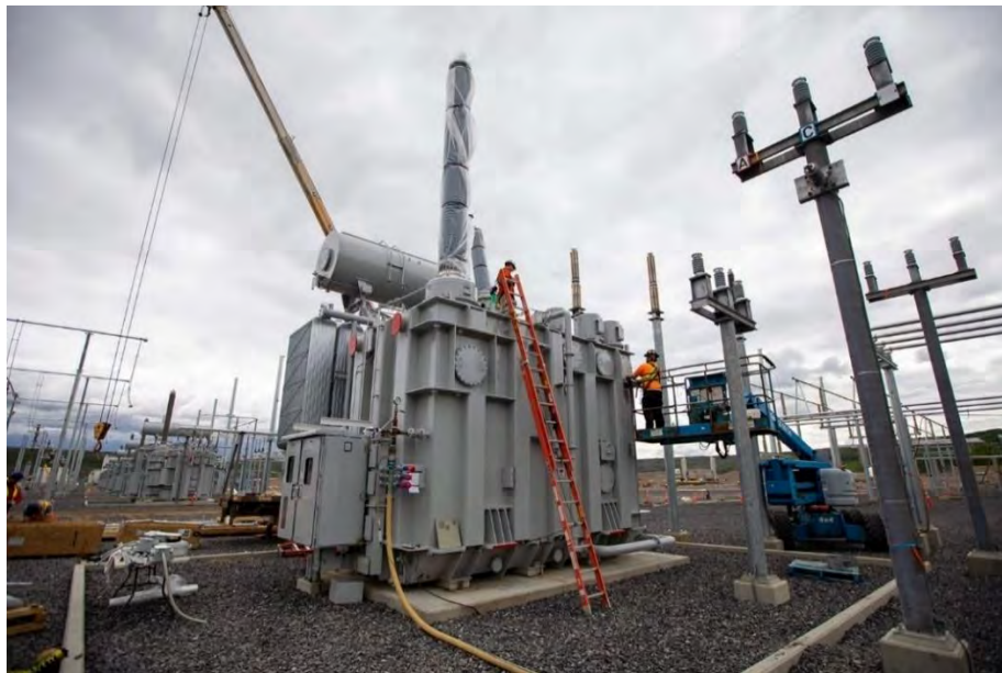
Figure A-24 Workers connect a transformer for the Peace Region Electrical Supply (PRES) system - located at the Site C substation (June 2020)
