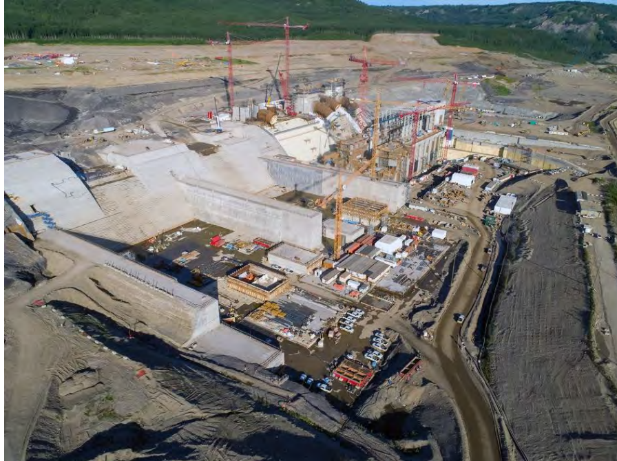
Figure A-23 View of the spillway headworks, stilling basin, intakes, penstocks and powerhouse (June 2020)
