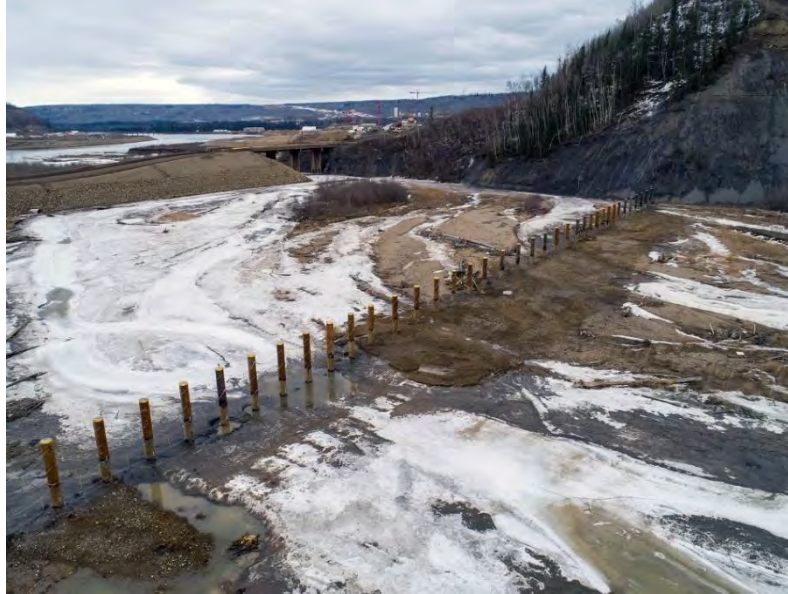
Figure A-13 The completed piles structure, located at the mouth of the Moberly River (April 2020)
