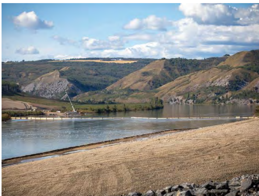
Figure A-34 Debris booms are in position upstream of the inlet portal to help manage woody debris in the Peace River (August 2020)
