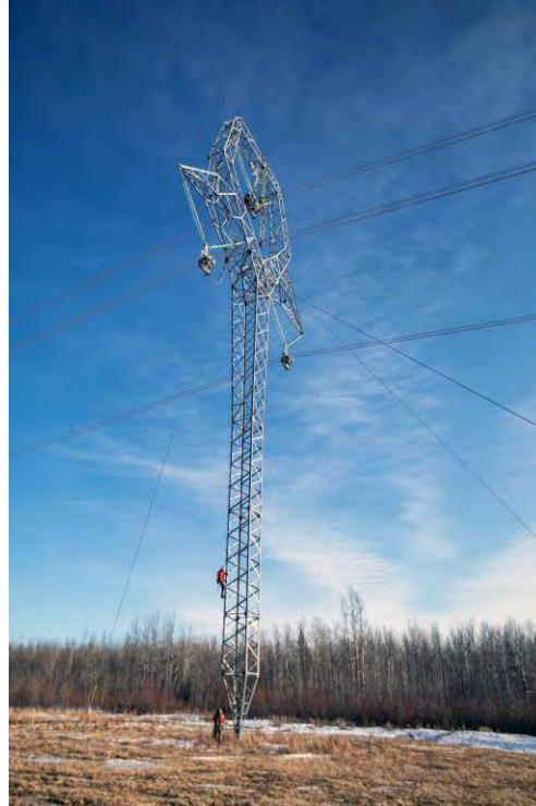
Figure A-5 Workers climbing a guyed tower to attach the conductors | February 2022
