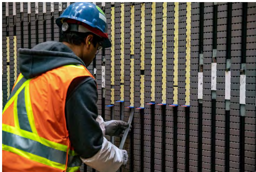
Figure A-24 Wedging the generator stator on unit 1 inside the powerhouse | November 2022
