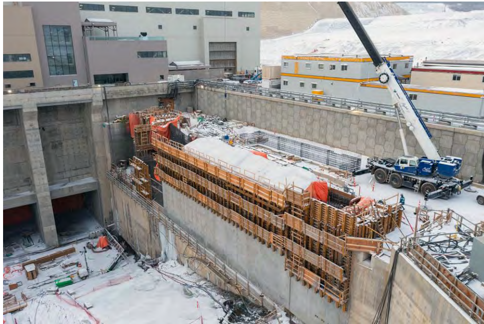
Figure A-27 Permanent upstream fish passage, which will help fish migrate upstream of the dam site | November 2022
