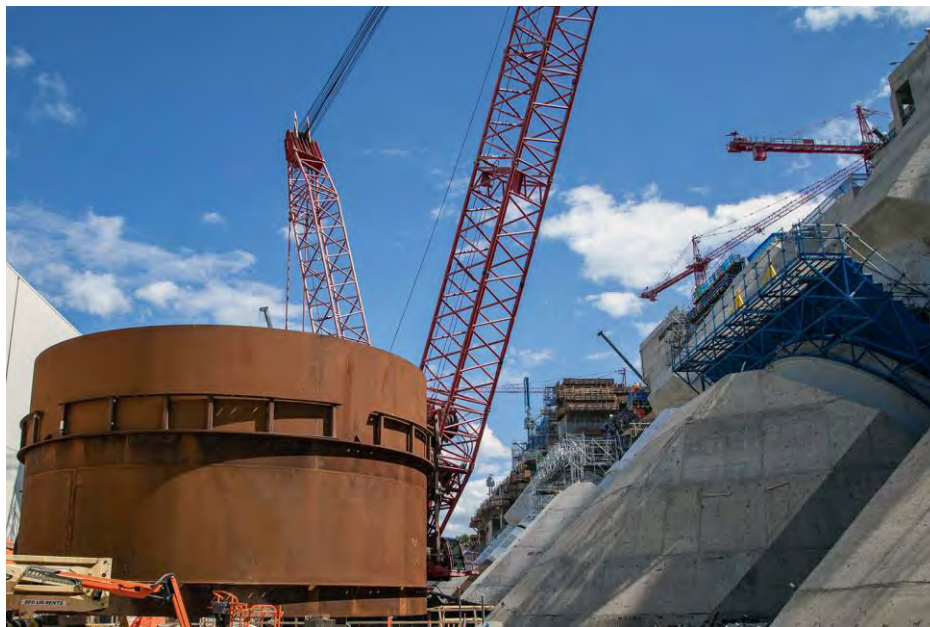
Figure A-8 The second to last penstock segment waits for installation on penstock unit 4 | June 2022
