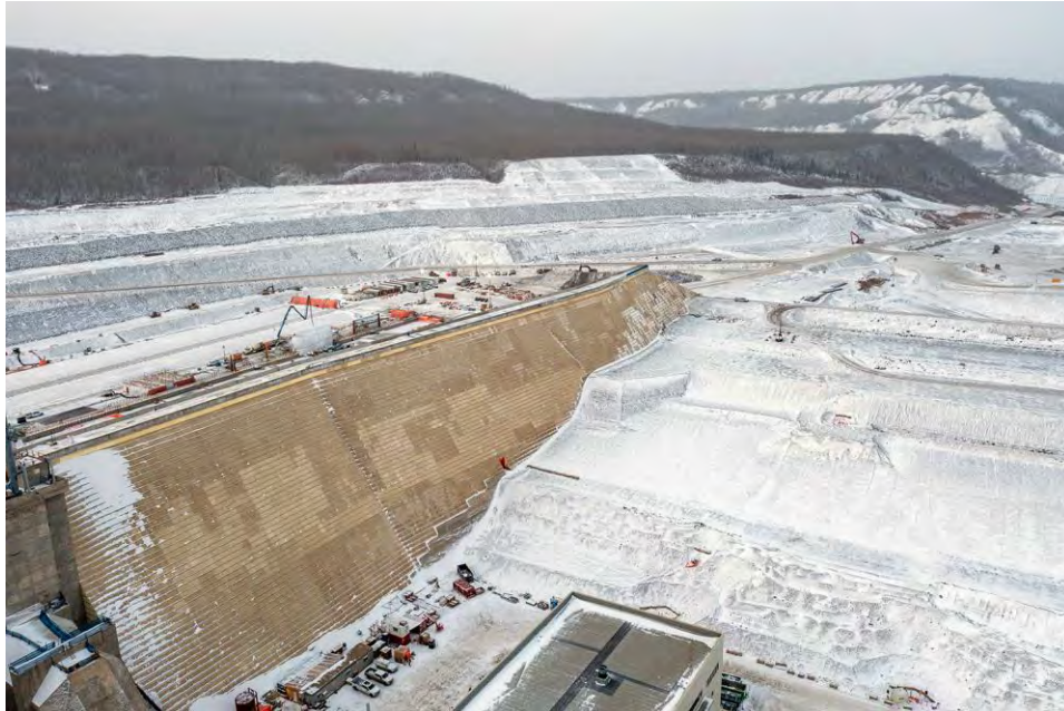
Figure A-29 The dam buttress, with the earthfill dam under construction, at a height of 445 metres above sea level | November 2022
