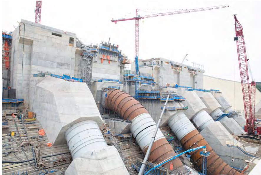
Figure A-11 The penstocks for units 1 (right side of picture) to 6 (left). Units 1-3 and unit 6 are encased in concrete; work is ongoing to complete units 4 & 5 | August 2022
