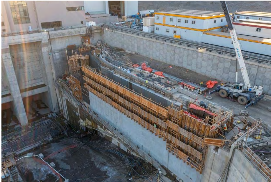
Figure A-19 Front-view of concrete placement and formwork installation at the permanent upstream fish passage facility | October 2022
