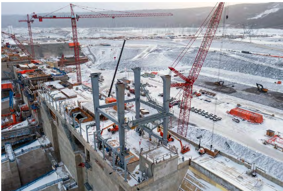
Figure A-28 A gantry crane on top of intake unit 1 | November 2022
