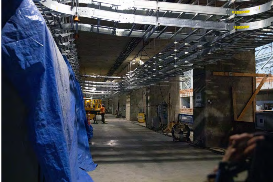
Figure A-13 A complete cable tray system on the generator floor level of the powerhouse | September 2022
