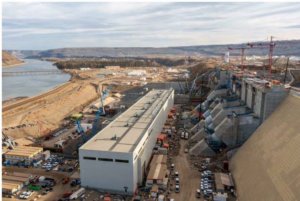
Figure A-18 East-facing view over the powerhouse and operations building and the future transformer yard | October 2022
