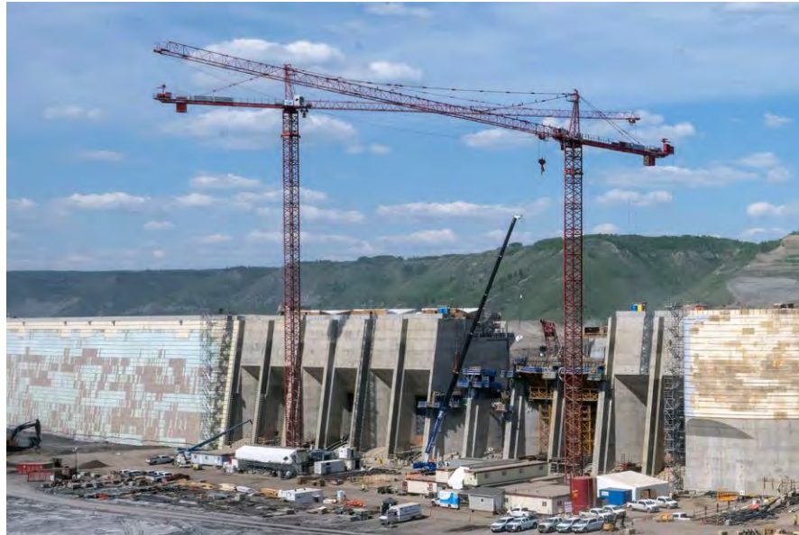
Figure A-7 The Intake structures for units 1, 2, 3 and 6 are at full elevation and construction on the intake structures for units 4 and 5 continues | June 2022
