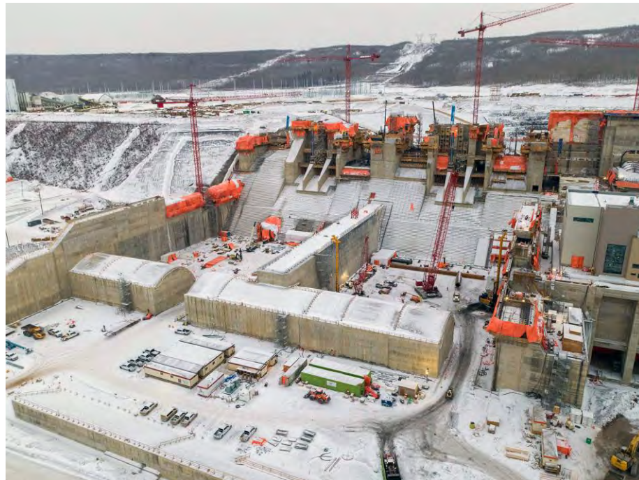
Figure A-2 Construction on the spillways including foundation enhancements and drilling of the west bay | January 2022
