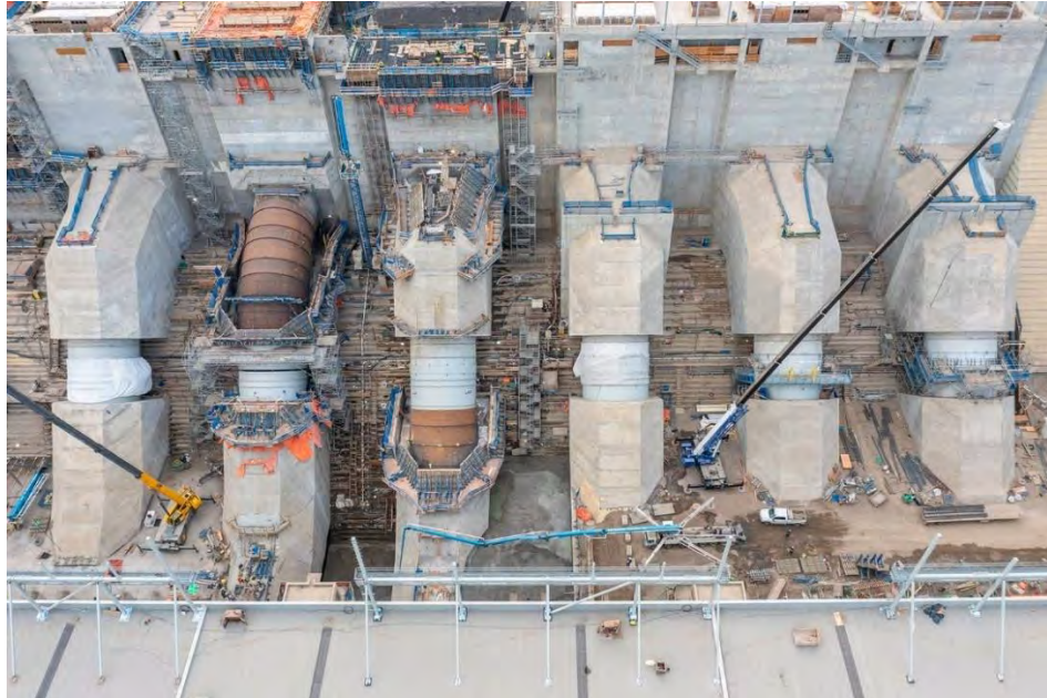
Figure A-17 Penstock units 1 (right) to 6 (left) at various stages of construction | October 2022
