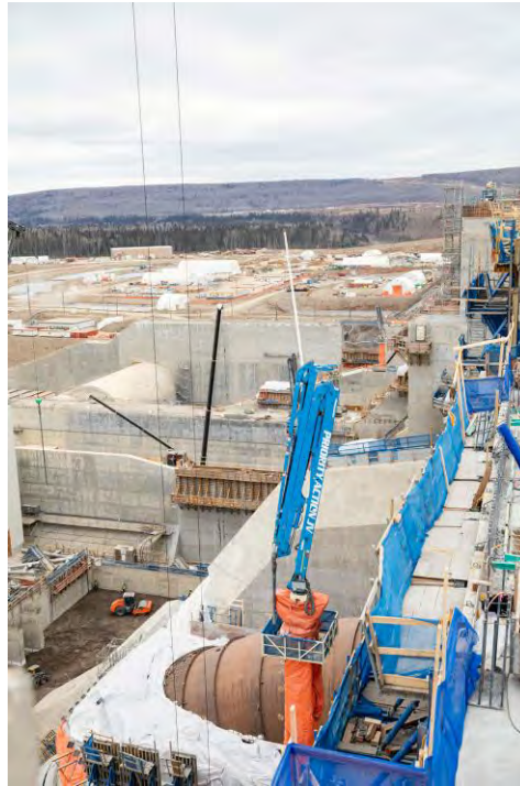
Figure A-23 Hoarding and heating (under the plastic sheeting) to protect from the cold while placing concrete at the penstocks | November 2022
