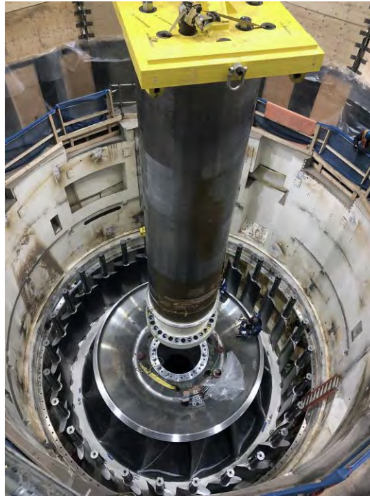
Figure A-25 Lowering unit 1 turbine shaft into position on the turbine runner. The shaft connects the turbine to the generator on the generating unit | November 2022
