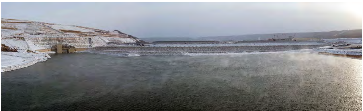
Figure A-30 The inlet portals (left) where the Peace River enters the diversion tunnels, and the earthfill dam (centre) being built. | November 2022
