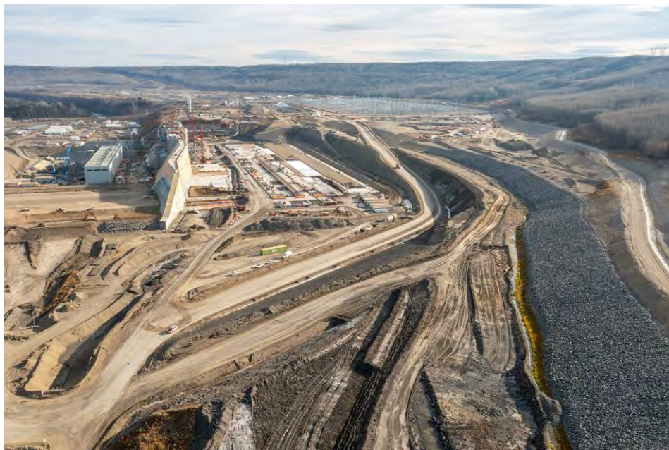
Figure A-16 East-facing view of the approach channel, where riprap (grey material on the right of the picture) defines the outer edge of the channel | October 2022
