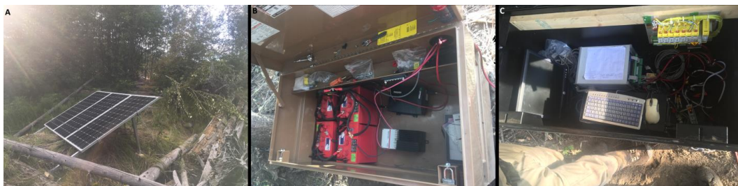
Figure 5. A) Solar panel array charged a battery bank B) to create a 12V power source. C) The battery bank powered the resistivity counter, video and PIT telemetry equipment.
