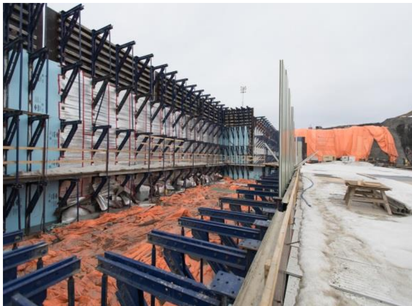
Figure A-4 Right Bank Insulation Placement on the Face of the Roller-compacted Concrete. Photo taken April 19, 2018.
