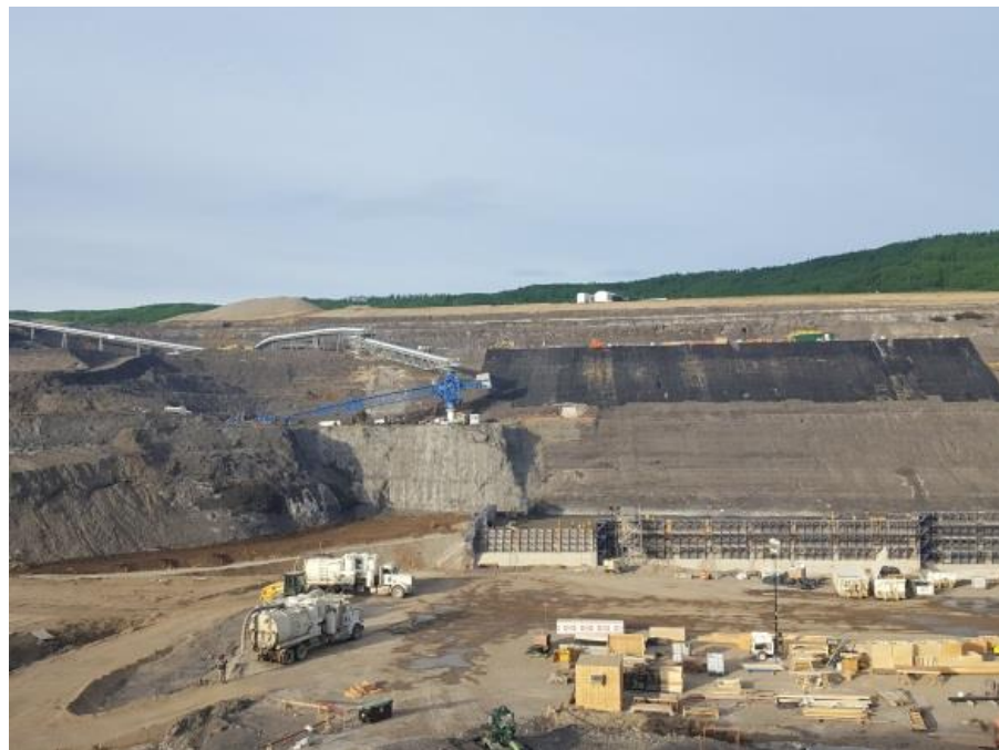
Figure A-6 Roller-Compacted Concrete Placement on the Right Bank for the Powerhouse Buttress. Photo taken May 2018.
