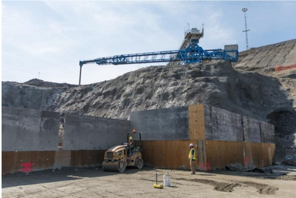
Figure A-9 Roller Compacted Concrete Placement and Shotcrete Application at the Spillway Buttress on the Right Bank. Photo taken June 22, 2018.
