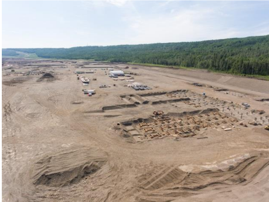
Figure A-7 Placing Concrete Foundations for the Substation on the Right Bank. Photo taken June 22, 2018.
