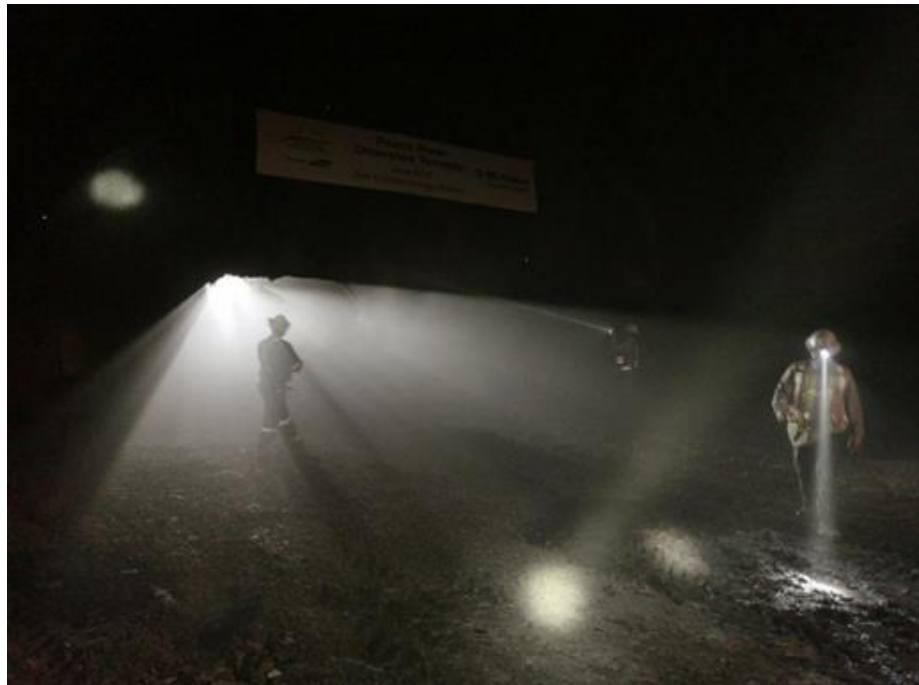
Figure A-10 Crews inspect the opening that connects both ends of the diversion tunnel excavations shortly after breakthrough in Tunnel 1 (June 2019).
