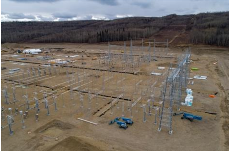
Figure A-3 Construction of the 500 kV Site C Substation on the right bank. The structural steel and equipment installations are in progress (April 2019).
