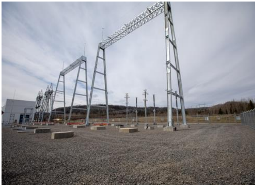
Figure A-2 Two new 500 kV gantries (5L5, 5L6) have been installed at the Peace Canyon Substation to receive the 500 kV lines from Site C. A gantry is where the transmission lines tie onto and anchor at the substation (April 2019).
