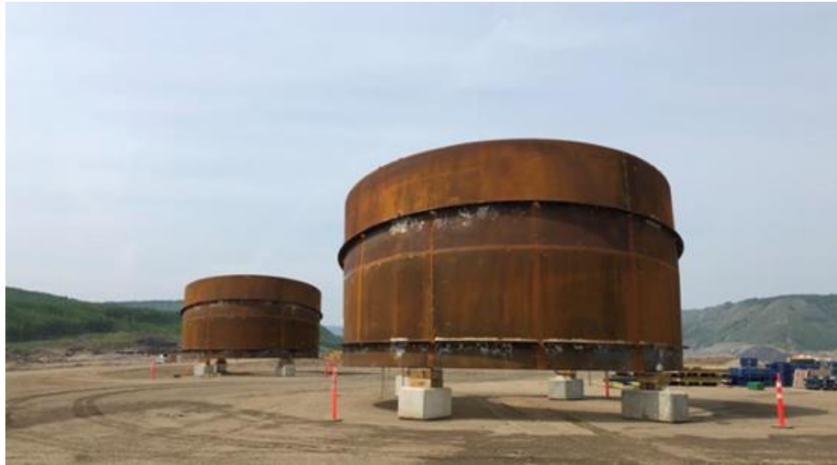
Figure A-7 We will be building and assembling 84 of these penstock sections over the next few years, to create the six penstock pipes for Site C's generating station (May 2019).
