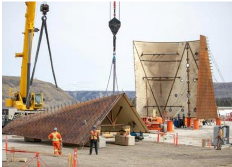
Figure A-6 After moving individual sections from a fabrication shop in Fort St. John, we assemble the penstocks on site. This is one of the six transition pieces which will funnel water from the river into our generating station (May 2019).
