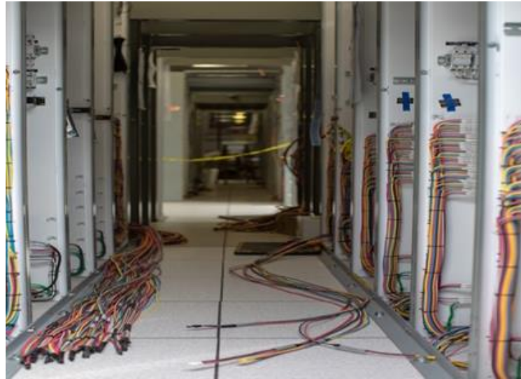
Figure A-1 Twenty-two new protection and control panels at Peace Canyon have been added and/or upgraded in preparation to receive the transmission from Site C (April 2019).
