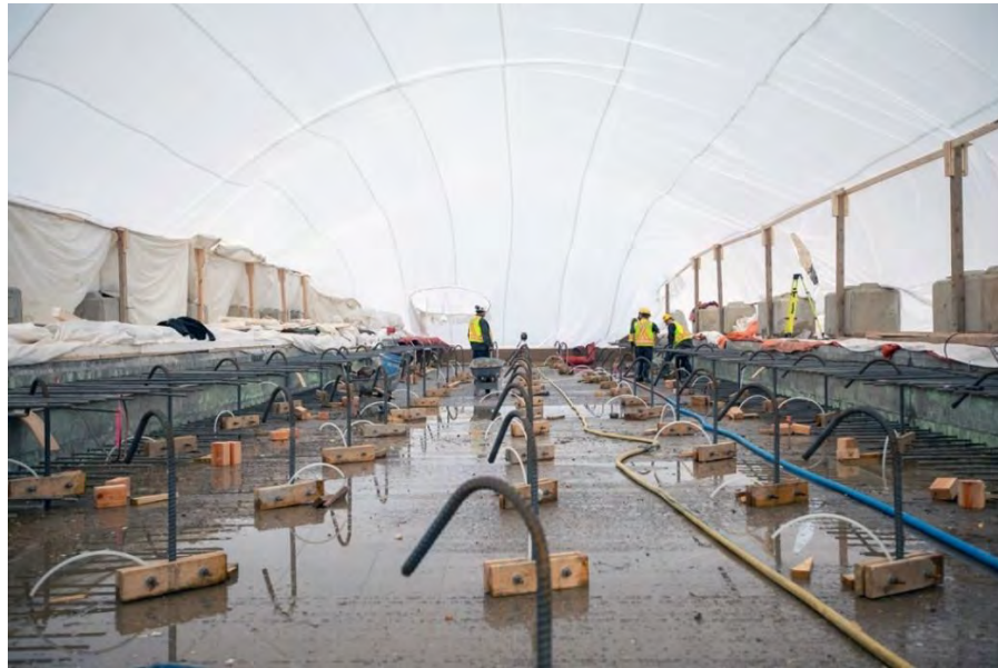
Figure A-37 Preparing Rebar Dowels for Grouting in the Spillway Stilling Basin, which will Anchor the Slabs to the Roller-compacted Concrete. About 8,000 Dowels will be Installed at Depths between Four to 13 metres in the Concrete below (November 2019)
