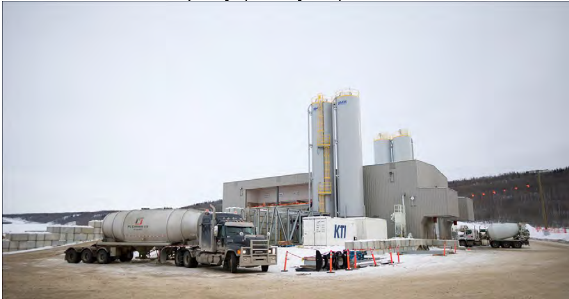
Figure A-5 On-site Concrete Batch Plant is used to Mix Concrete for the Generating Station and Spillways (February 2019)
