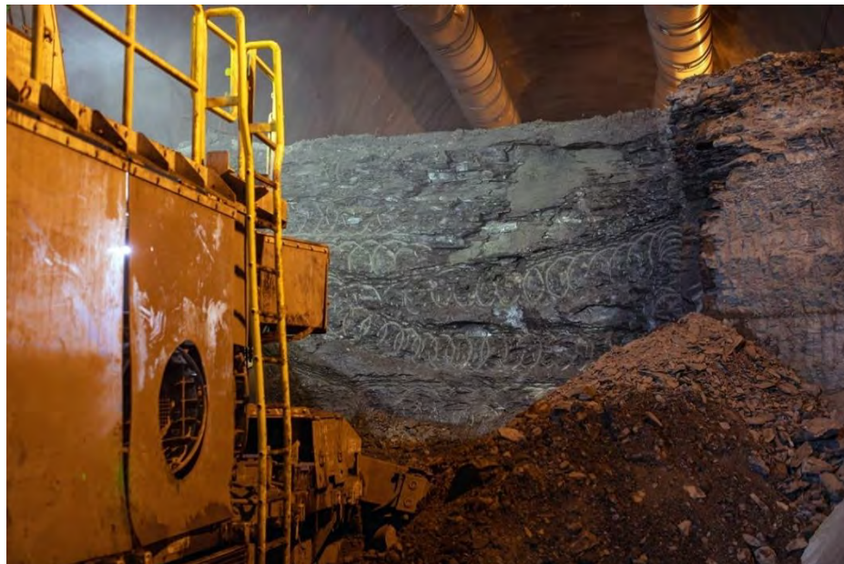
Figure A-32 Excavation of the Lower Half of a Diversion Tunnel (November 2019)
