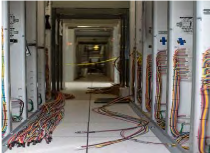
Figure A-9 Twenty-two New Protection and Control Panels at Peace Canyon have been Added and/or Upgraded in Preparation to Receive the Transmission from Site C (April 2019).
