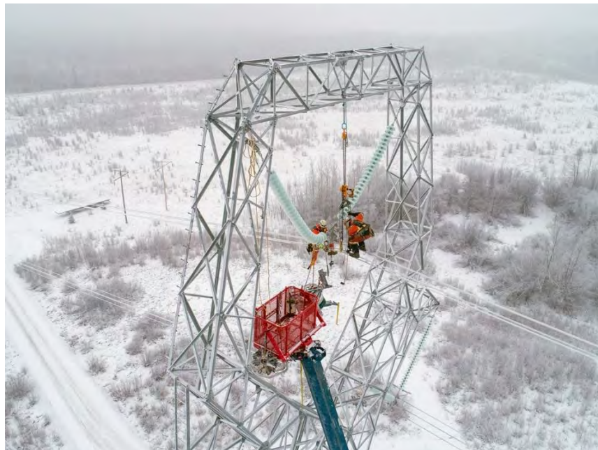
Figure A-42 Power Line Technicians Clip Conductors into the New Transmission Line Insulator Assembly (December 2019)
