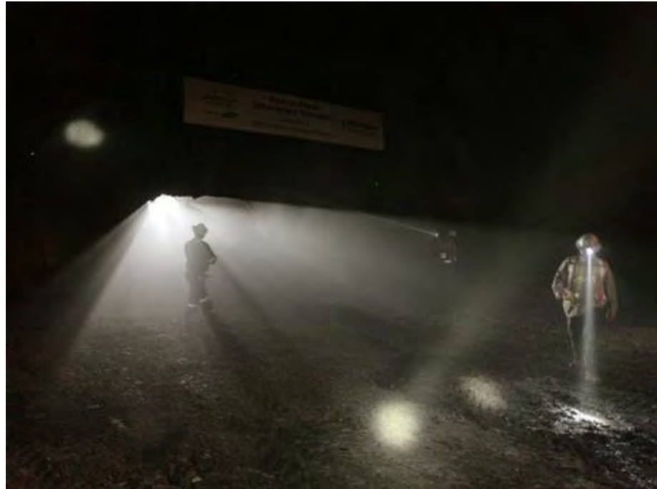
Figure A-15 Crews Inspect the Opening that Connects both Ends of the Diversion Tunnel Excavations Shortly after Breakthrough in Tunnel No. 1 (June 2019)
