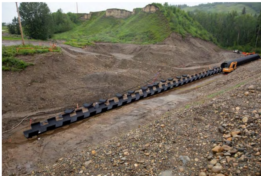
Figure A-18 Assembly of a Multi-plate Culvert that will Provide Drainage under a Realigned Segment of Highway 29 in the Cache Creek Area. A variety of Culverts are Being Installed as Part of the Highway 29 Realignment (July 2019)
