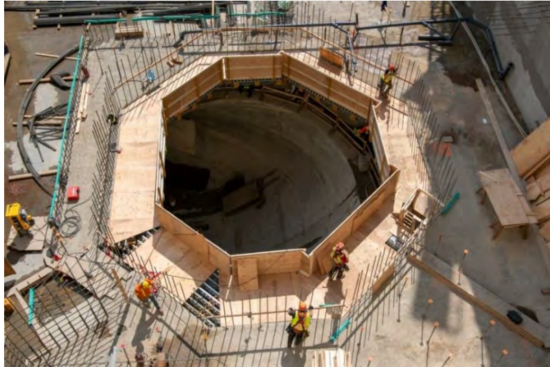
Figure A-17 View of Inside the Unit 1 Draft Tube in the Powerhouse. Once Site C is Operational, Water will Enter the Penstocks, Move through the Turbines and then be Released into the Draft Tubes prior to Exiting through the Tail Race (July 2019)
