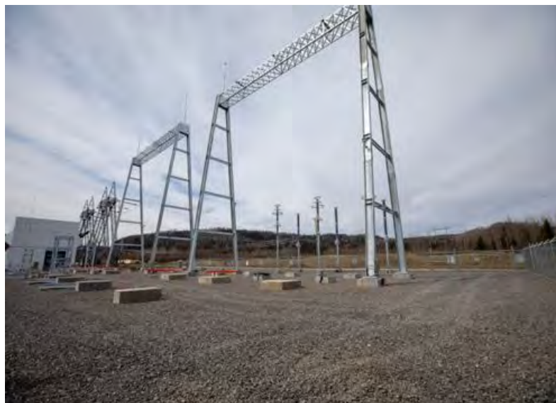
Figure A-10 Two New 500 kV Gantries (5L5, 5L6) have been Installed at the Peace Canyon Substation to Receive the 500 kV Lines from Site C. A Gantry is where the Transmission Lines Tie onto and Anchor at the Substation (April 2019).
