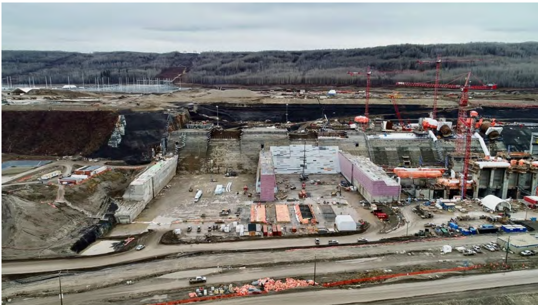
Figure A-24 Looking South at the Spillways Buttress (Left) and the Construction of the Site C Powerhouse (Right) (October 2019)
