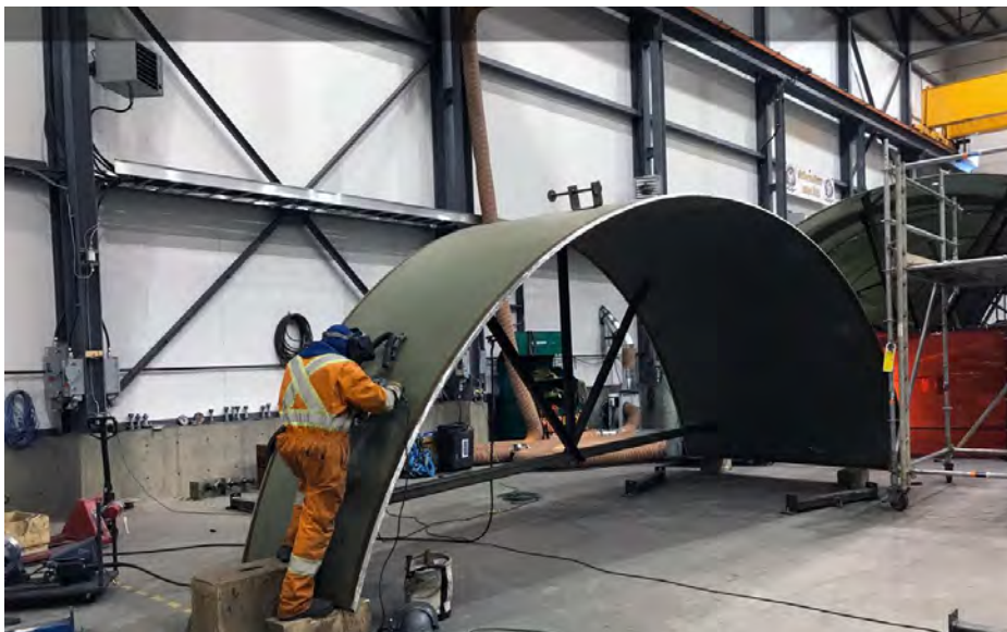
Figure A-2 A Welder Works on Part of the Spiral Case in the On-site Turbines and Generators Manufacturing Facility (January 2019)
