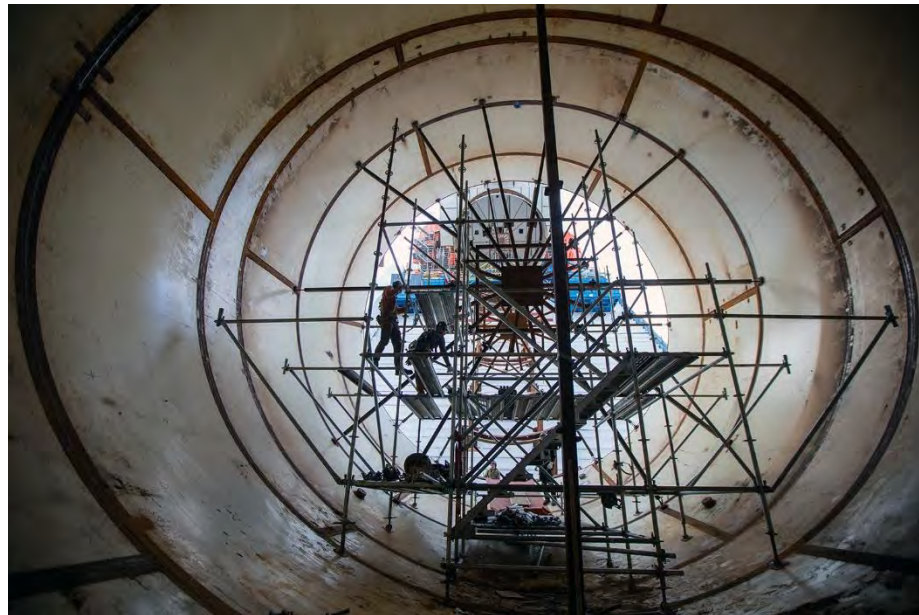
Figure A-36 Scaffolding is Installed Inside a Penstock to Allow Access Around the Circumference of the Init to Weld Sections together (November 2019)
