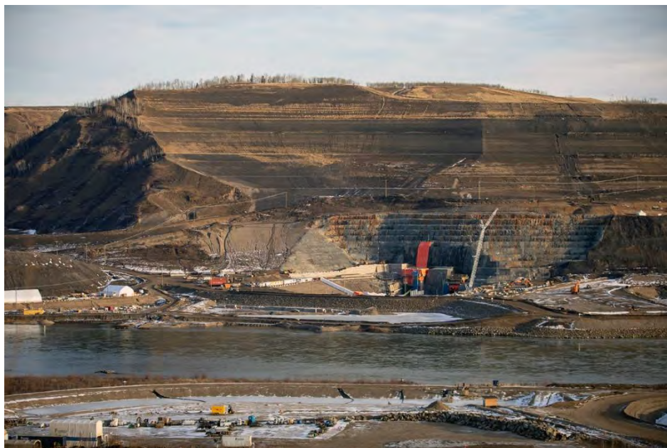
Figure A-34 View of the Tunnel Inlet Portal with the Inlet Bypass Road and Diversion Structures under Construction (November 2019)
