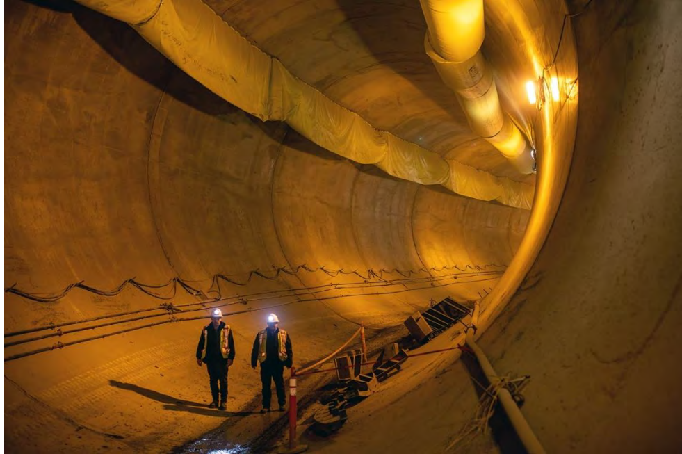
Figure A-31 Workers Walk through a Segment of One of the Diversion Tunnels, Recently Lined with Concrete (November 2019)
