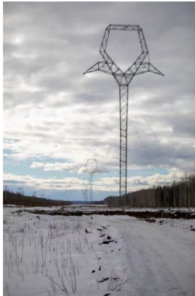
Figure A-7 As of March 31, 2019, 51 Towers had been Raised along the 75-Kilometre-Long Transmission Line Corridor. In Total, 405 Towers will Hold Up Two New 500 kV Transmission Lines, which will Connect Site C Power to the Rest of BC Hydro's Grid (February 2019)
