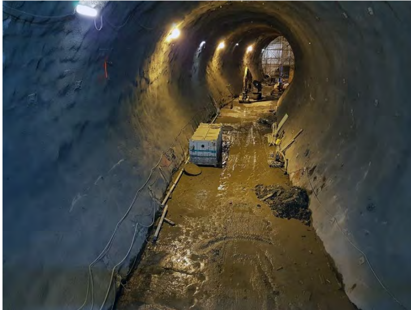
Figure A-39 In Late December 2019, we Substantially Completed Excavations in the Two Peace River Diversion Tunnels. The Tunnels are Temporarily Coated with Shotcrete until the Permanent Concrete Liner is Installed (December 2019)
