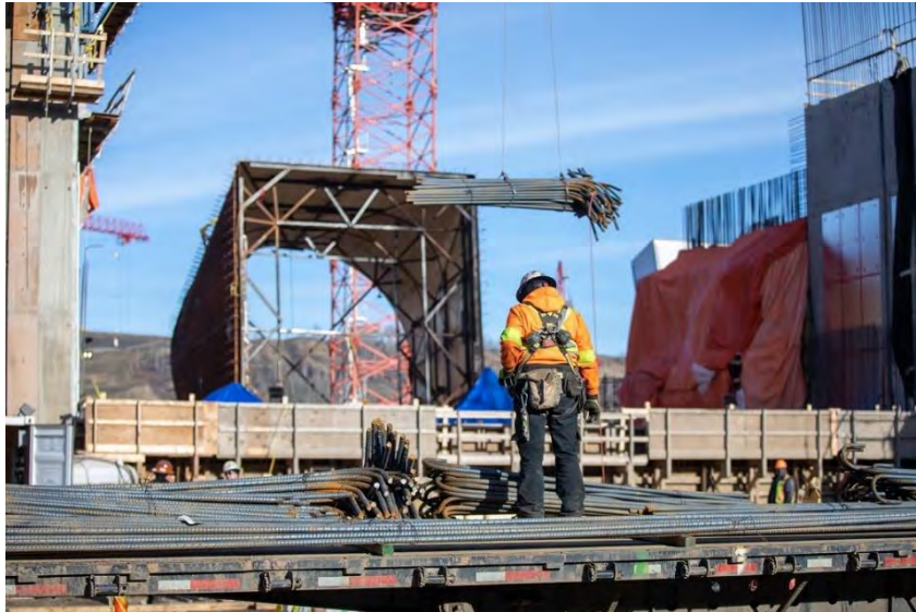
Figure A-29 Rebar is being Delivered at the Intake Area where it will be Used to Reinforce the Concrete Intake Structures. More than 5,000 tons of Rebar will be Installed in the Six Intake Structures (October 2019)
