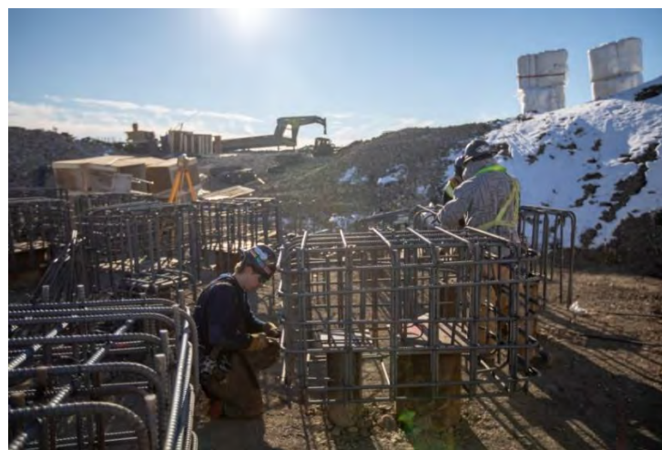
Figure A-8 This Photograph shows Work Underway on the Five-Kilometre-long Electric Conveyor System that will Move Excavated till Material from the 85 th Avenue Industrial Lands to the Dam Site for Construction of the Site C dam. Piles have Concrete Caps with Bolt Settings onto which the Conveyor Structure is Bolted (March 2019)
