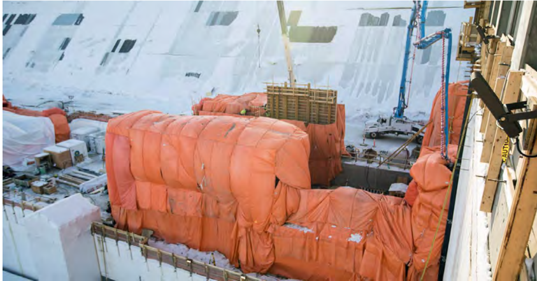
Figure A-3 Hoarding and Heating Protects Concrete from the Cold as it is Placed at the Generating Station's Double Chamber Walls (January 2019)
