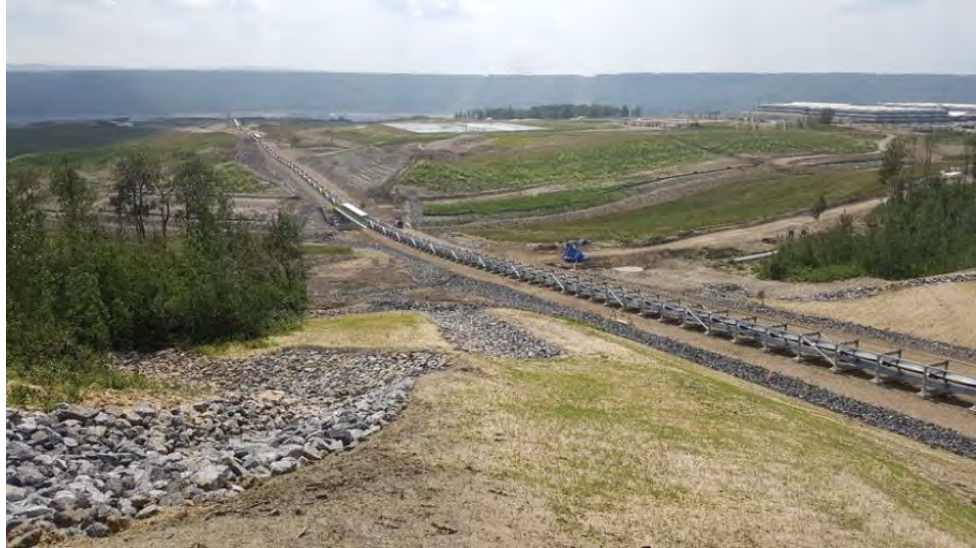
Figure A-21 The Five-km Conveyor System, which Runs from the 85 th Avenue Industrial Lands to the Dam Site (September 2019)
