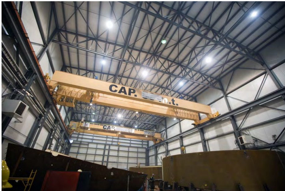
Figure A-1 Overhead Cranes in the Workshop in Fort St. John where the Penstock Parts are Assembled. Penstocks are Ten-Metre-Wide Pipes that Move Water from the Reservoir Intakes to the Turbines (January 2019)
