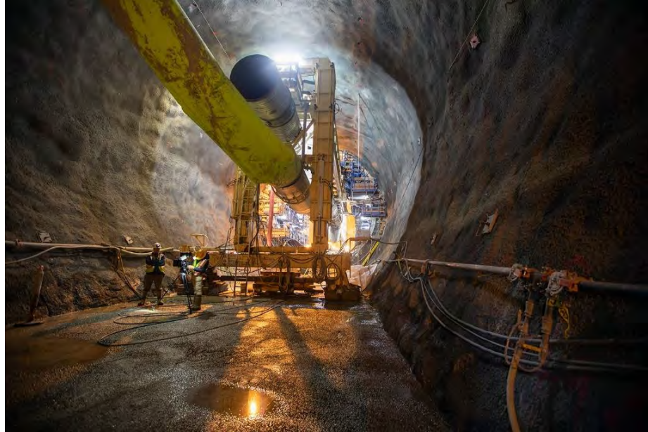
Figure A-33 Inside One of Two Diversion Tunnels where a Slip form Places Concrete (November 2019)
