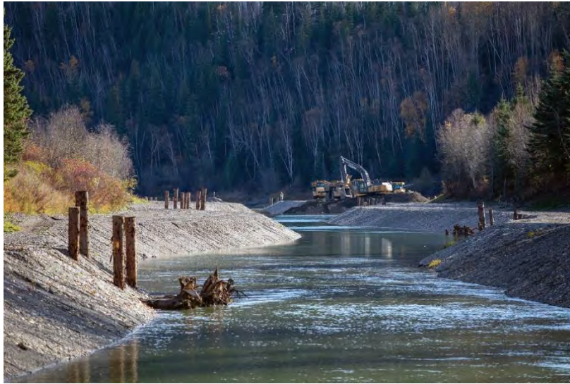
Figure A-27 Back Channel Enhancement Project Created Approximately Two Hectares of Permanent New Wetted Fish Habitat. Areas with Water Fluctuations are Filled in to Prevent Fish Stranding. Engineered Logjams Provide Rearing Habitat for Juvenile Fish (October 2019)
