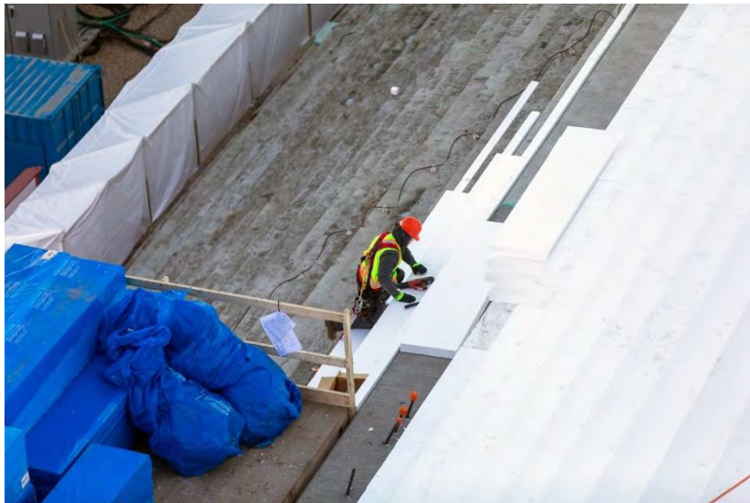
Figure A-28 A Worker Insulates the Steps and Slope of the Powerhouse Buttress. As it Gets Colder Outside it is Necessary to Reduce the Temperature Difference Between the Core and the Surface of the Concrete to Prevent Cracking (October 2019)
