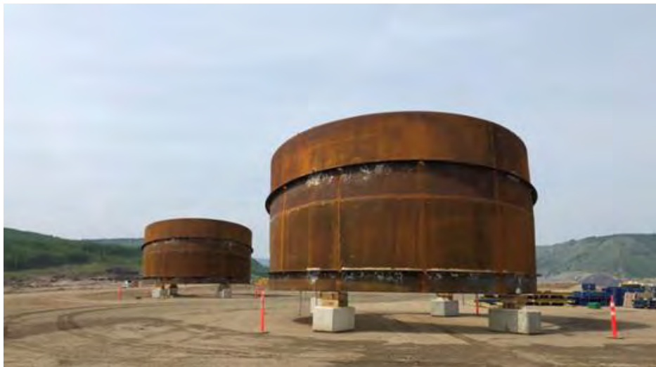
Figure A-12 We will be Building and Assembling 84 of these Penstock Sections over the Next few Years, to Create the Six Penstock Pipes for Site C’s Generating Station (May 2019)
