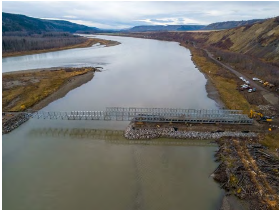
Figure A-22 Construction Starting on a Temporary Bridge to an Island in the Peace River Near Halfway River, as Part of Clearing Activities for the Project. (September 2019)
