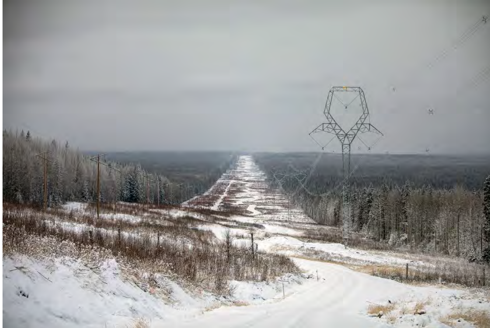
Figure A-41 Towers with Stringing Complete, as Part of the New 75 km Transmission Line (December 2019)
