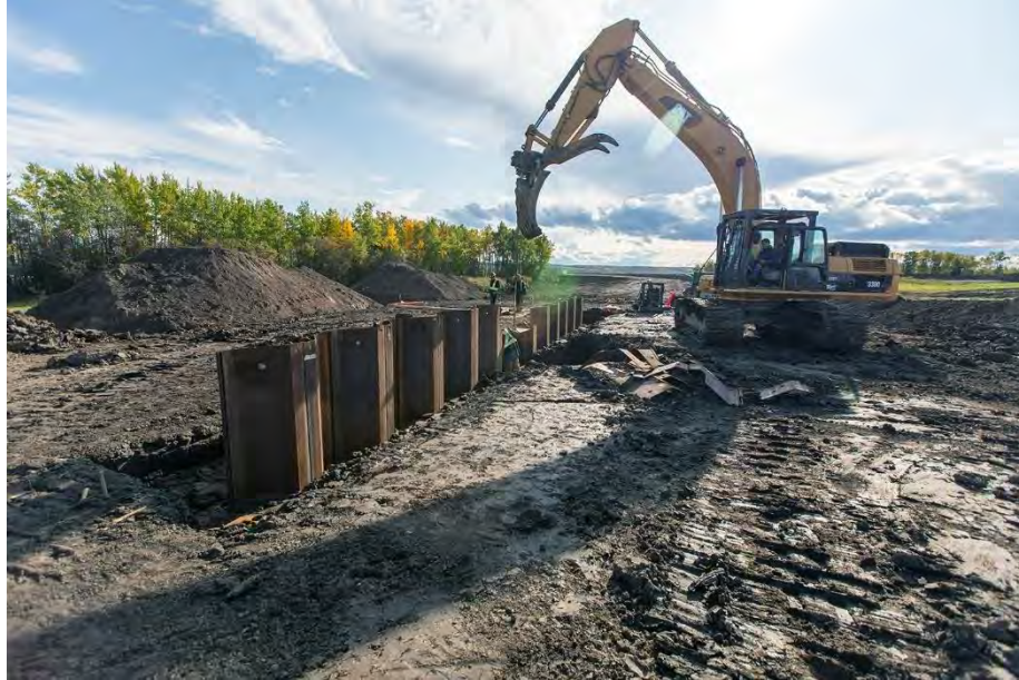
Figure A-23 Levelling of Sheet Piles for the Water Control Structure in the Main Basin of the Golata Creek Wetland (October 2019)
