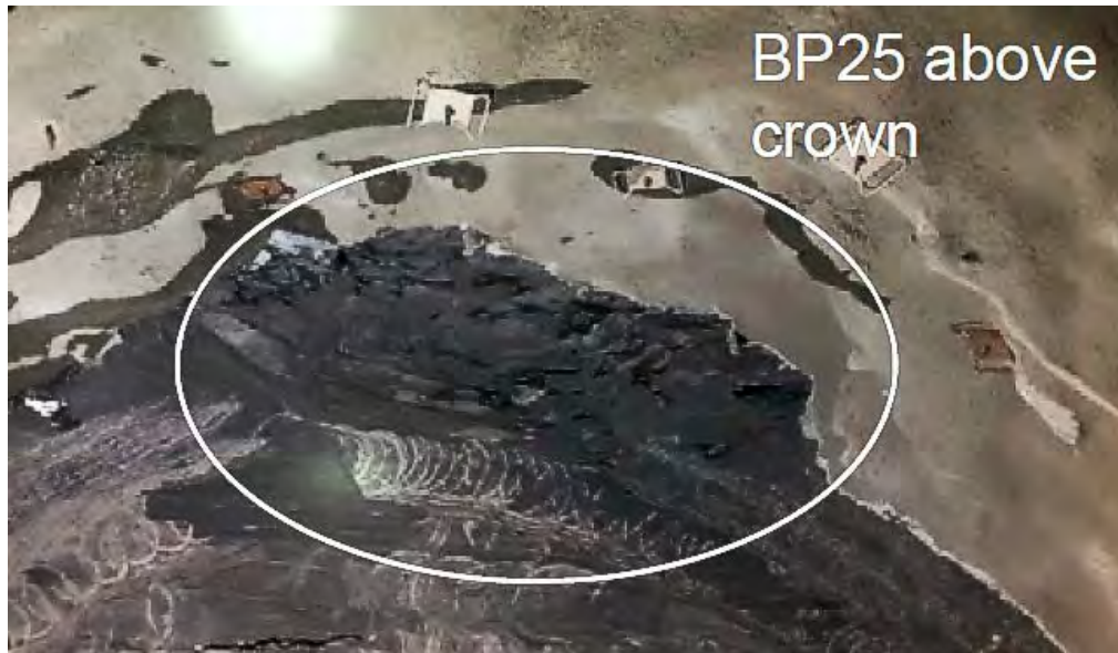
Figure 2: Buckling of shale in the crown of Diversion Tunnel No. 2
