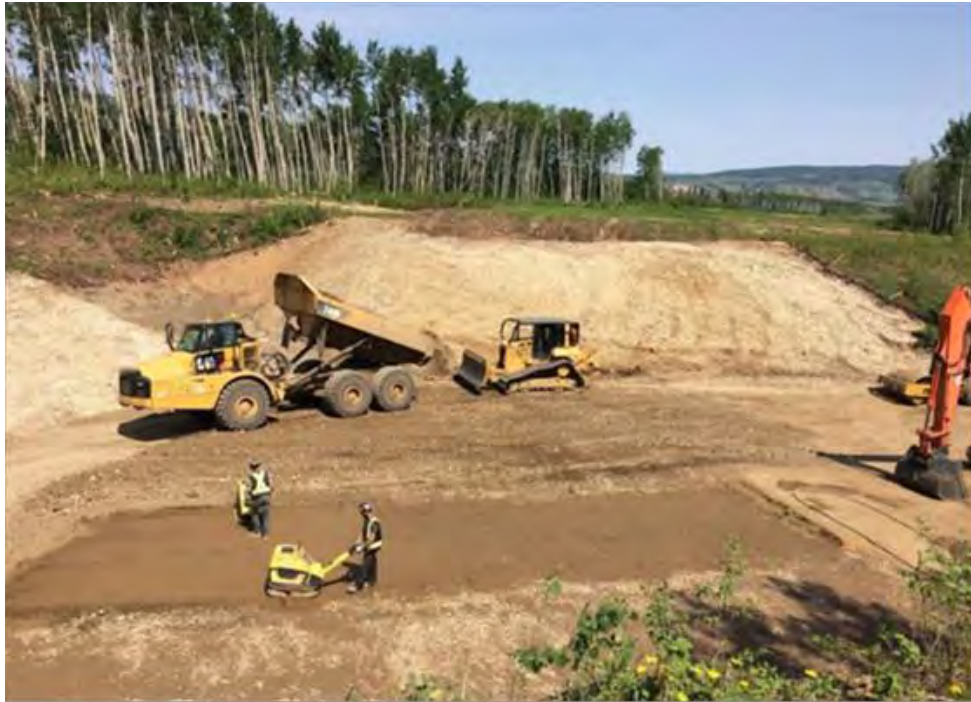
Figure A-13 Grading and Levelling Occurring on the New Alignment of Highway 29 at Cache Creek West (June 2019)
