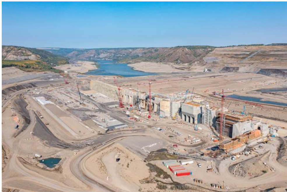
Figure A-6 The ongoing construction of the approach channel, looking upstream (September 2022)
