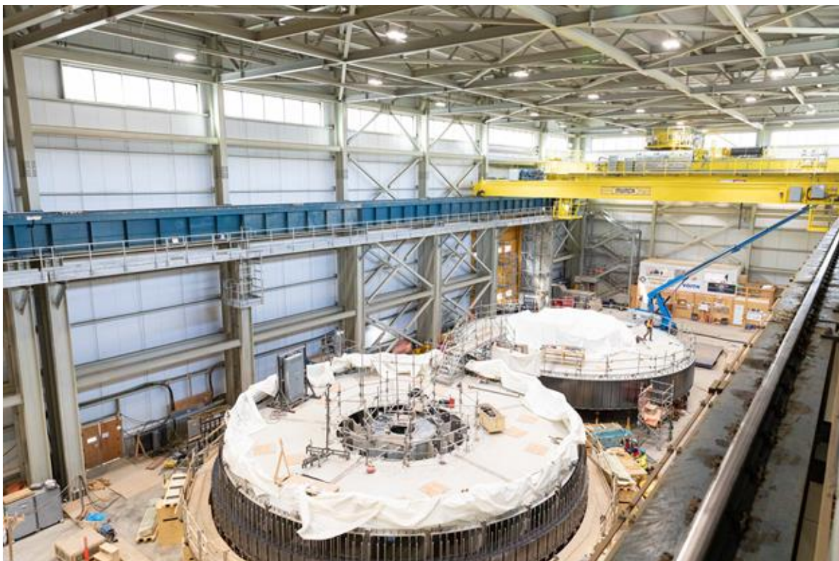
Figure A-10 Generator rotors for units 1 and 2 being assembled in the powerhouse service bay, as an additional bridge crane is assembled in the background (September 2022)
