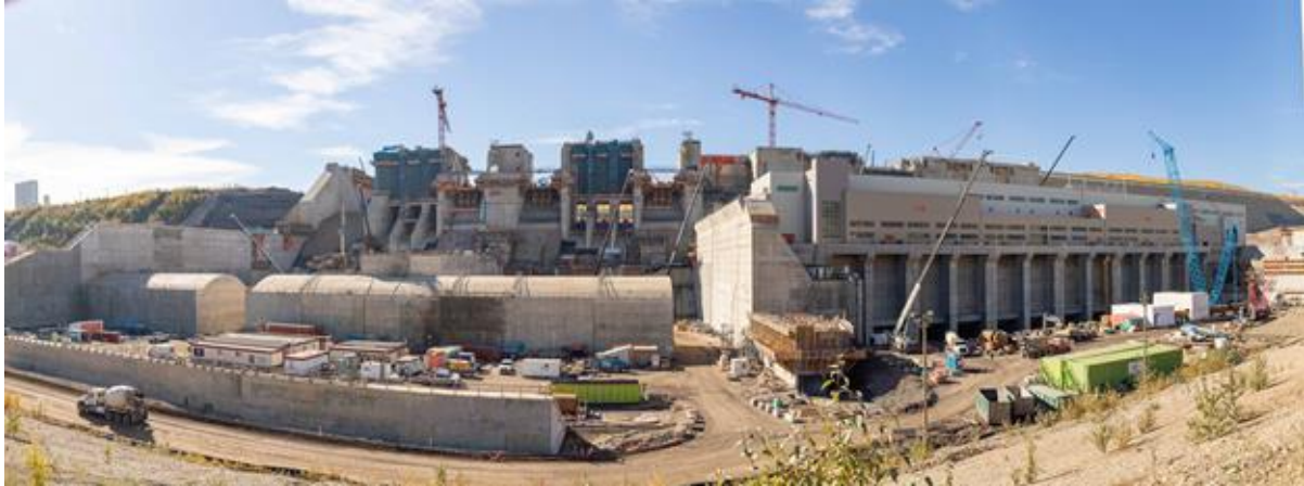
Figure A-9 Construction of the Site C spillways and stilling basin, powerhouse and tailrace (September 2022)
