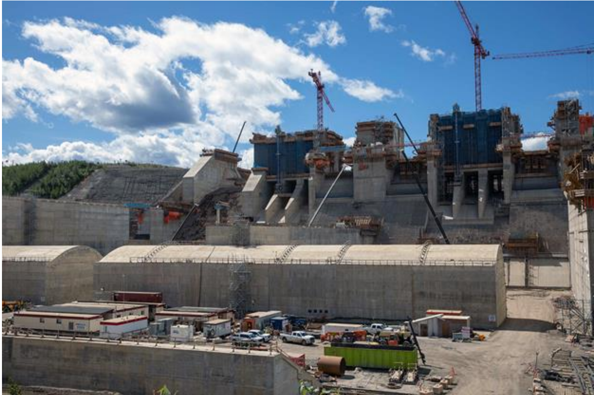
Figure A-3 Construction of the spillway upper headworks and stilling basin (July 2022)
