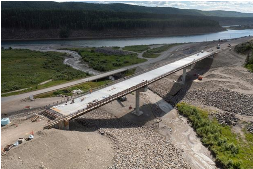
Figure A-2 Concrete deck placements being completed for the Lynx Creek bridge on Highway 29 (July 2022)
