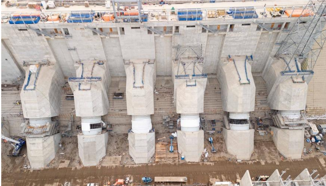
Work continues on the six penstocks that will direct water into the powerhouse. See more construction photos in our gallery.
