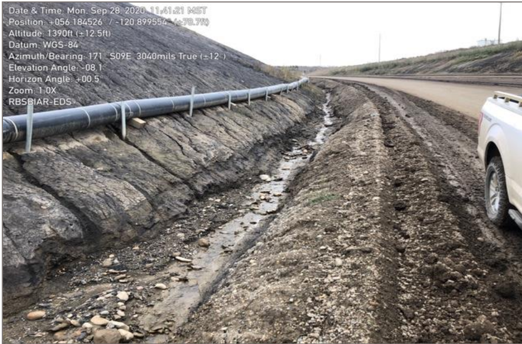
Photo 15: RBSBIAR-EDS downstream east ditch, September 28, 2020.
