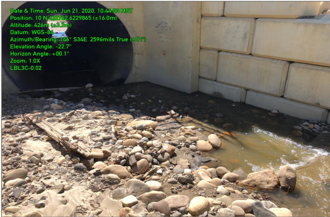
Photo 17: L3 Creek LBL3C-0.02 discharge location, June 21, 2020.
