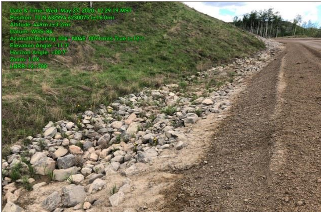
Photo 7: River Road LBRR-12+700 location, May 27, 2020.
