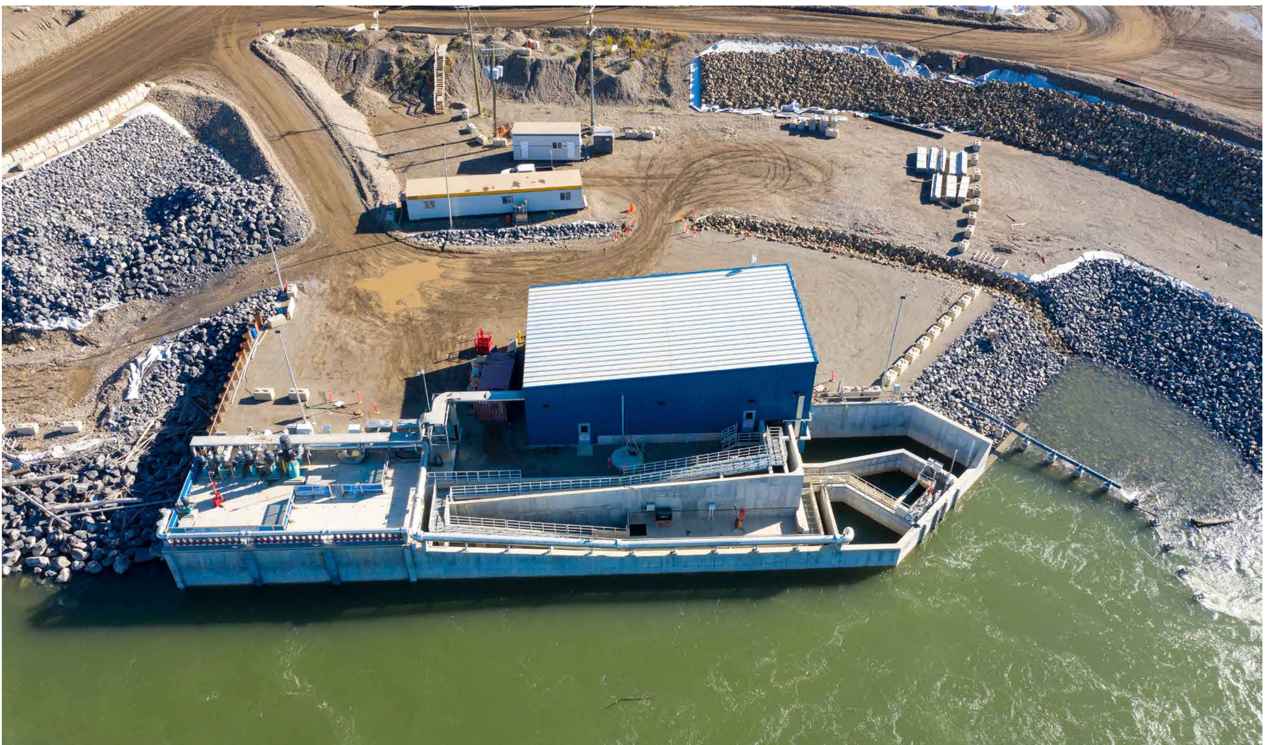
We built a temporary fish passage facility, which we used during dam construction. We used what we learned from the temporary facility to build the permanent facility.
