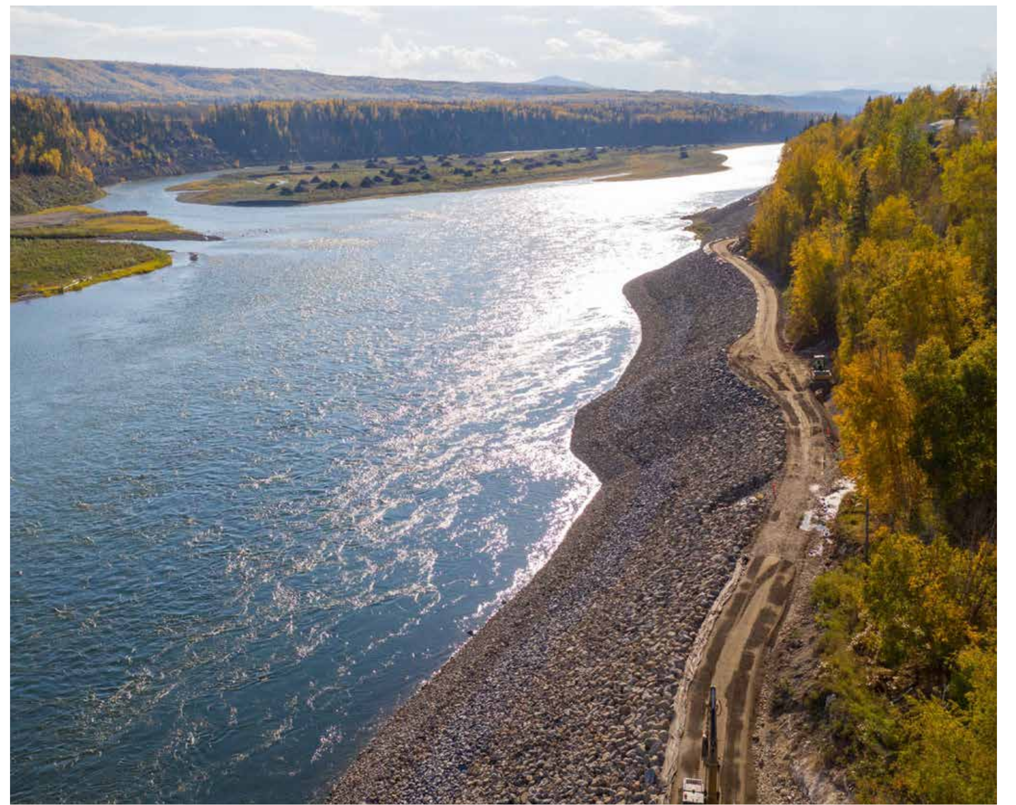
The shoreline protection berm extends for 2.6 km and is made of riprap, rocks, and gravel.
