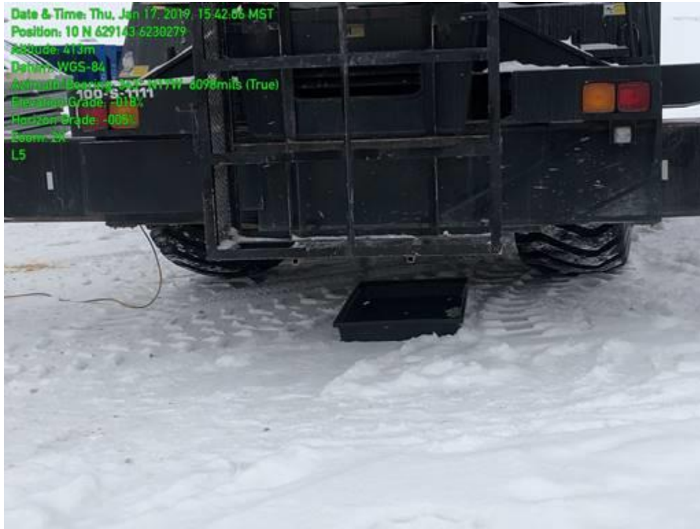
Figure 2. Crews ensure drip trays are placed under machinery parked less than 30 meters from the high-water mark at the diversion outlet cofferdam (top; January 8, 2019) and RSEM L5 (bottom; January 17, 2019).
