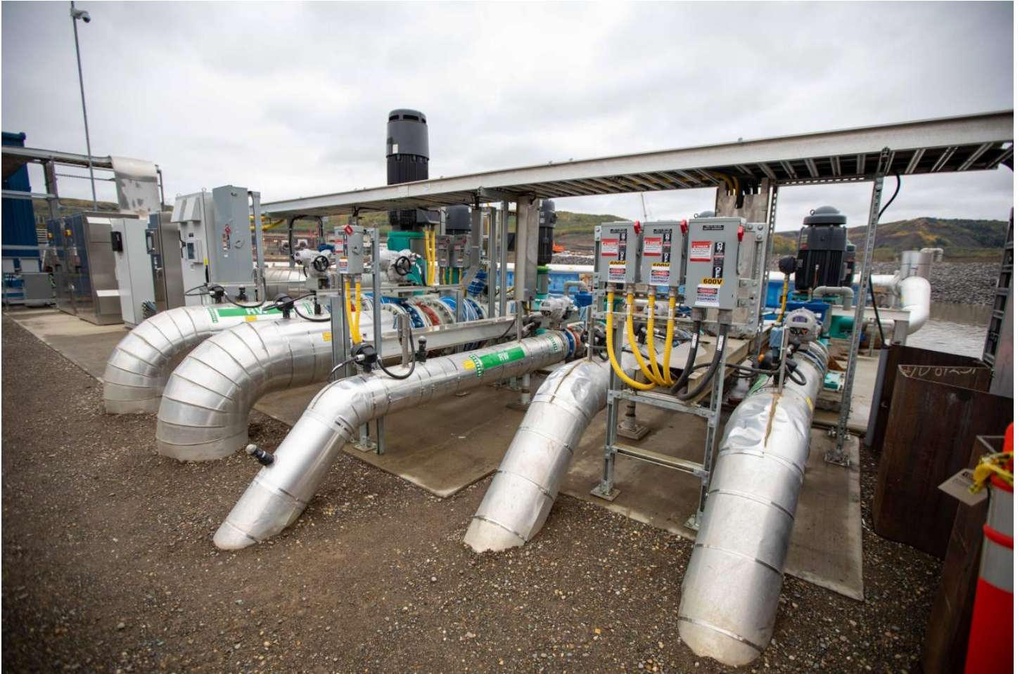
Photo 11. Ten pumps are located on site to provide flows to the fishway and the sorting facility (September 14, 2020).
