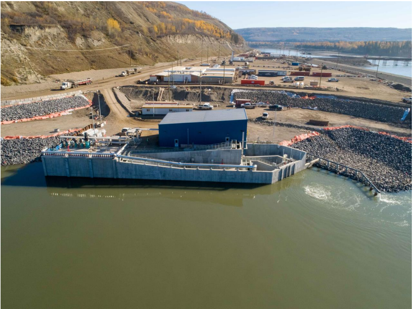
Photo 2. Overview of the temporary facility located at the outlet of the diversion tunnels (October 2, 2020).
