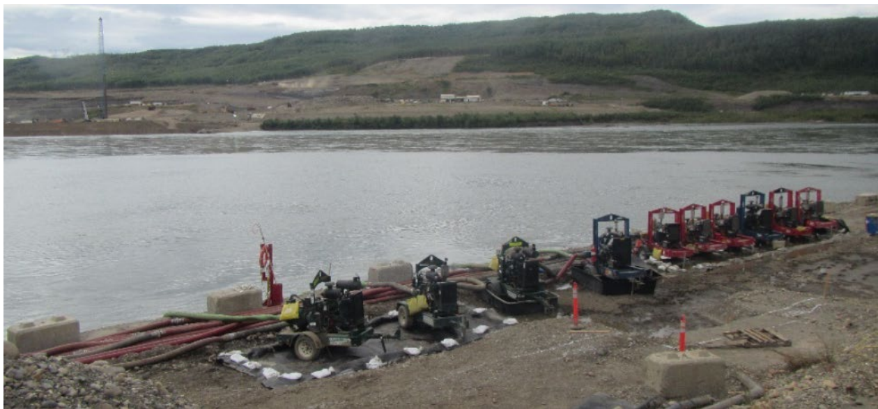
Figure 5. Diversion inlet pumps and containment. Water was pumped from the Peace River into the diversion inlet cofferdam area to balance water levels in preparation for removal of the inlet cofferdam (August 29, 2020).
