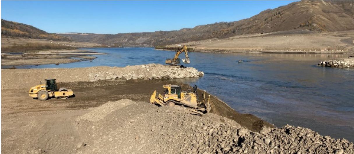
Figure 5. Rockfill berm extends from each bank of the Peace River to support river diversion. On site Qualified Environmental Professionals in place to ensure measures, including slow starts, controlled pace, and continuous of advancement, were being following to deter fish from active work areas (September 30, 2020; from south bank looking west).
