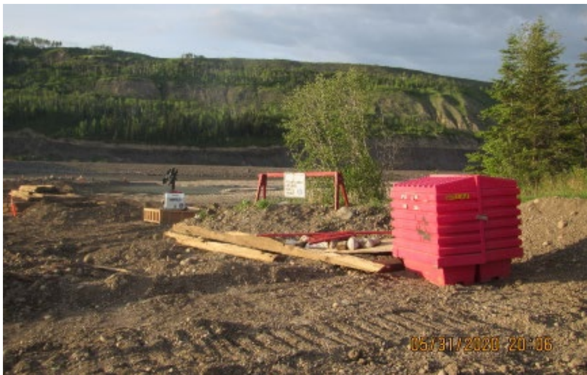
Figure 3. Spill prevention measures, including floating boom, within the dam site construction area adjacent to the Peace River (May 31, 2020).
