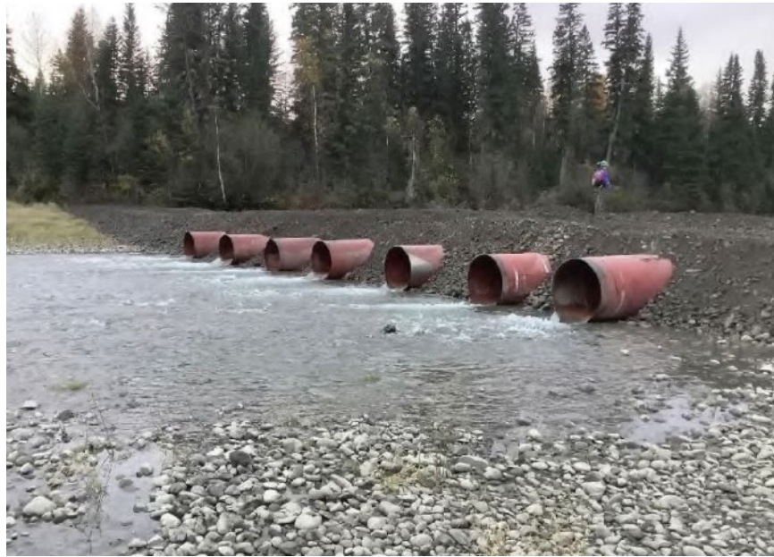
Figure 1. Temporary Peace River side channel crossings within middle reservoir clearing area. On site Qualified Environmental Professionals in place and site specific mitigation plans (September 26, 2020).
