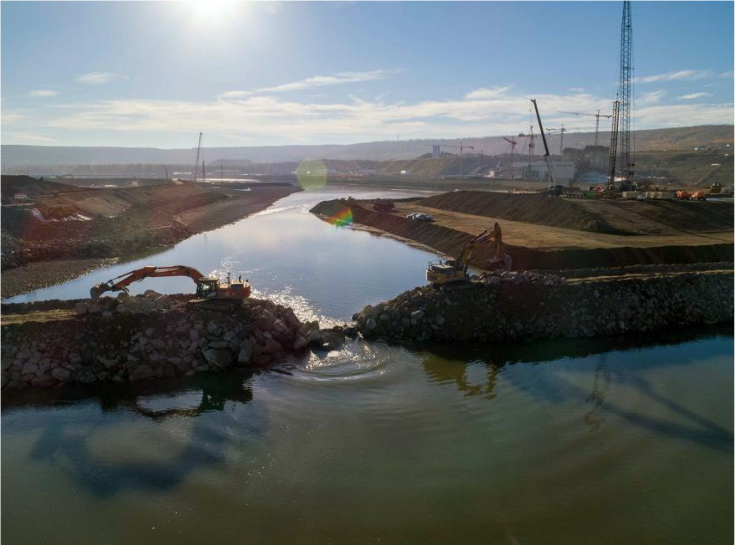
Photo 5. Final rip rap is placed on the rockfill berm (center) to close the Peace River on October 3, 2020 (looking downstream).
