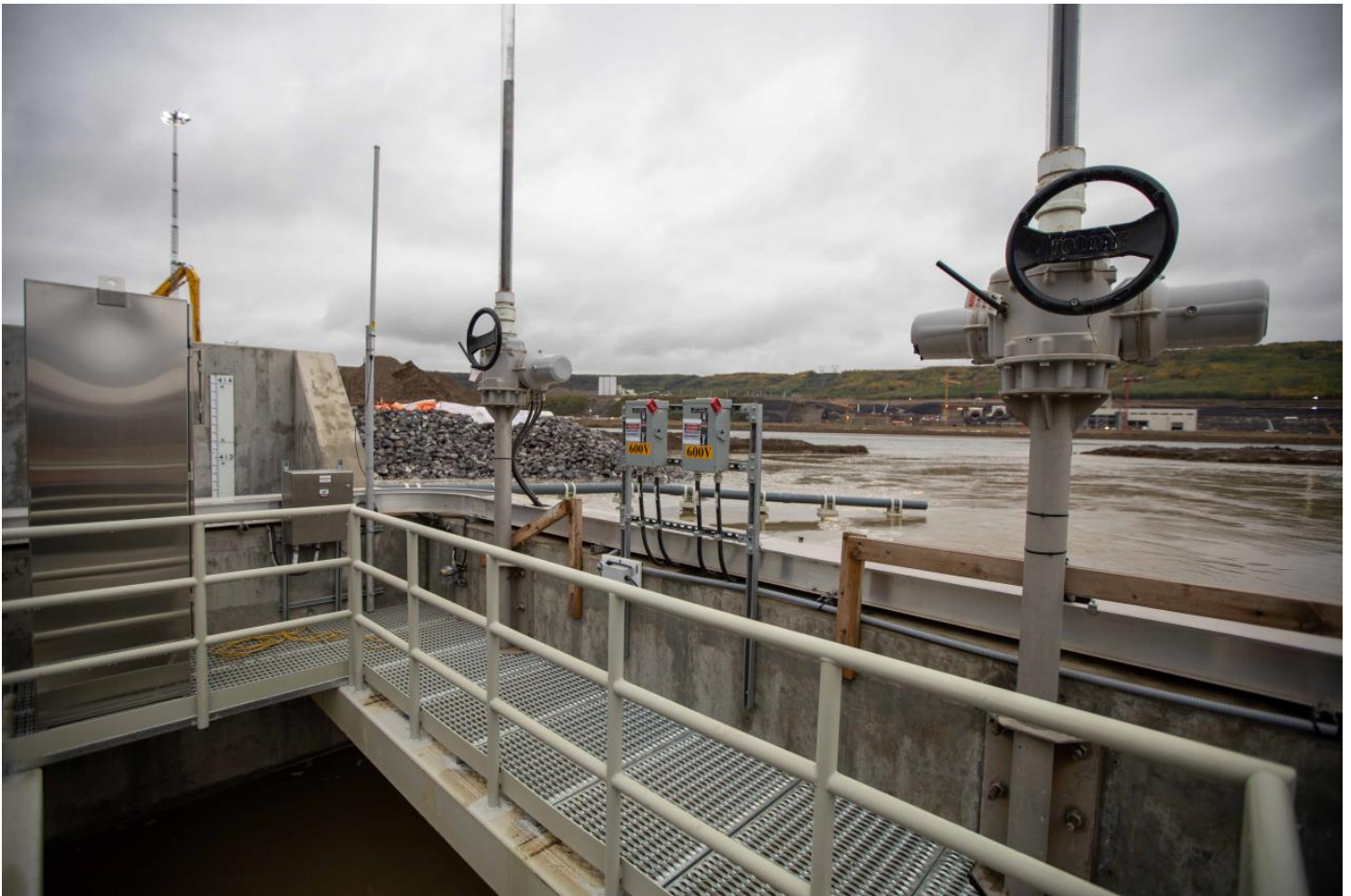
Photo 12. Two entrance gates provide the attraction flows at the fishway entrance. Gates are programmed to automatically adjust their position to maintain the same head differential between the entrance pool and the diversion tunnel outlet (September 14, 2020).
