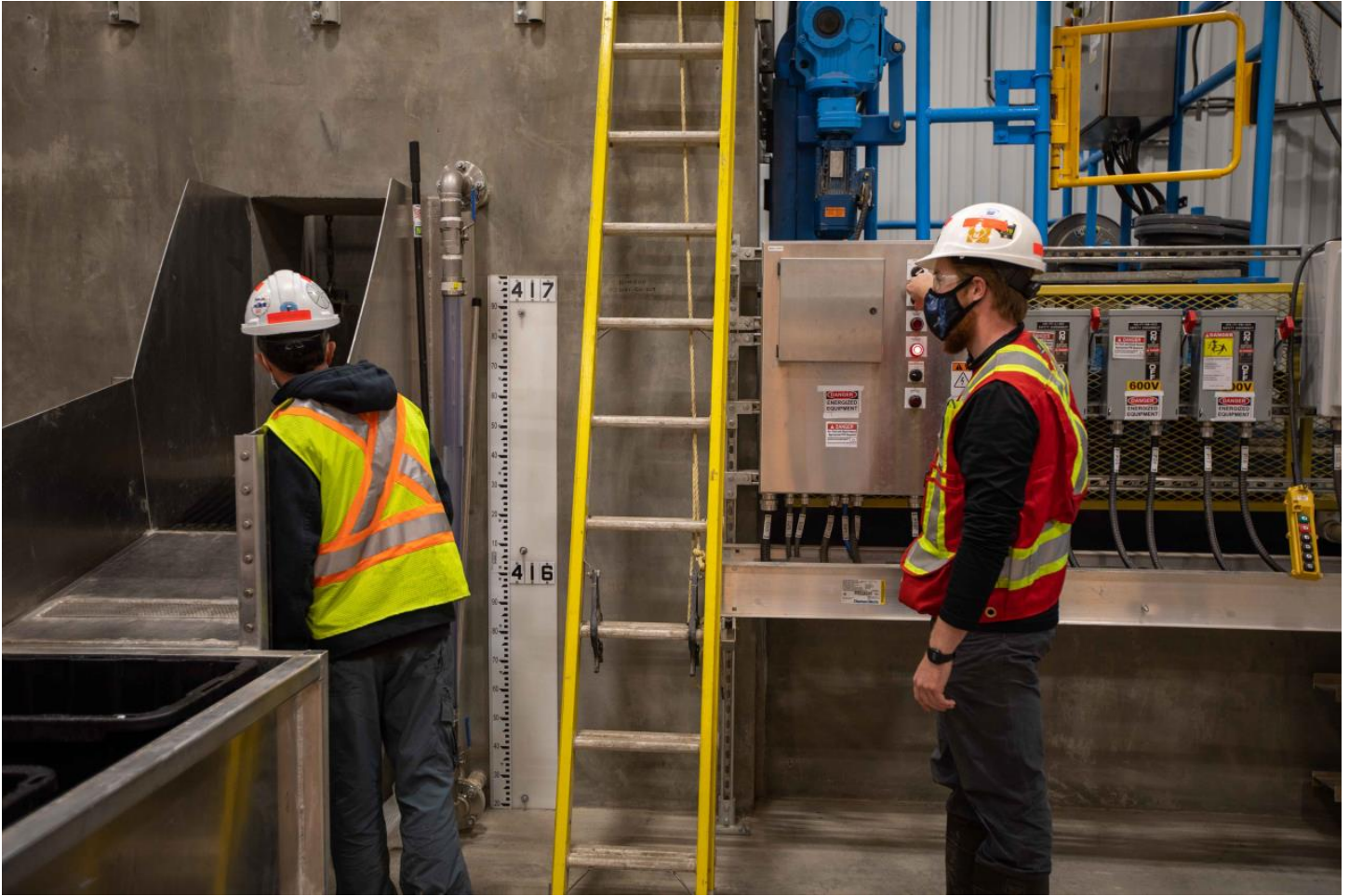
Photo 6. Workers conduct a crowding cycle during the first day of commissioning the temporary facility (September 23, 2020).
