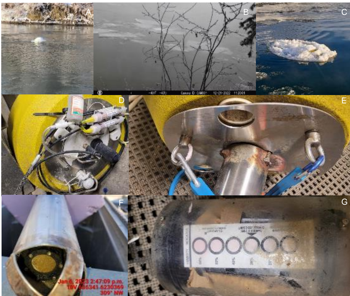
Figure 10: TDG station at Stn_112.5L with ice build-up on its dome cover (A), ice floating through the monitoring site on 21 December (B), the station without its dome cover and encased in ice on 6 January (C), damage to the topside station components (D and E), the TDG probe with biofouling (F), and moisture inside the DCP cannister (G).
