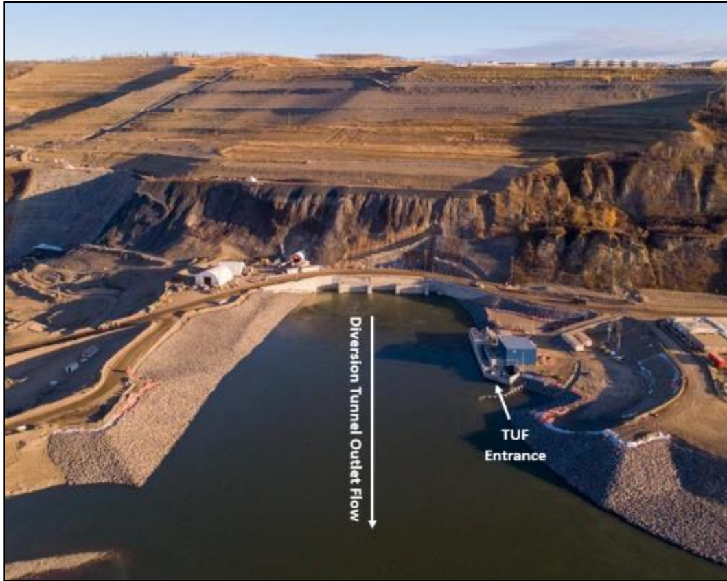
Figure 1 Aerial photo of the diverted Peace River and the temporary upstream fish passage facility (TUF) at the Site C Clean Energy Project, located on the east bank of the diversion tunnel outlet. The Peace River is diverted through two tunnels which do not allow for upstream fish passage. Photo provided by BC Hydro, June 8, 2021.
