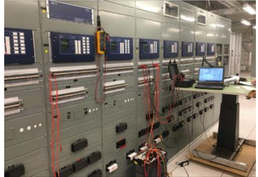
P&C relay testing & NERC hardening
