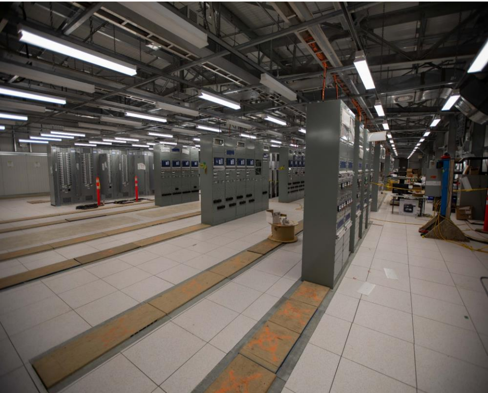
Completed protection and control panels inside of the SBK control room
