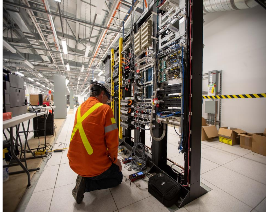
Technician confirming connectivity to Sundance Lakes Substation near Chetwynd
