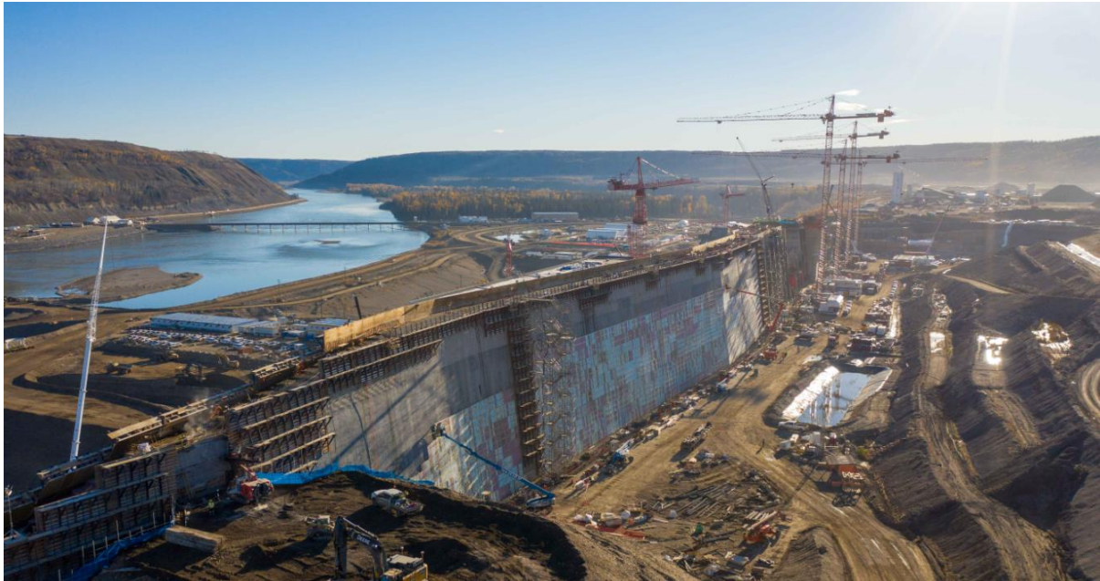
Figure A-23 Roller-compacted concrete ramps are removed from the dam and core buttress, and insulation is installed on the upstream side of the buttress (Fall 2021)
