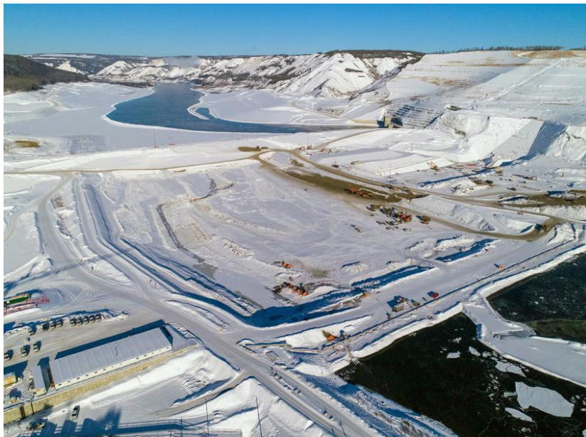
Figure A-4 The upstream and downstream cofferdams, which divert the Peace River through the two diversion tunnels (February 2021)
