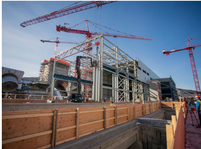
Figure A-3 Powerhouse steel superstructure construction. The powerhouse construction also includes concrete placements at the powerhouse, intakes and spillways, and the installation of penstock segments (February 2021)
