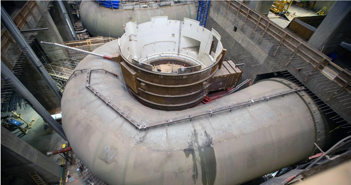
Figure A-28 Crews install the unit 1 pit liner and spiral case inside the powerhouse (December 2021)
