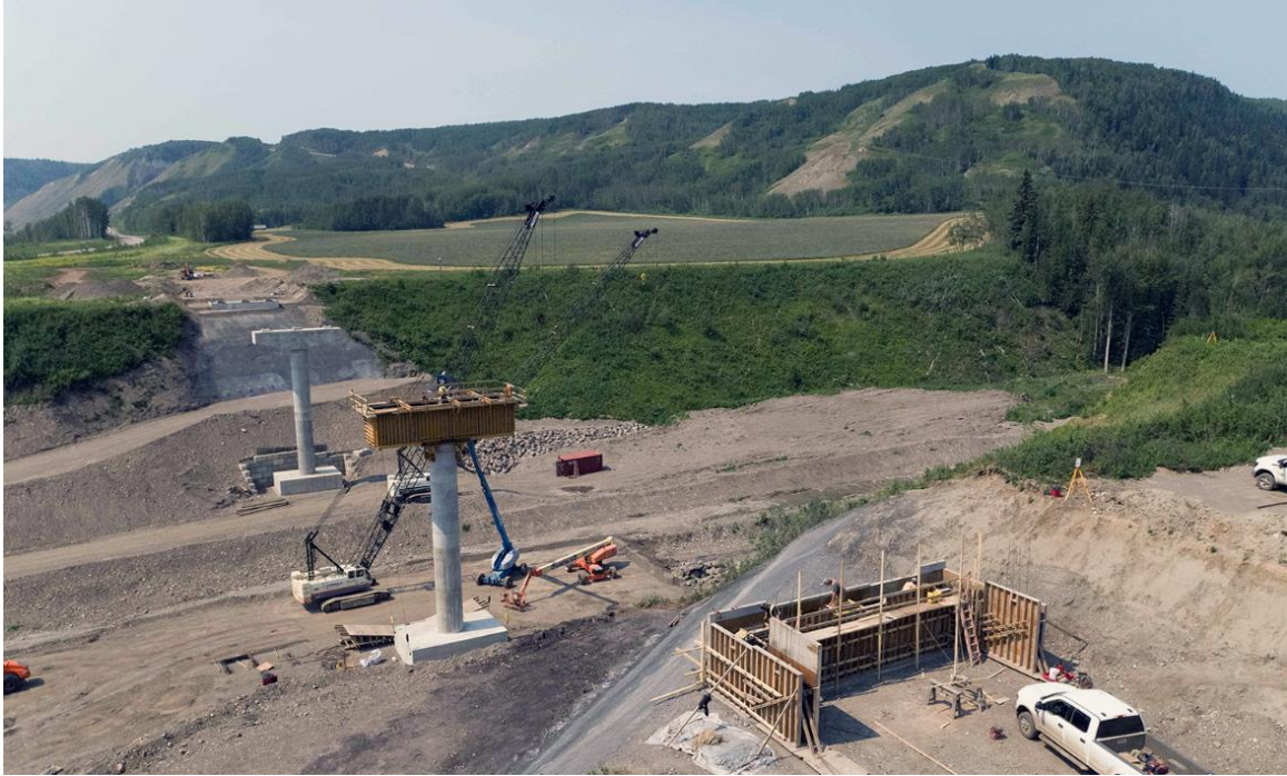
Figure A-15 Bridge formwork under construction at the Dry Creek section of Highway 29 (July 2021)
