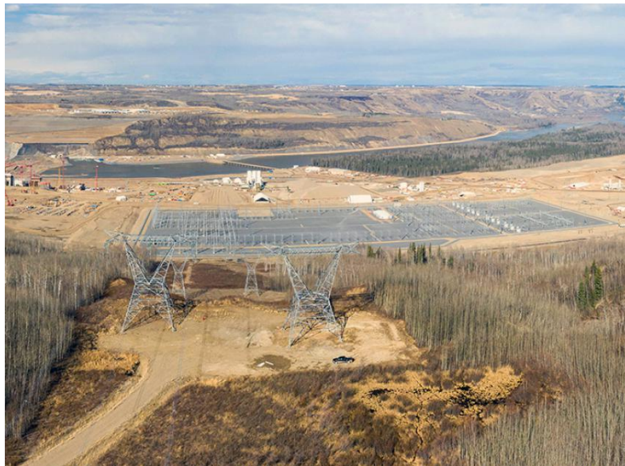
Figure A-8 Transmission towers for two new transmission lines stand side-by-side above the completed Site C substation (April 2021)
