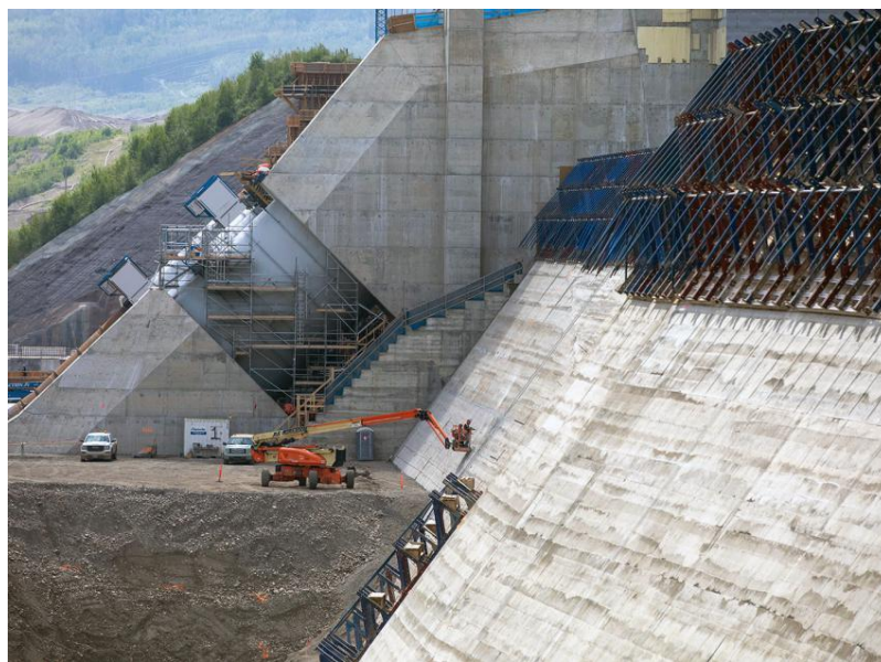
Figure A-12 Workers inspect the roller-compacted concrete at the dam and core buttress after the formwork is removed (June 2021)
