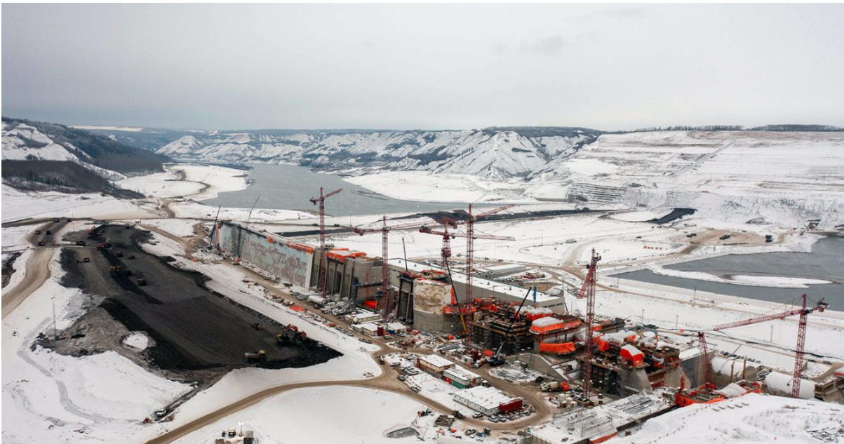
Figure A-27 A view of the dam construction site with the approach channel pictured on the left (December 2021)
