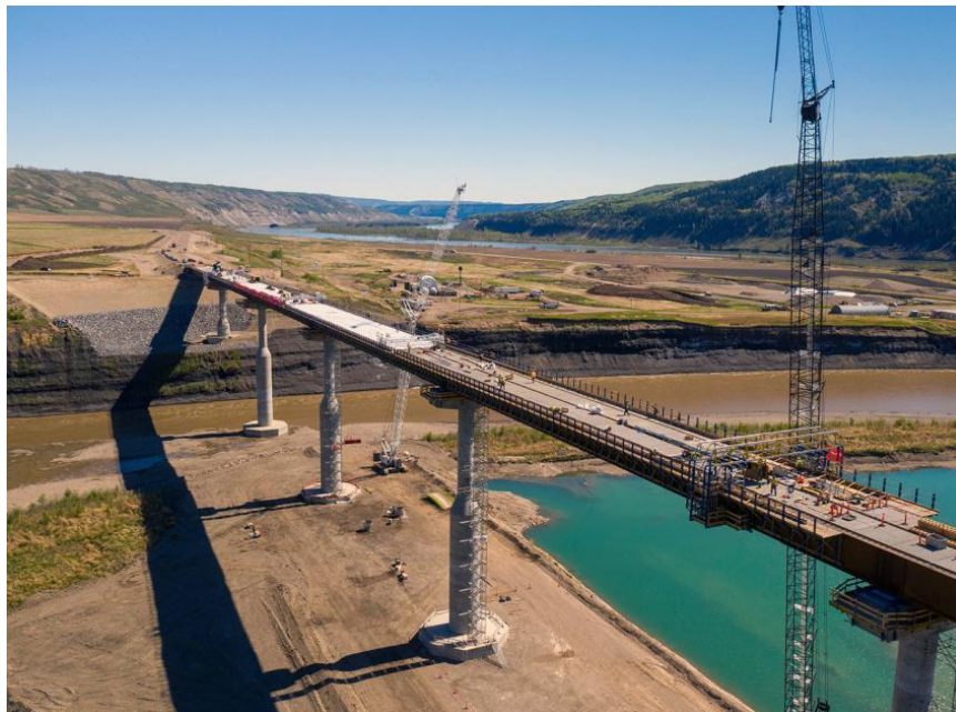
Figure A-10 Halfway River bridge showing cast-in-place bridge deck construction. The new bridge is over one kilometre long (May 2021)
