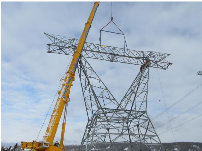
Figure A-6 The last of 205 transmission towers on the second transmission line was completed at the end of March – eight months ahead of schedule (March 2021)
