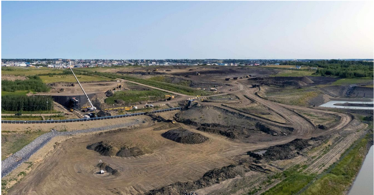
Figure A-19 Glacial till is extracted at the 85 th Ave. Industrial Lands and sent by conveyor belt to the dam site (August 2021)
