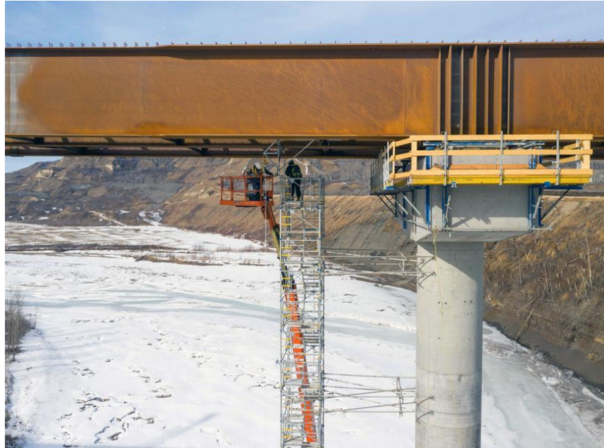
Figure A-5 Girder installation is complete, and workers remove scaffolding from the Halfway River bridge (March 2021)
