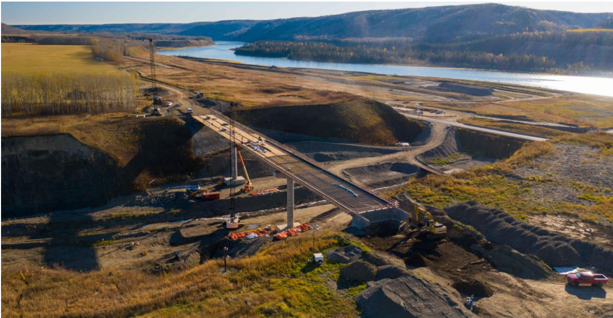
Figure A-22 Dry Creek bridge alignment on Highway 29 showing the formwork and rebar for the first concrete deck placement (Fall 2021)
