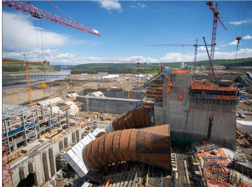
Figure A-11 An aerial view of the installation underway on the Unit 5 intake transition penstock section (May 2021)
