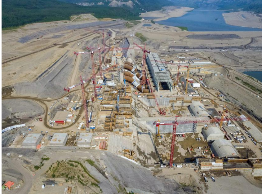
Figure A-13 An upstream view of the approach channel at top left and the powerhouse, generating station, and spillways at centre (June 2021)
