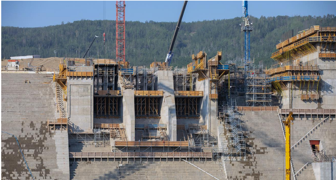
Figure A-17 Construction progresses at the spillways headworks east low-level outlet gate. The spillways will allow the passage of large volumes of water from the reservoir into the river channel downstream (July 2021)
