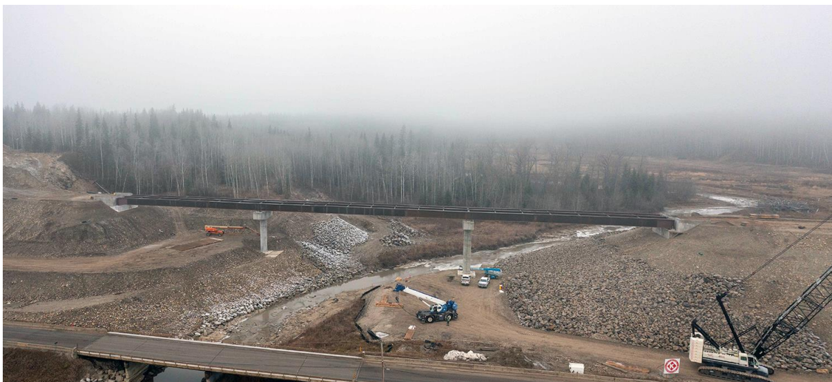
Figure A-24 Steel girder installation is complete on the Lynx Creek bridge (November 2021)
