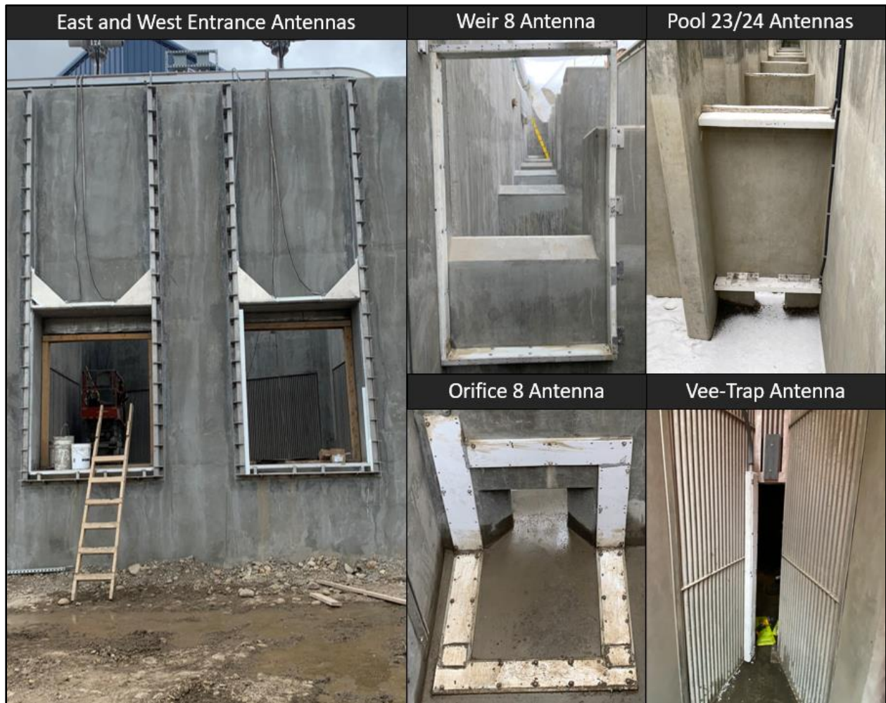
Figure 8 Photos of completed PIT antennas installed within the dewatered temporary upstream fish passage facility prior to operations.
