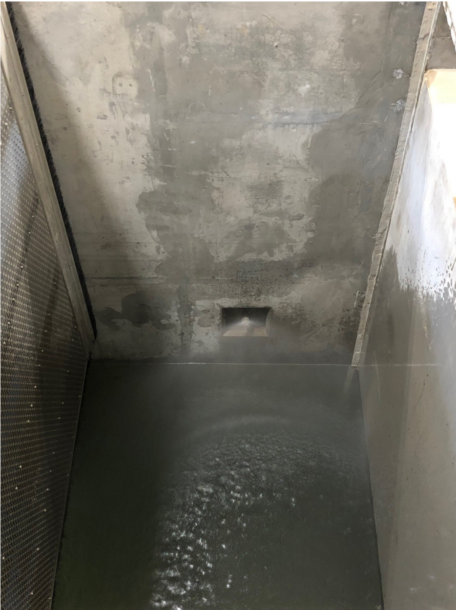
Photo 5. Sprayers located at the upstream end of the pre-sort holding pool (August 16, 2021).
