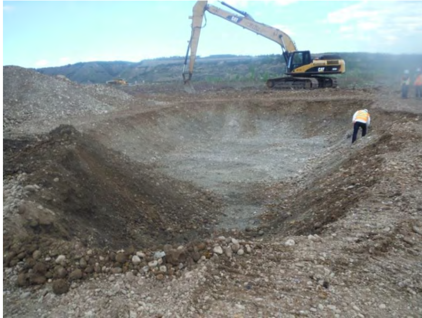
Figure A-22 Peace River Hydro Partners Digging Test Pits in the Generating Station and Spillways Area (May 2016)
