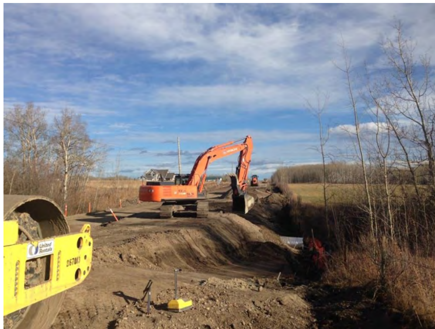
Figure A-15 Ministry of Transportation and Infrastructure Contractor A.L. Sims and Sons Prepares 240 Road for Paving (November 2015)
