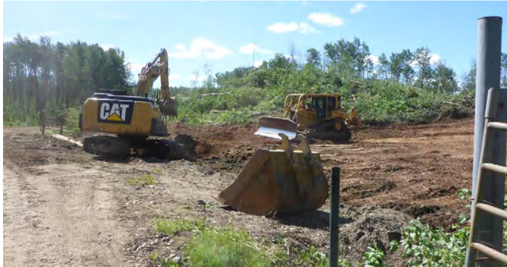
Figure A-1 Construction of the Site C Project Started July 2015 with Site Preparation Activities
