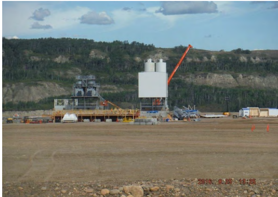
Figure A-25 Roller-Compacted Concrete Batch Plant (August 2016)
