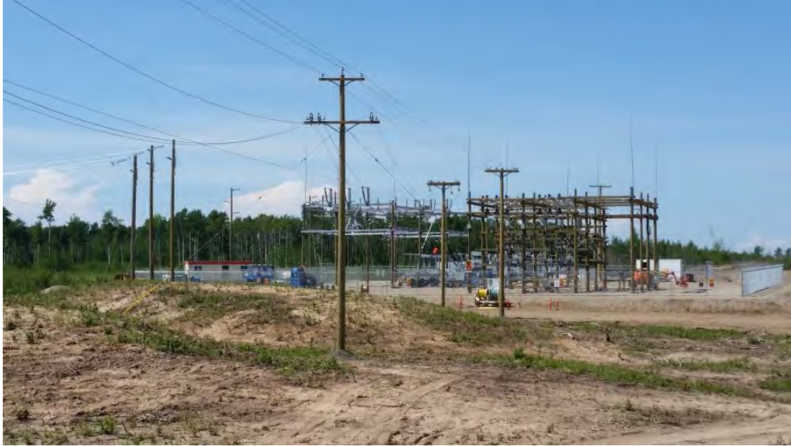
Figure A-20 Completed Site C Temporary Substation (July 2016)
