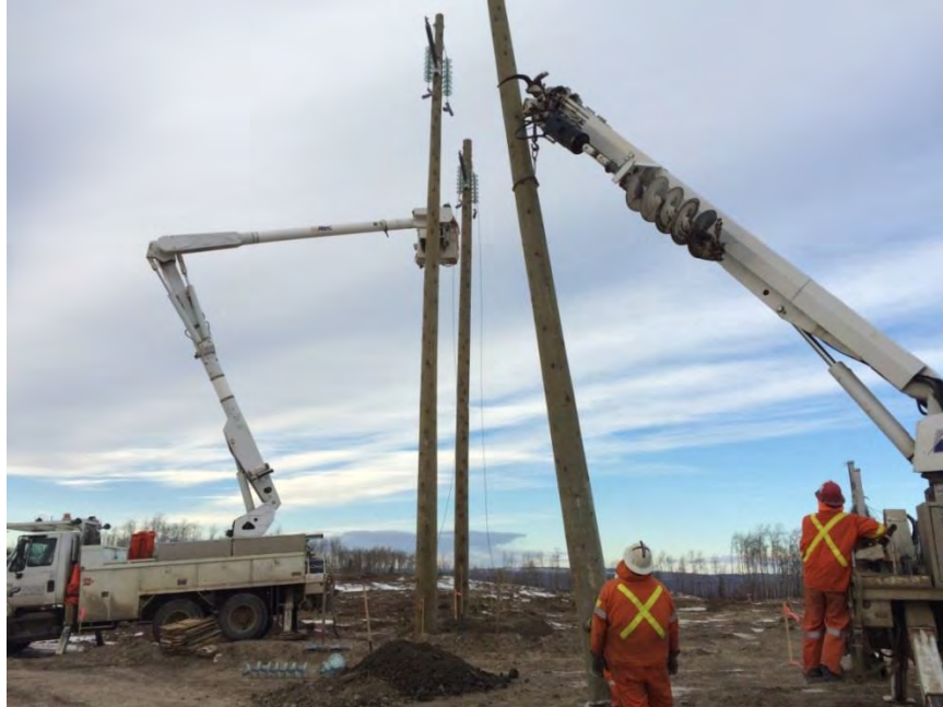
Figure A-18 Raising of 138 Kilovolt Transmission Poles for Septimus Road Crossing (November 2015)
