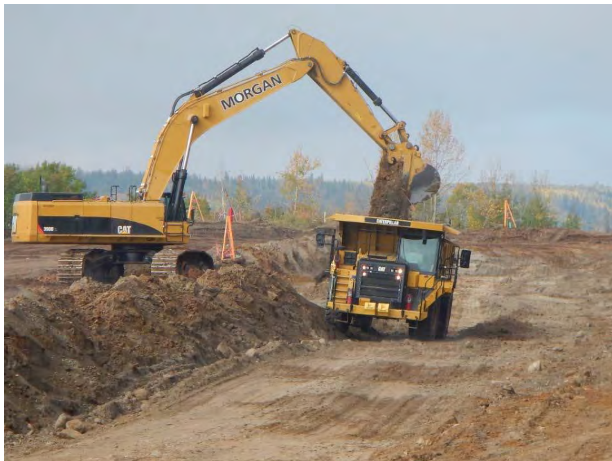
Figure A-4 Excavation of Material, Part of the North Bank Stabilization of the Site C Dam Site (September 2015)
