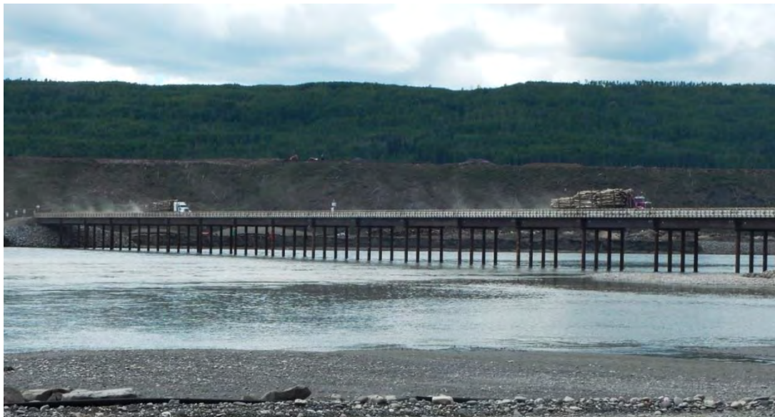
Figure A-11 Logging Trucks Hauling Timber from the Dam Site on Temporary Construction Access Bridge (May 2016)
