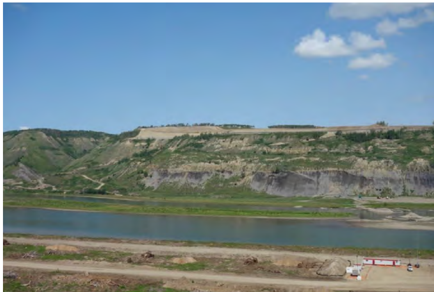
Figure A-6 North Bank Excavation viewed from South Bank. The Main Civil Works Component of the North Bank Excavation Commenced June 2016
