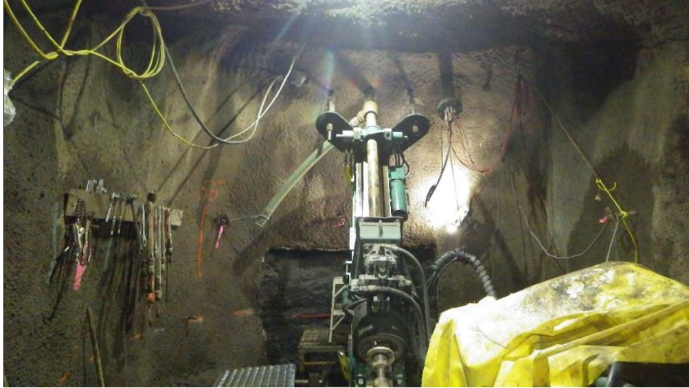
Figure A-26 In Progress Drilling for Instrumentation of Right Bank Adit 5 (August 2016)
