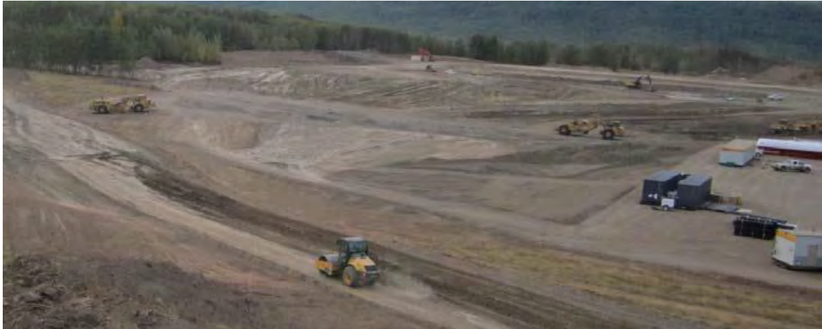
Figure A-9 Working on Access Roads and Site Preparation for the Worker Accommodation Lodge (August 2015)
