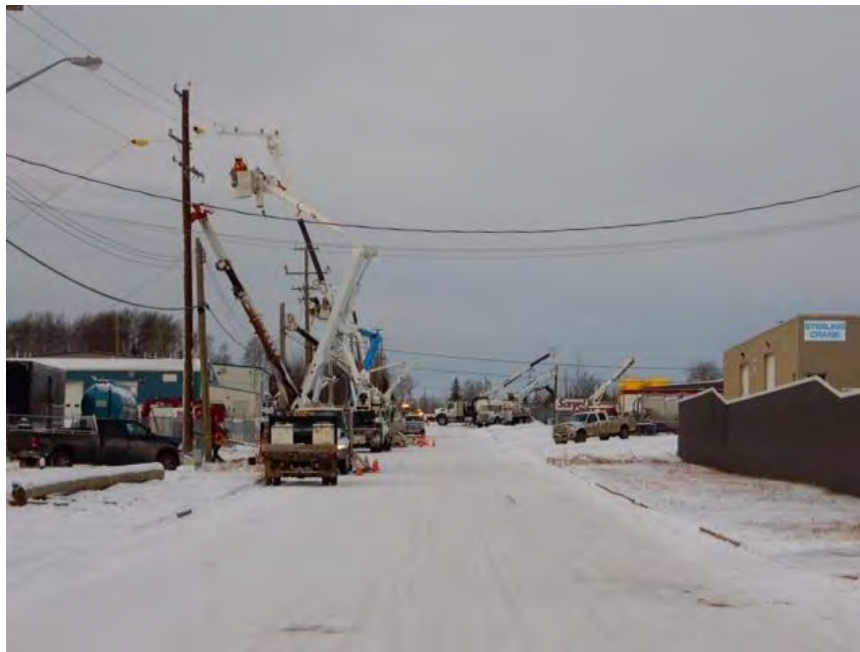
Figure A-17 Construction of Site C North Bank Distribution Line by Arctic Arrow (December 2015)
