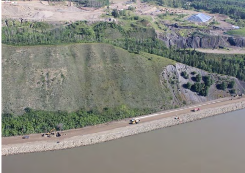
Figure A-14 Aerial View of North Bank of Dam Site Showing River Road Riprap Placement (July 2016)
