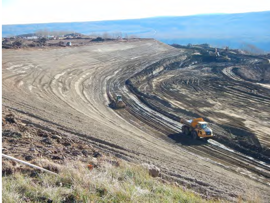
Figure A-5 North bank stabilization of the Site C Dam Site (October 2015)
