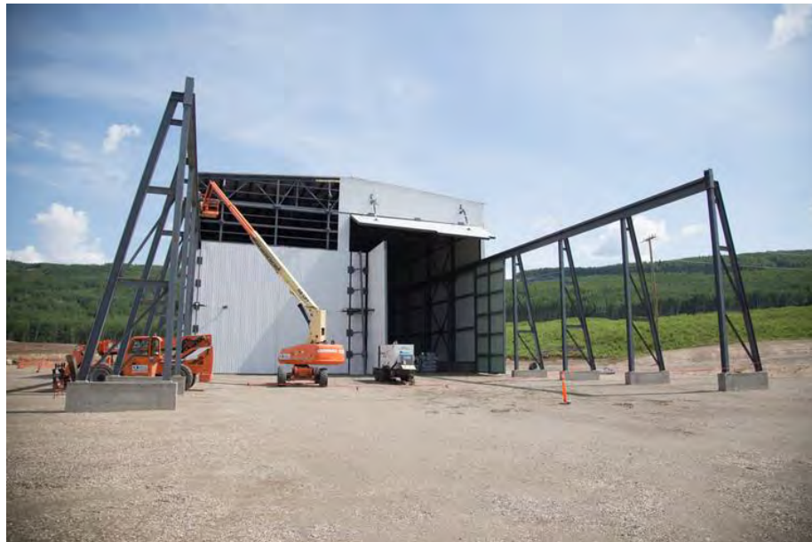
Figure A-18 Exterior View of the Temporary On-site Manufacturing Facility for the Turbines and Generators (June 2017)
