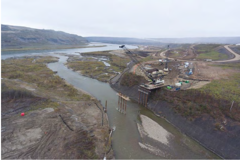
Figure A-1 Construction of the Moberly River Construction Bridge, Looking Northeast. (October 2016)
