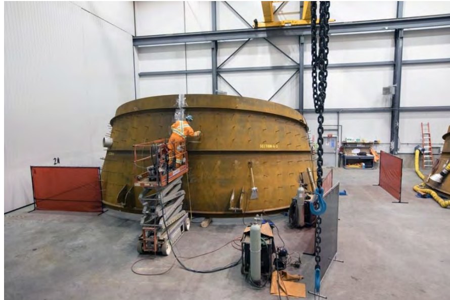
Figure A-30 Turbines and Generators Contractor Assembling Equipment at their Work Area (November 2017)
