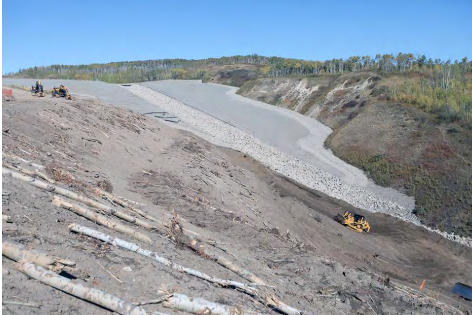
Figure A-27 Completed Upper Inclined Portion of the Closure Channel in the L3 Gully on the North Bank. (September 2017)
