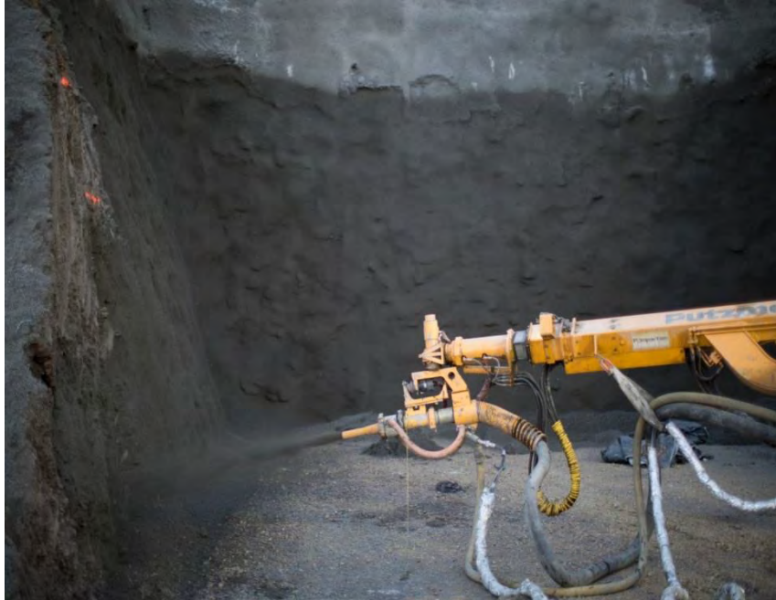
Figure A-8 Shotcrete Application at the Drainage Tunnel on the South Bank (December 2016)
