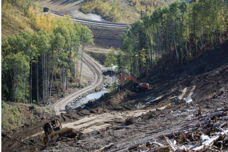
Figure A-23 Slope Stabilization above the Closure Chancel in the L3 Gully on the North Bank (September 2017)
