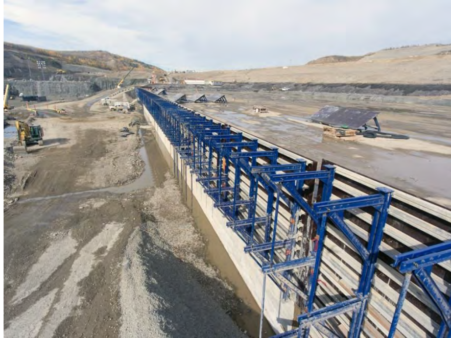
Figure A-25 Roller-compacted Concrete Placement at the Stilling Basin on the South Bank (September 2017)
