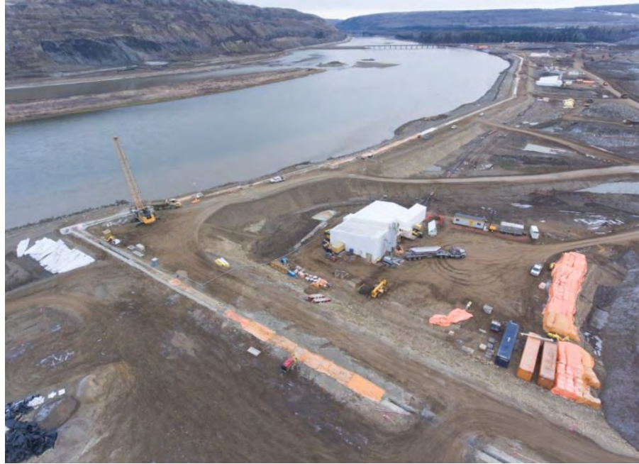
Figure A-5 Aerial View of the Stage 1 Right Bank Cofferdam, including One of Three Slurry (Concrete) Production Plants (November 2016)
