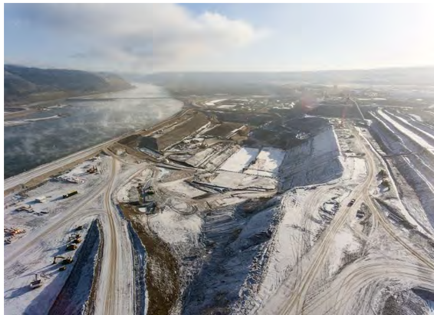
Figure A-33 Aerial View of the South Bank, with the Powerhouse and Spillway Buttress and Approach Channel Excavation (November 2017)
