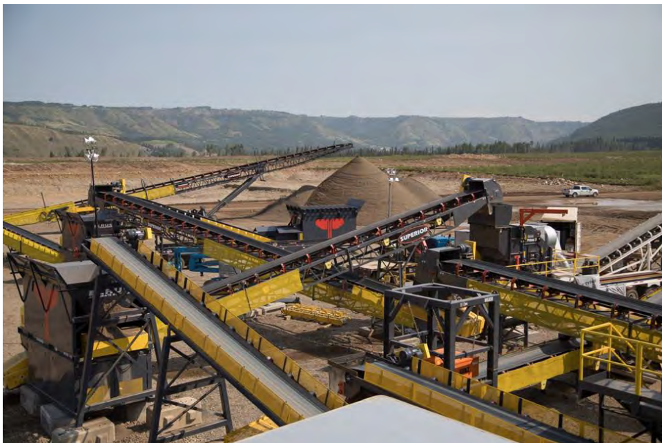
Figure A-22 Aggregate Crushing Facility on the South Bank (July 2017)
