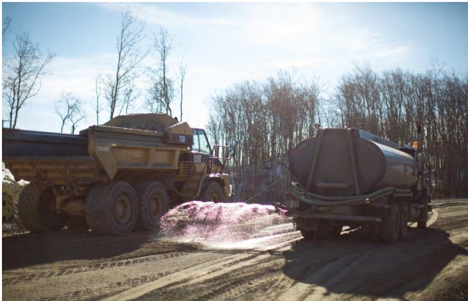
Figure A-2 Dust Mitigation on the North Bank View Point Access Road (October 2016)
