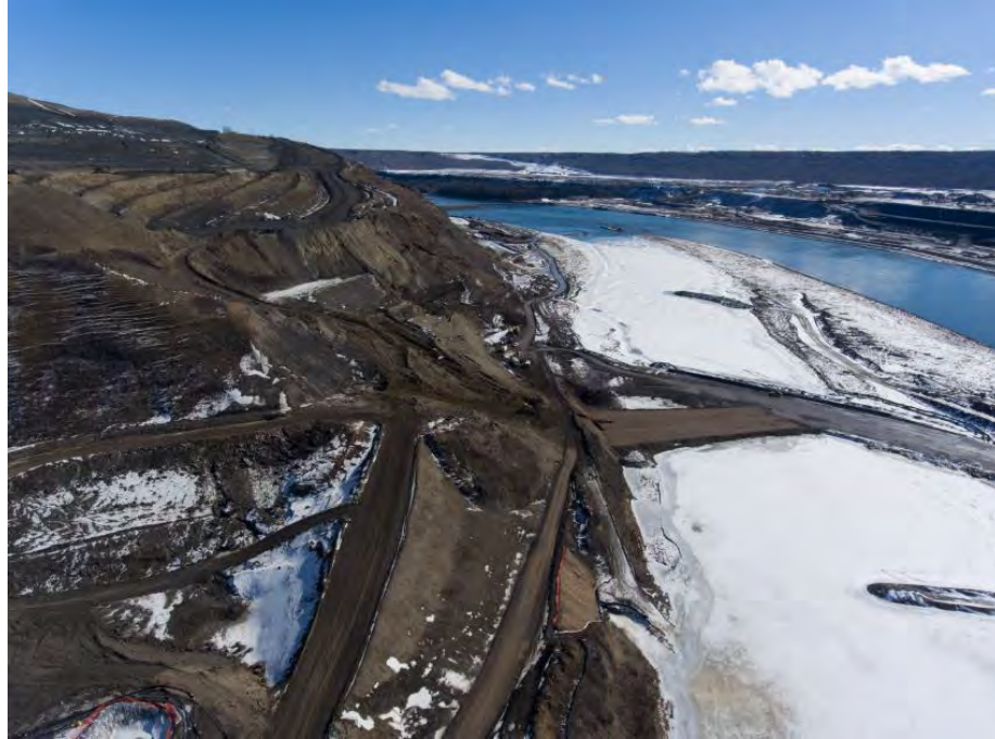
Figure A-11 Aerial View of Remediation for the Tension Crack on the North Bank (March 2017)
