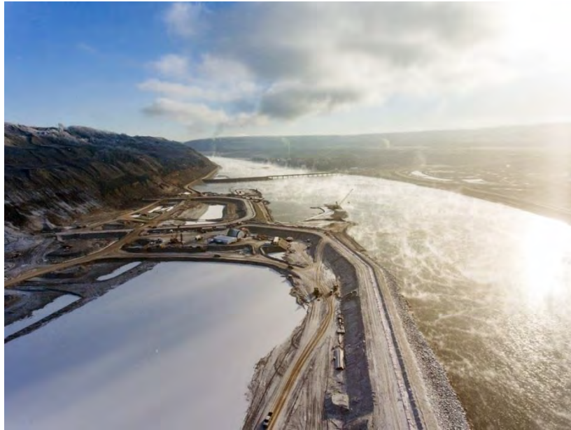
Figure A-32 Aerial View of the North Bank, with Cofferdams and Laydown Area, Looking East (November 2017)
