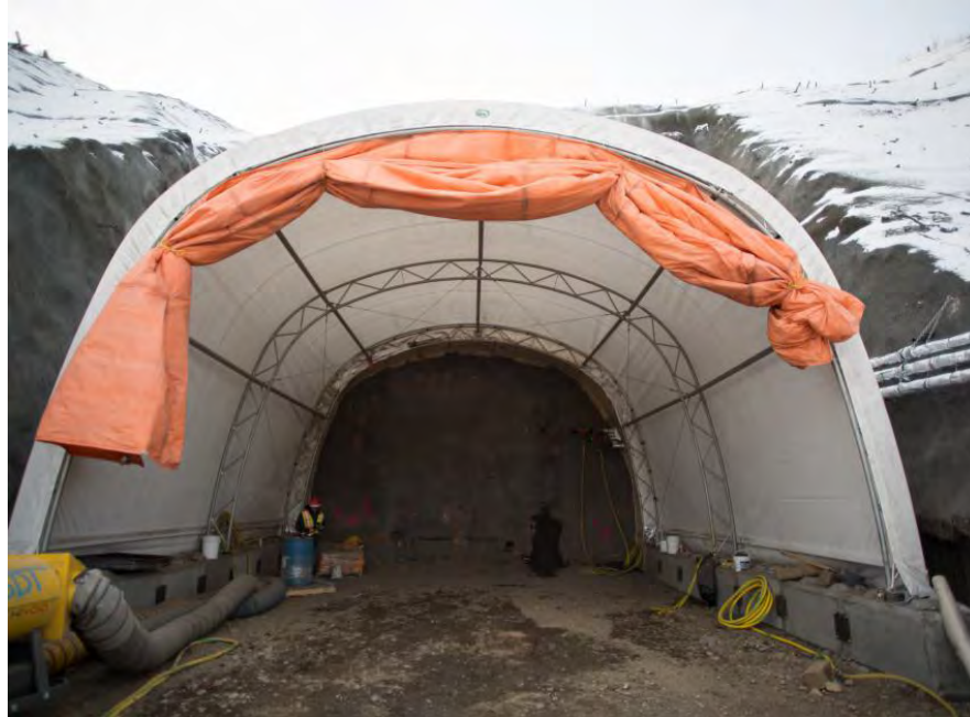
Figure A-10 Preparation for the Start of Tunnelling at the Drainage Tunnel on the South Bank (January 2017)
