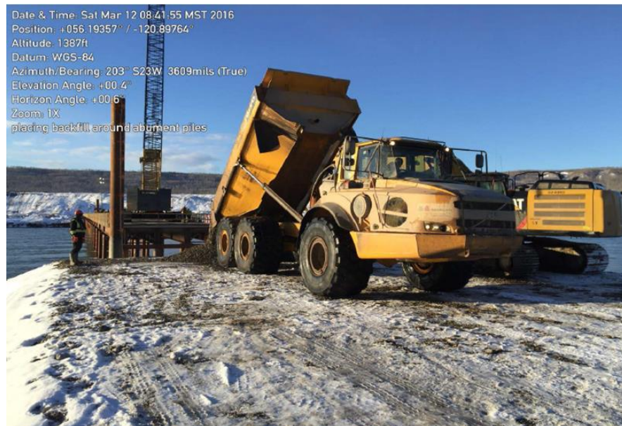
Figure A2 Contractor Backfilling the Approach to the Peace River Construction Bridge
