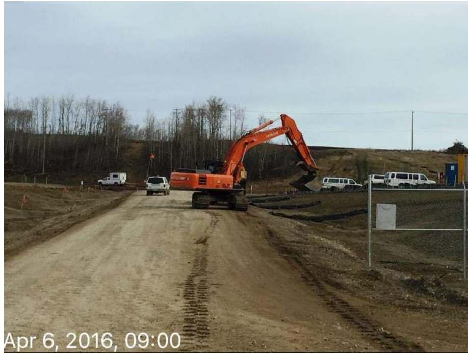
Figure A3 Maintenance of Erosion and Sediment Control along Storm Ditch West of Worker Accommodation Camp
