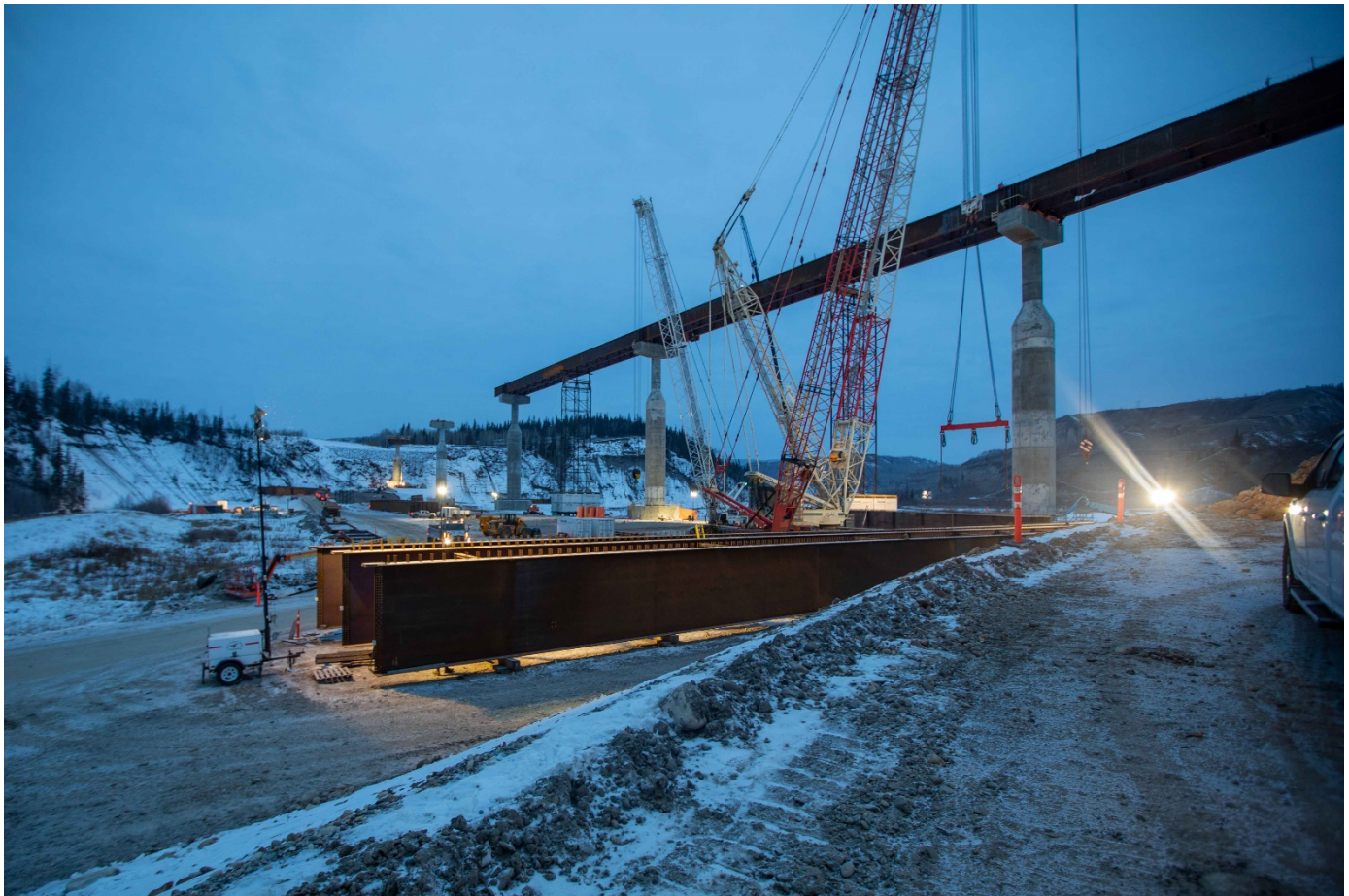
The first girders are placed on the Cache Creek bridge along Highway 29. See more project photos in the image gallery .
