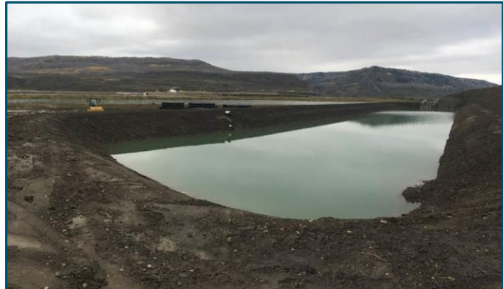
Above: Sediment pond at the Site C dam site. Sediment ponds are a best practice in sediment control. During a rain event, these ponds capture runoff that may contain eroded soil. The pond allows the sediment to drop to the bottom and keeps the water exiting the pond clean.
