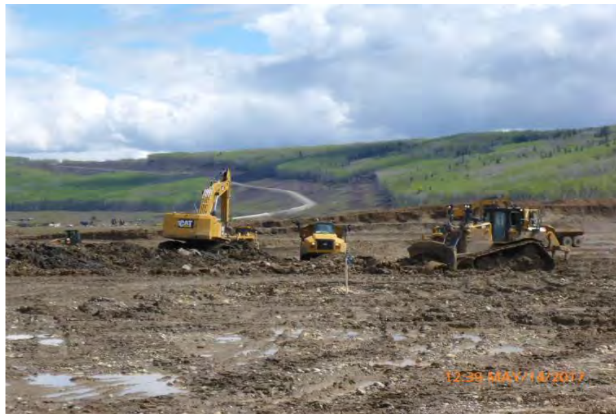
Figure A-2 Substation – Excavating Saturated Clay Material from within the Transmission Line Right of Way. Photo taken May 14, 2017.
