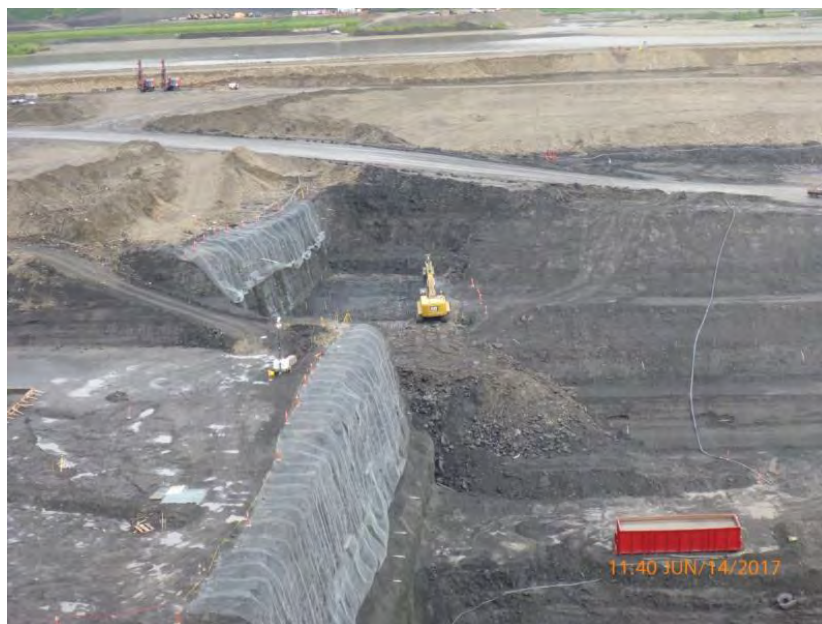
Figure A-8 Roller-Compacted Concrete Buttress – Excavator Cleaning Floor on Elevation 385 Pad. Photo taken June 14, 2017.
