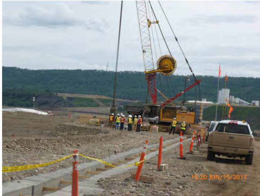
Figure A-9 Inlet Cofferdam – Contractor Excavating Test Panel Sections. Photo taken June 15, 2017.
