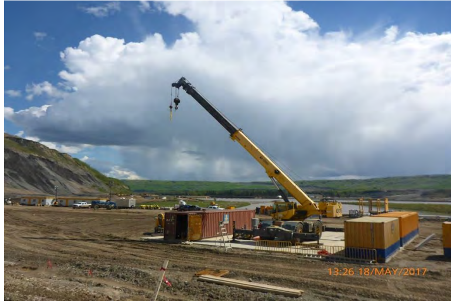
Figure A-3 Left Bank Cofferdam – Contractor beginning to set up Slurry Plant #1. Photo taken May 18, 2017.
