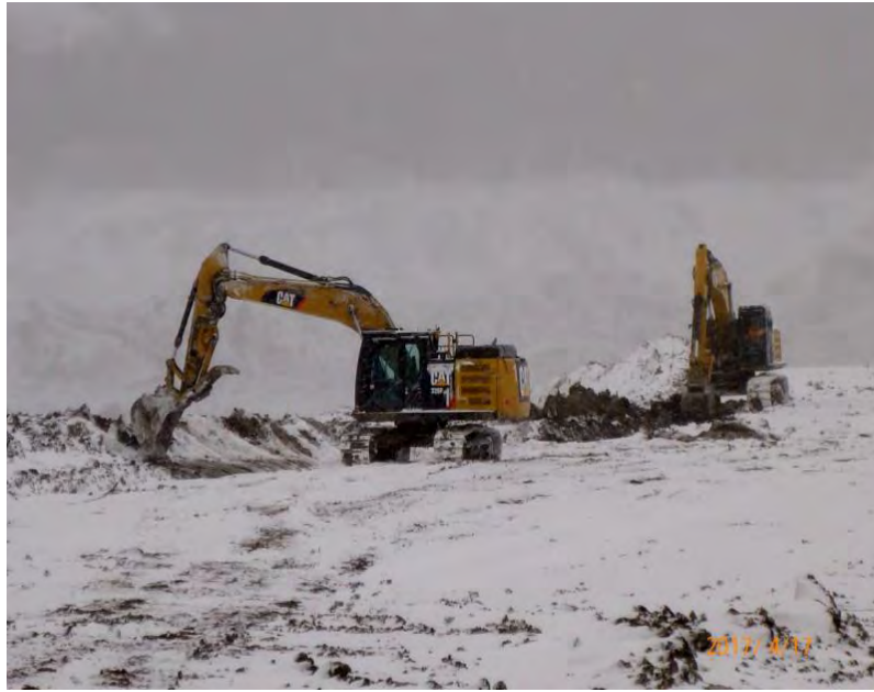
Figure A-1 Left Bank Excavation – Excavators Ditching along Outside Berm. Photo taken April 17, 2017.
