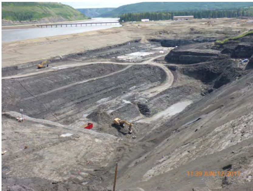
Figure A-6 Powerhouse Buttress – Excavator Working on the Detailed Excavation of Elevation 375 Bench. Photo taken June 12, 2017.
