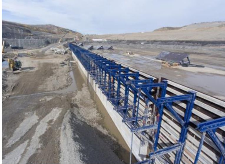
Figure A-11 Roller-Compacted Concrete Placement at the Stilling Basin on the South Bank. Photo taken September 26, 2017.
