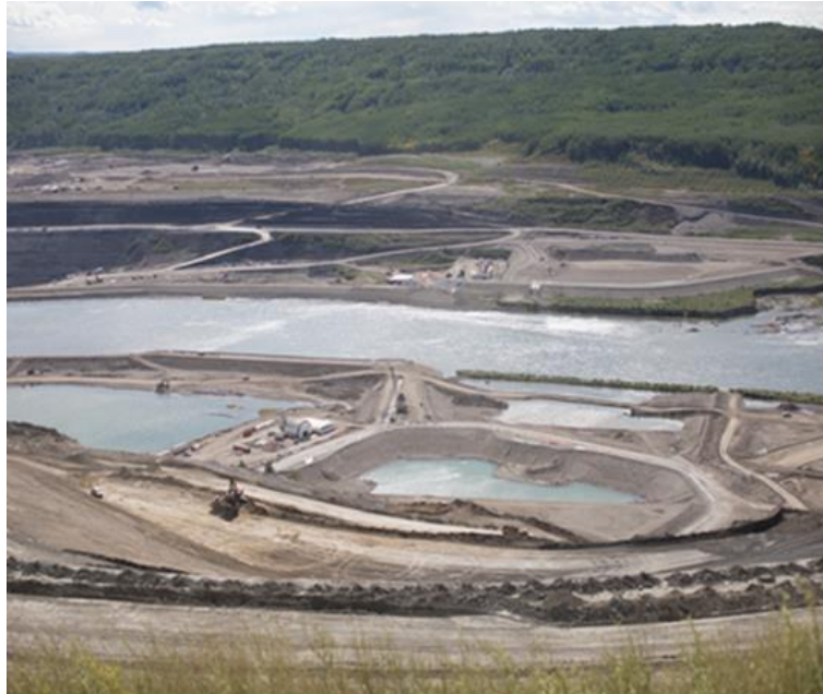
Figure A-9 Aerial View of North Bank Diversion Inlet Portal and Dam Core Areas. Photo taken August 20, 2017.
