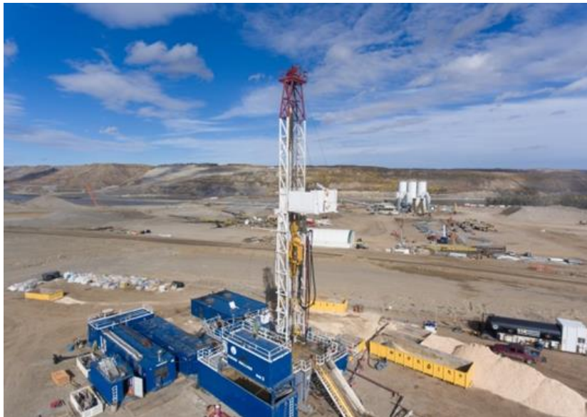
Figure A-12 Work to Decommission the Abandoned Wellbore on the South Bank. Photo taken September 26, 2017.
