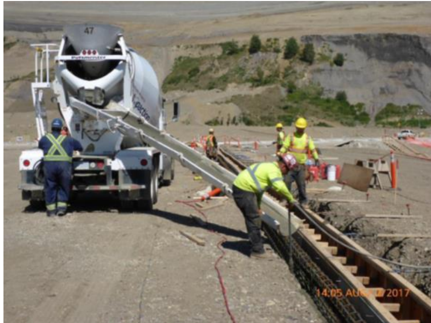
Figure A-5 Workers Installing Formwork and Rebar Cages for Slurry Guide Wall. Photo taken August 2, 2017.
