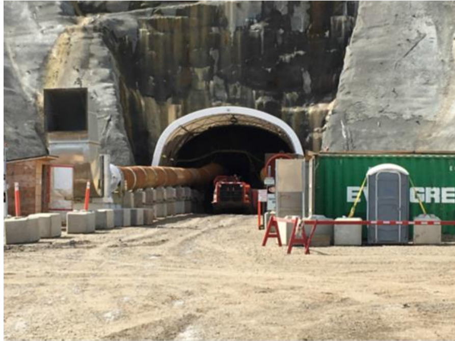
Figure A-3 Right Bank Drainage Tunnel – Silica Mitigation Production Trial Underway. Photo taken July 2017.
