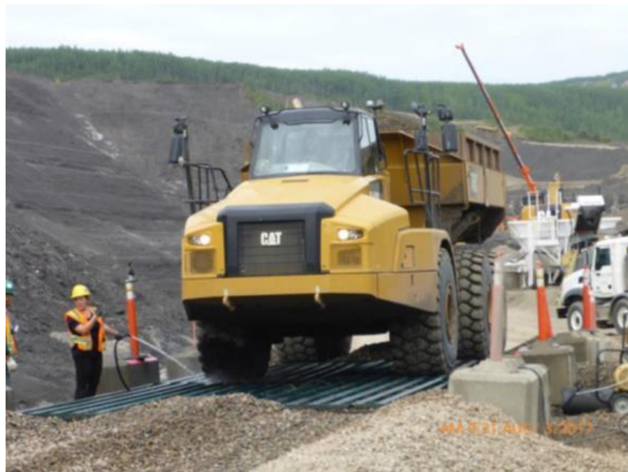
Figure A-8 Stilling Basin Temporary Wheel Wash Station. Photo taken August 3, 2017.
