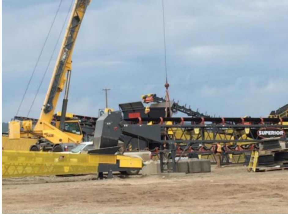
Figure A-7 Installation of Conveyors in the Crusher Plant. Photo taken August 3, 2017.
