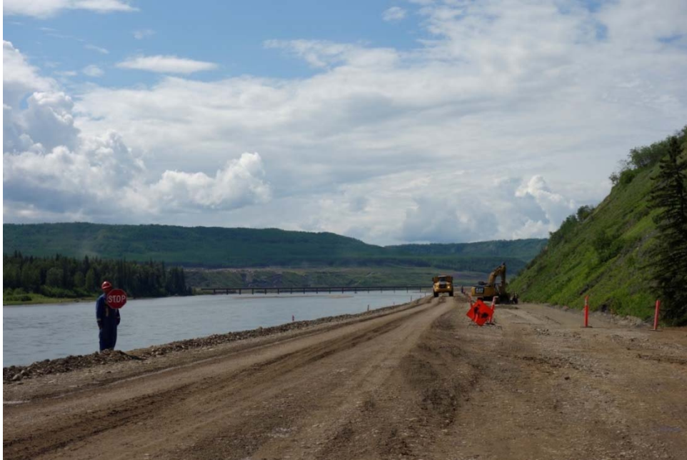
Figure A-5 Viewing westbound along River Road near Final Grade (Morgan Construction)
