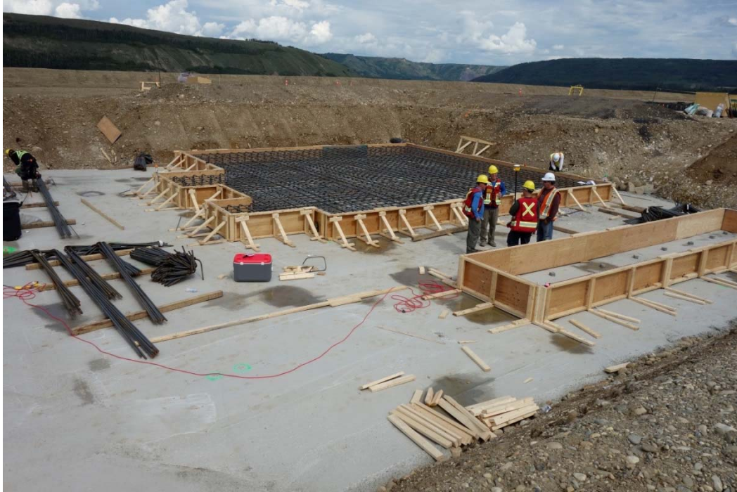
Figure A-7 Preparation of Roller-Compacted Concrete Batch Plant Foundations (Peace River Hydro Partners)
