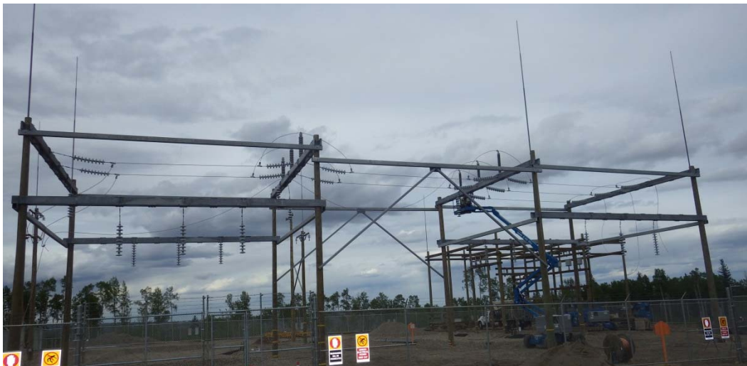
Figure A-2 Temporary Transmission Substation
