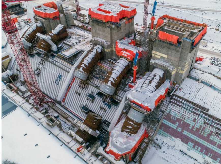
Figure A-1 An aerial view of the Site C penstocks and intakes under construction (January 2021)
