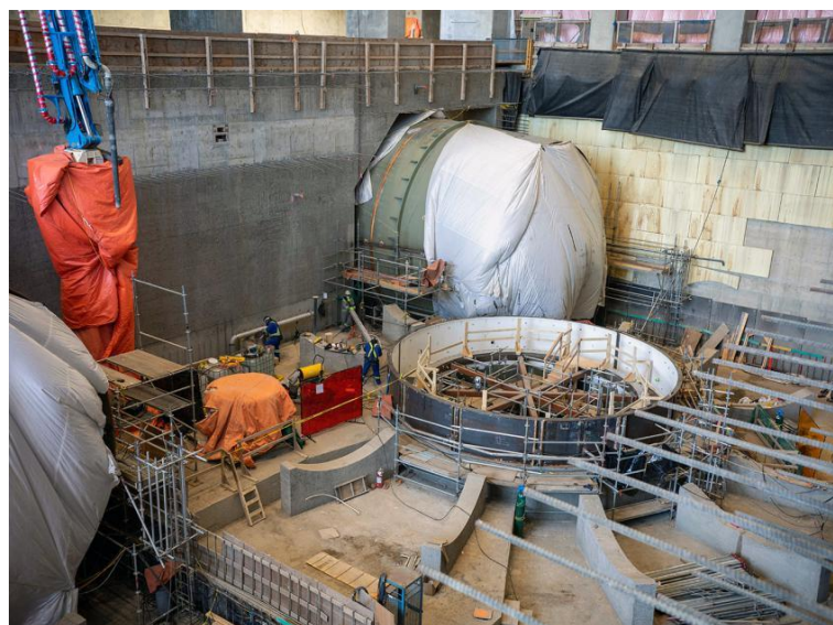
Figure A-6 Crews have commenced installation of the turbine-embedded components for Units 1 and 2 inside the powerhouse. The Unit 1 draft tube cone and thrust ring are being prepared for installation (February 2021)
