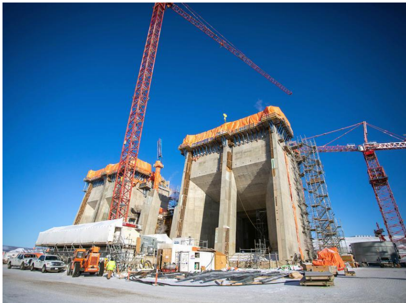
Figure A-8 Intake Units 1 and 3 are nearing completion as part of the ongoing powerhouse construction (February 2021)
