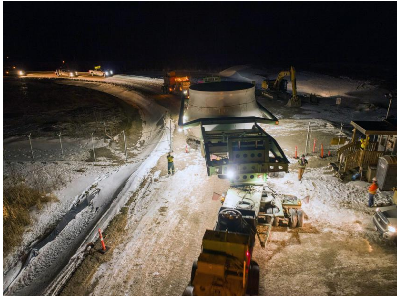
Figure A-3 Unit 1 turbine runner arrives at Site C after travelling from Sao Paulo, Brazil, by ship to Prince Rupert, and transported on a customized truck to the project site (January 2021)
