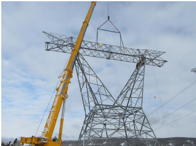
Figure A-12 The last of 205 transmission towers on the second transmission line was completed at the end of March – eight months ahead of schedule (March 2021)
