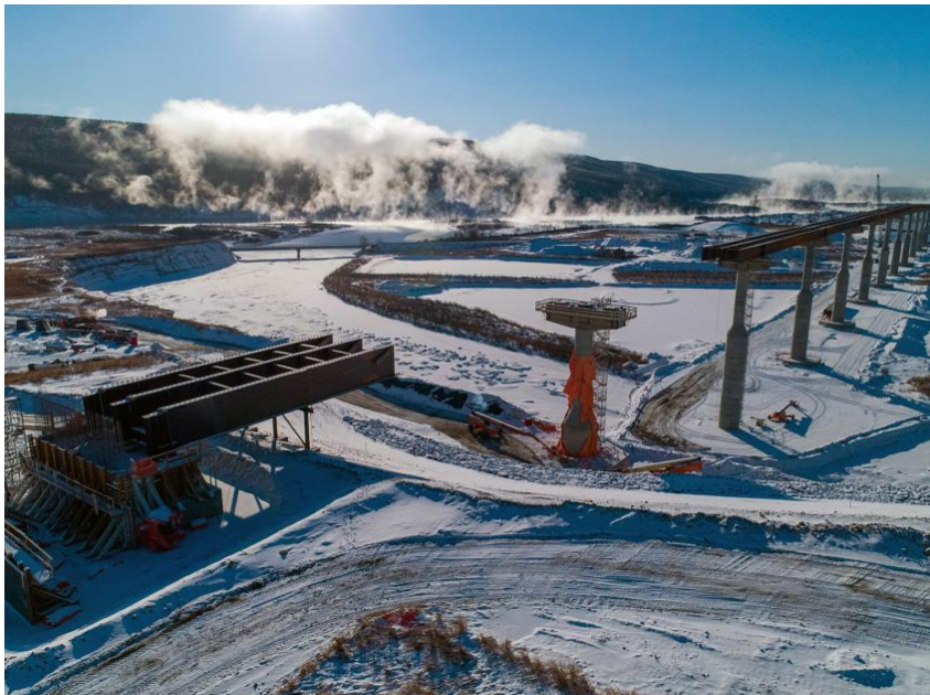
Figure A-2 Halfway River bridge construction where the final girders will connect pier 12 to the eastern bridge abutment (January 2021)
