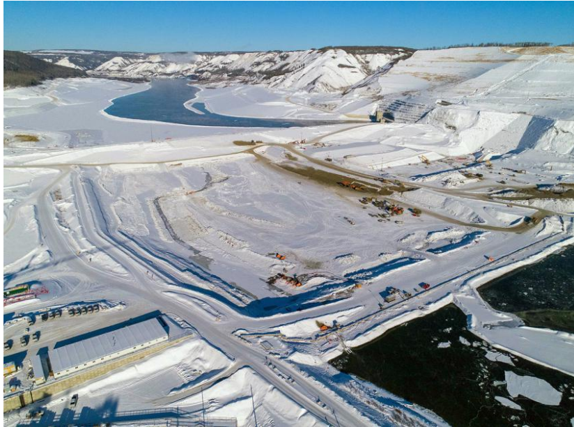
Figure A-7 The upstream and downstream cofferdams, which divert the Peace River through the two diversion tunnels (February 2021)
