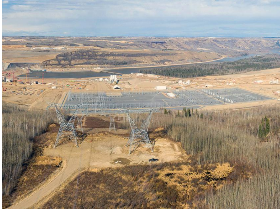
Figure A-3 Transmission towers for two new transmission lines stand side-by-side above the completed Site C substation (April 2021)
