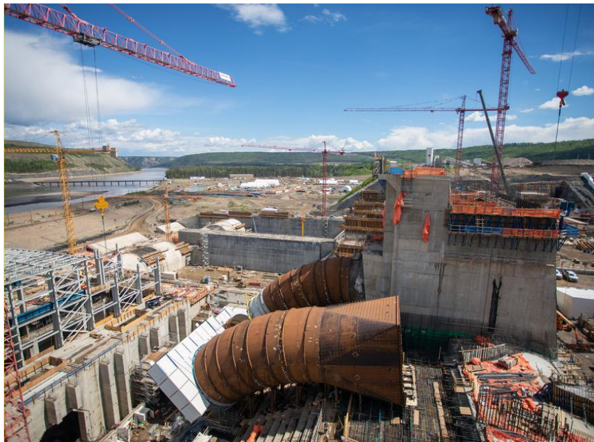
Figure A-8 An aerial view of the installation underway on the Unit 5 intake transition penstock section (May 2021)
