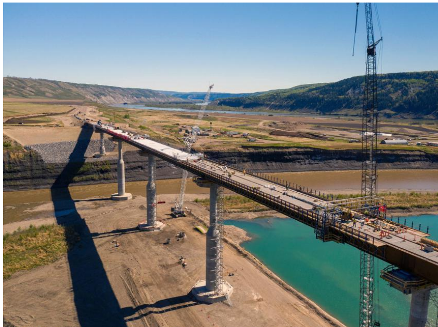
Figure A-6 Halfway River bridge showing cast-in-place bridge deck construction. The new bridge is over one kilometre long (May 2021)
