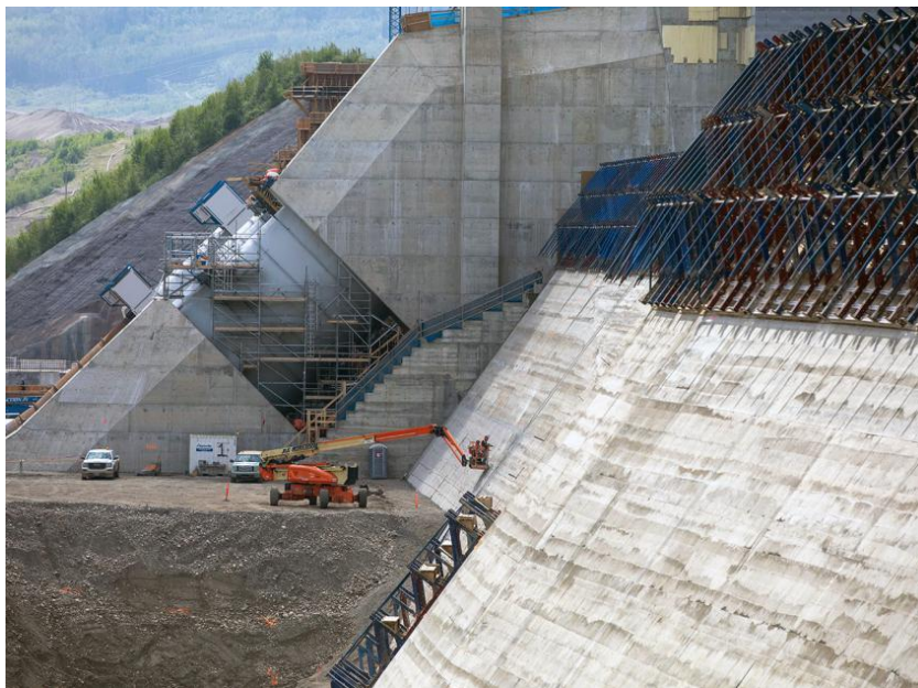
Figure A-10 Workers inspect the roller-compacted concrete at the dam and core buttress after the formwork is removed (June 2021)
