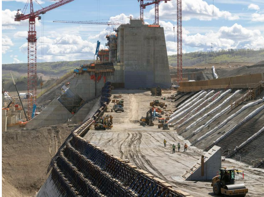
Figure A-5 Crews place roller-compacted concrete on the dam and core buttress (May 2021)
