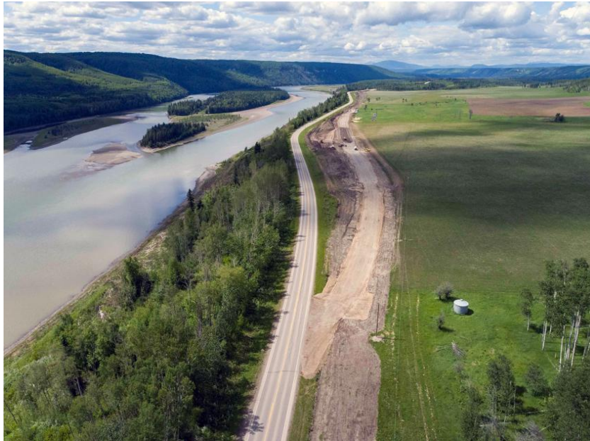
Figure A-9 Highway 29 construction at Farrell Creek east. Current activities at Farrell Creek include construction of a 411-metre-long bridge and 1.9 kilometres of highway realignment (June 2021)
