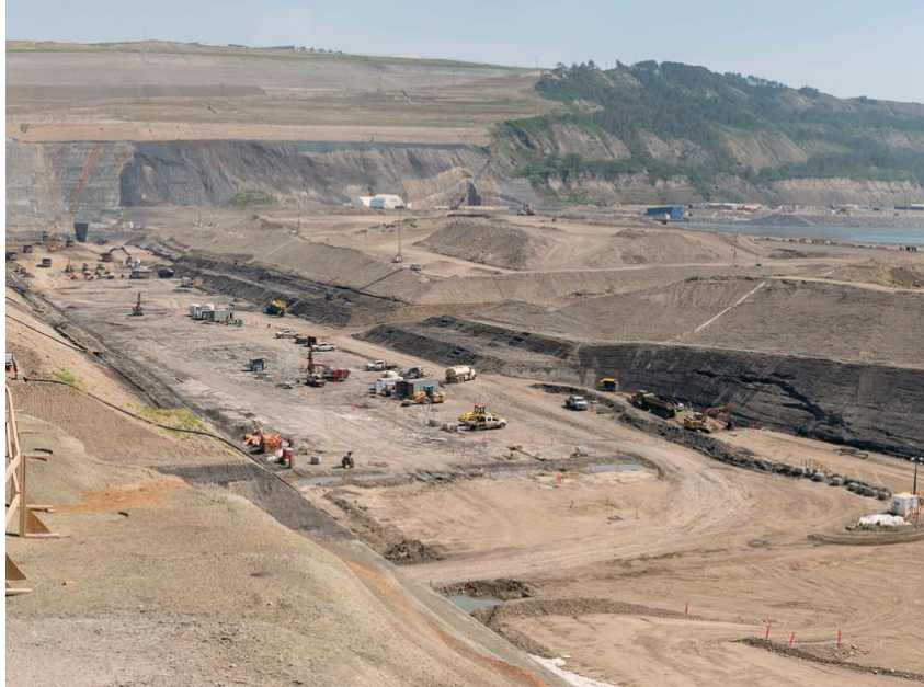
Figure A-11 The dam core trench showing the downstream shell of the dam (June 2021)
