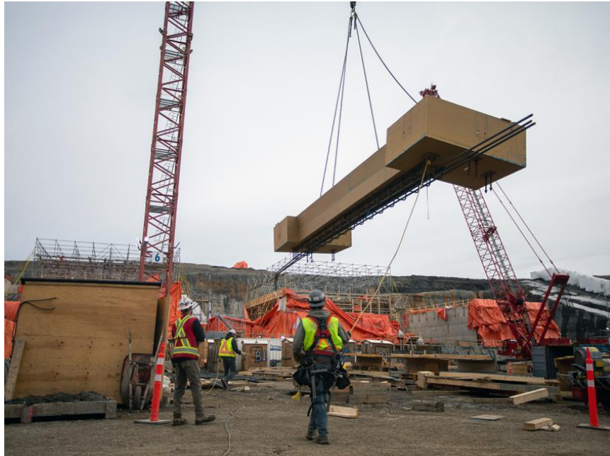
Figure A-1 Crews use a crane to lift formwork for placement at the spillway headworks (April 2021)
