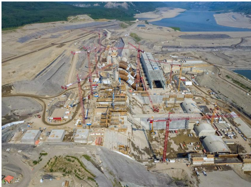
Figure A-12 An upstream view of the approach channel at top left and the powerhouse, generating station, and spillways at centre (June 2021)
