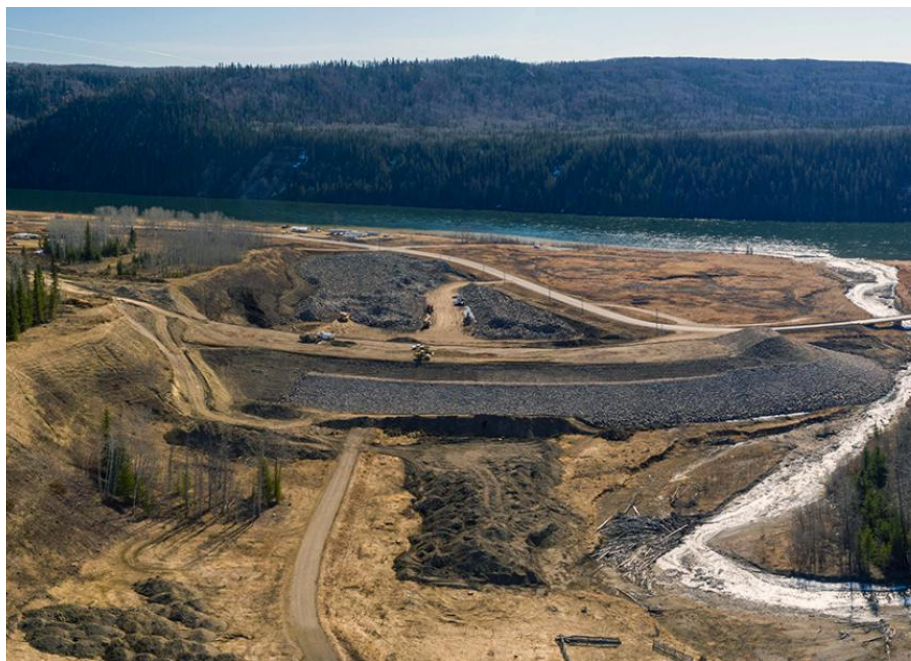
Figure A-4 Causeway construction on the Highway 29 realignment at Lynx Creek (April 2021)
