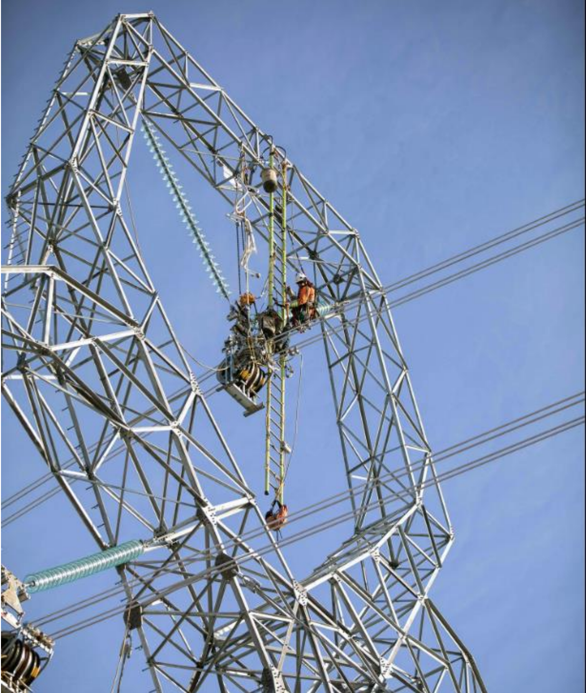
Figure A-9 Attaching the centre-phase conductor and installing corona rings on a transmission tower (February 2022)
