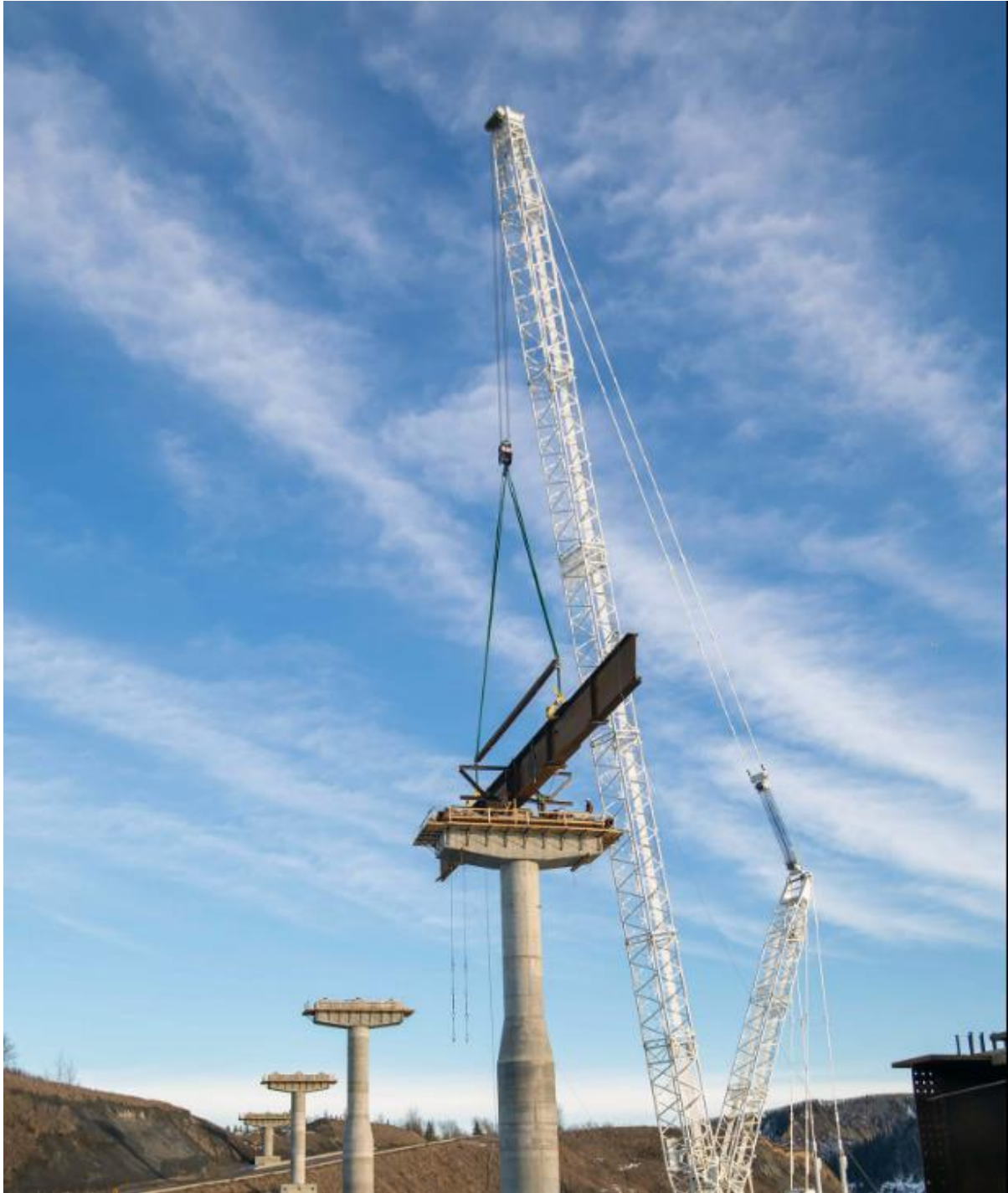
Figure A-3 The first girder is lifted onto a pier on the Farrell Creek Bridge (January 2022)
