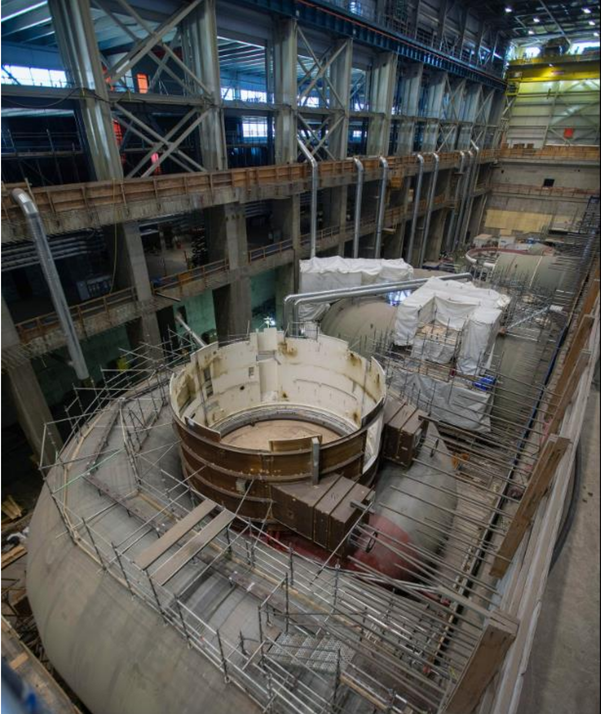
Figure A-5 Inside the powerhouse are six spiral cases at various stages of completion with this photo showing Units 4, 5, and 6 (February 2022)
