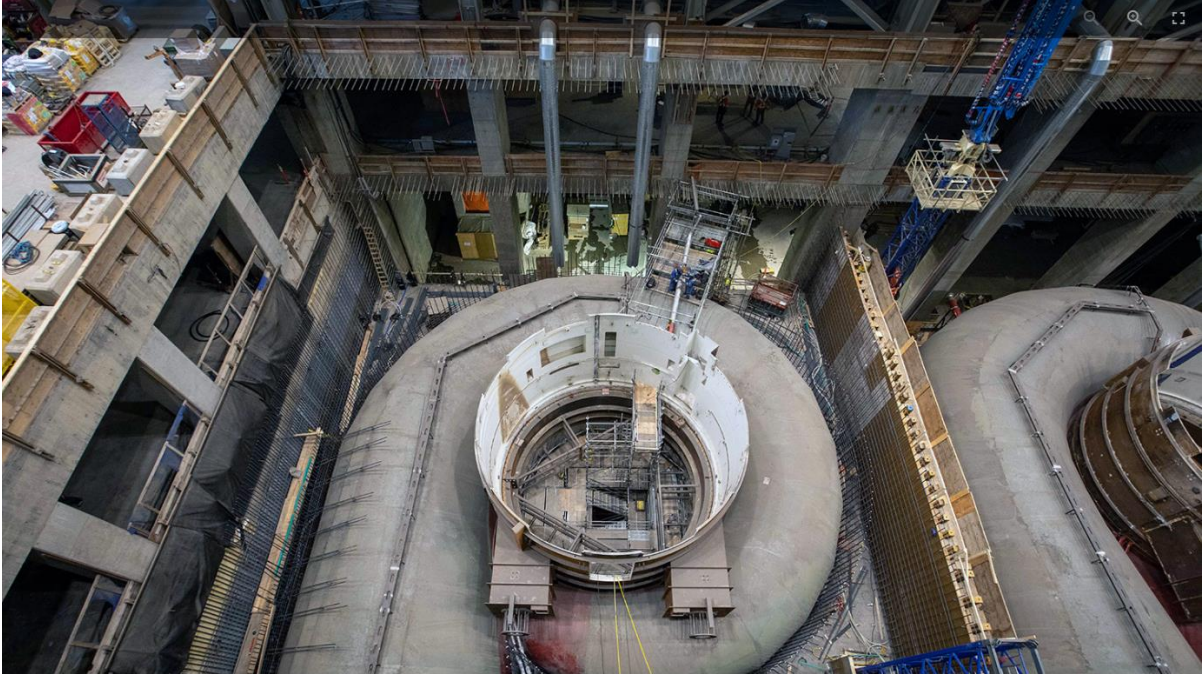
Figure A-8 Preparing embedded piping for a second lift of concrete on spiral case Unit 1 (February 2022)
