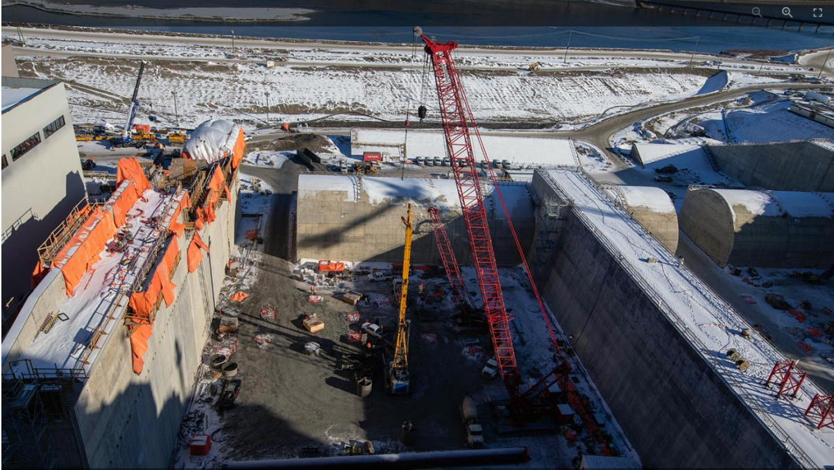
Figure A-4 Pile installation for foundation enhancement on the west spillway stilling basin (February 2022)
