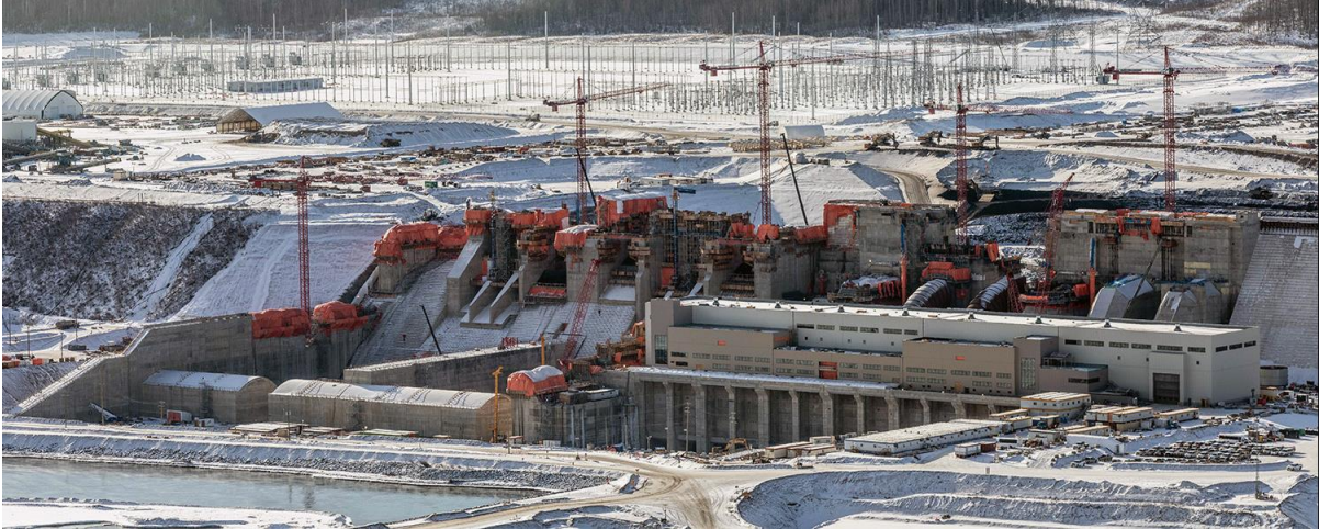
Figure A-6 A winter view of the spillways, penstocks, powerhouse, operations building and tail race (February 2022)
