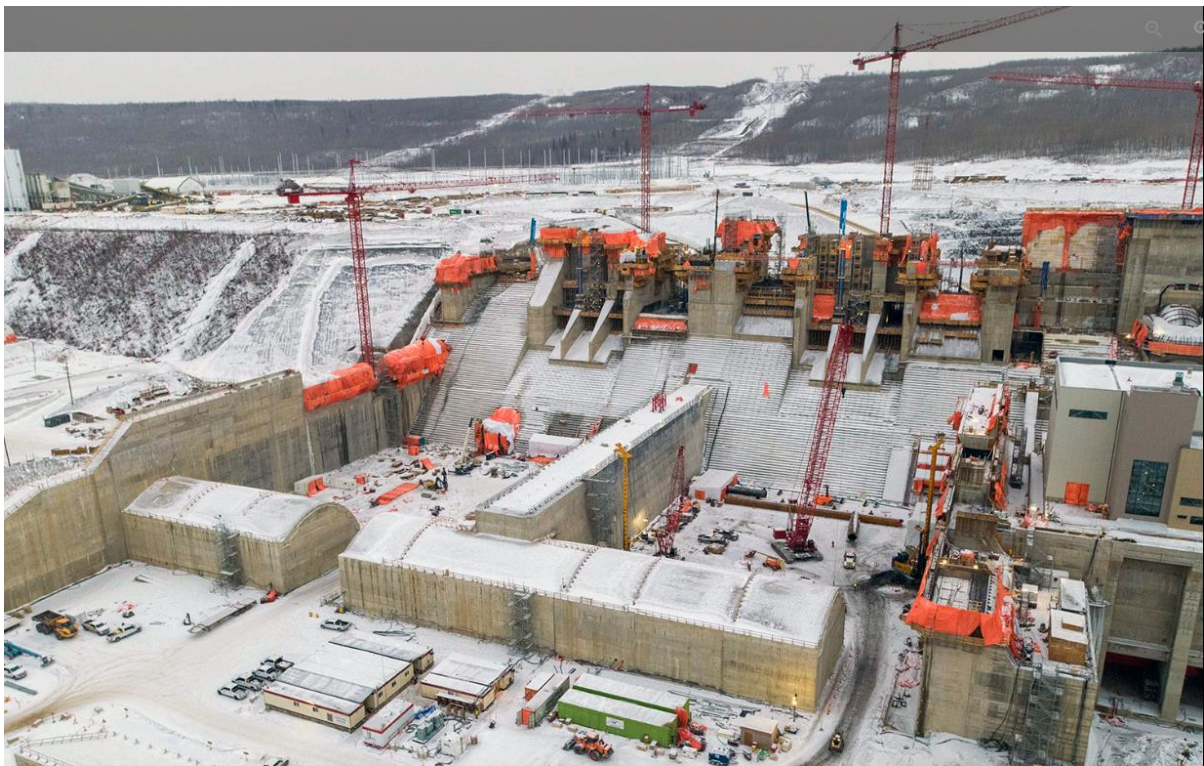
Figure A-2 Construction on the spillways including foundation enhancement work in the west bay (January 2022)
